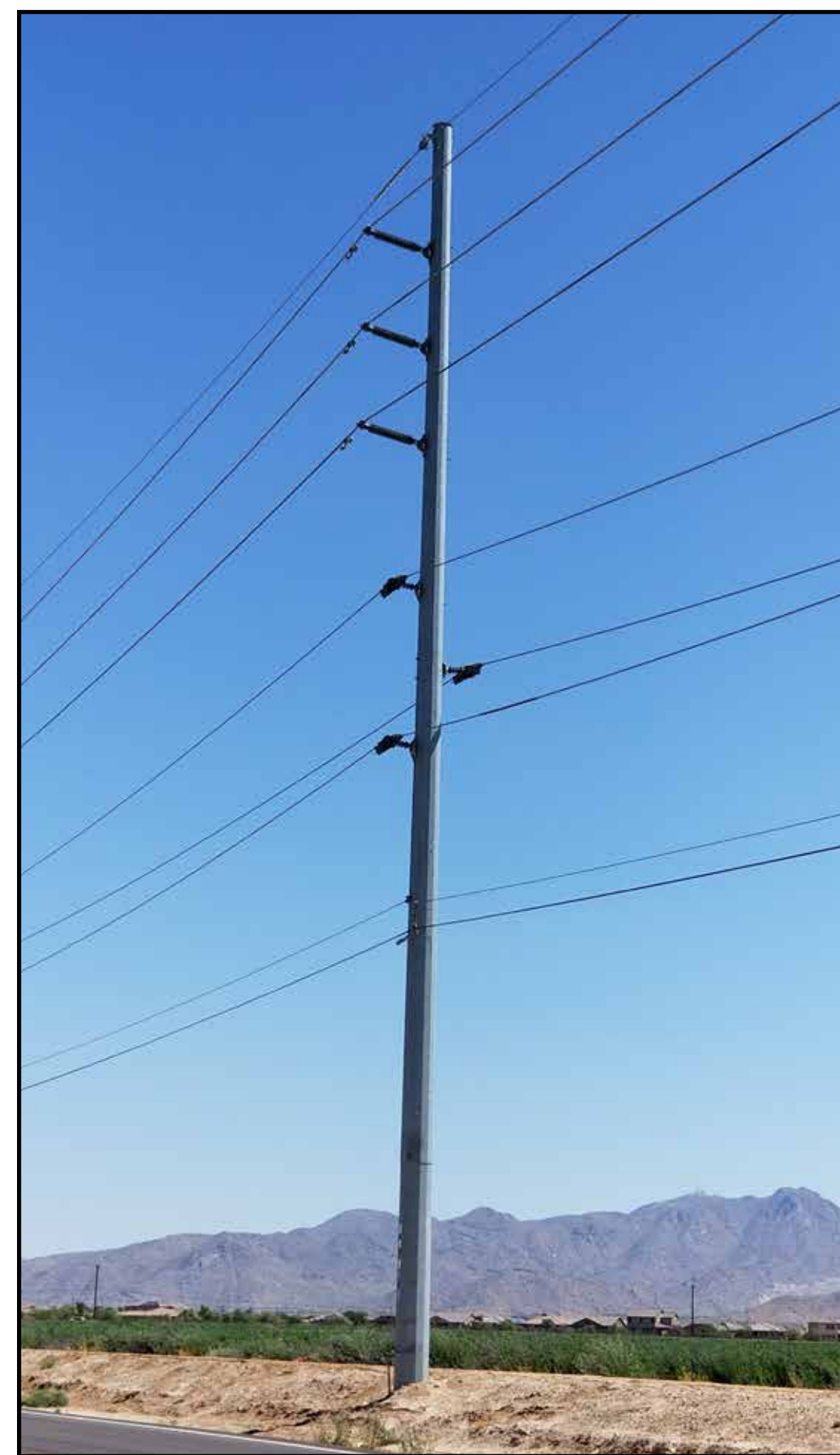
Single-circuit 69kV with 12kV under-build structure
