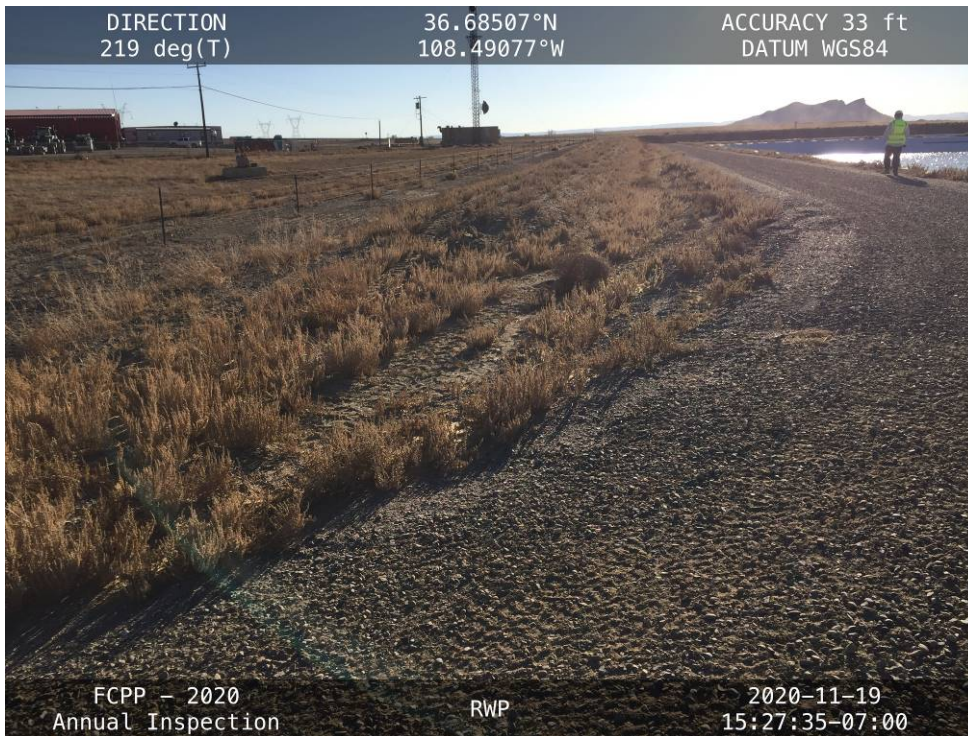
20201119 – IMG_3866 The drainage ditch along the downstream slope of the Southeast Embankment, facing southwest.
