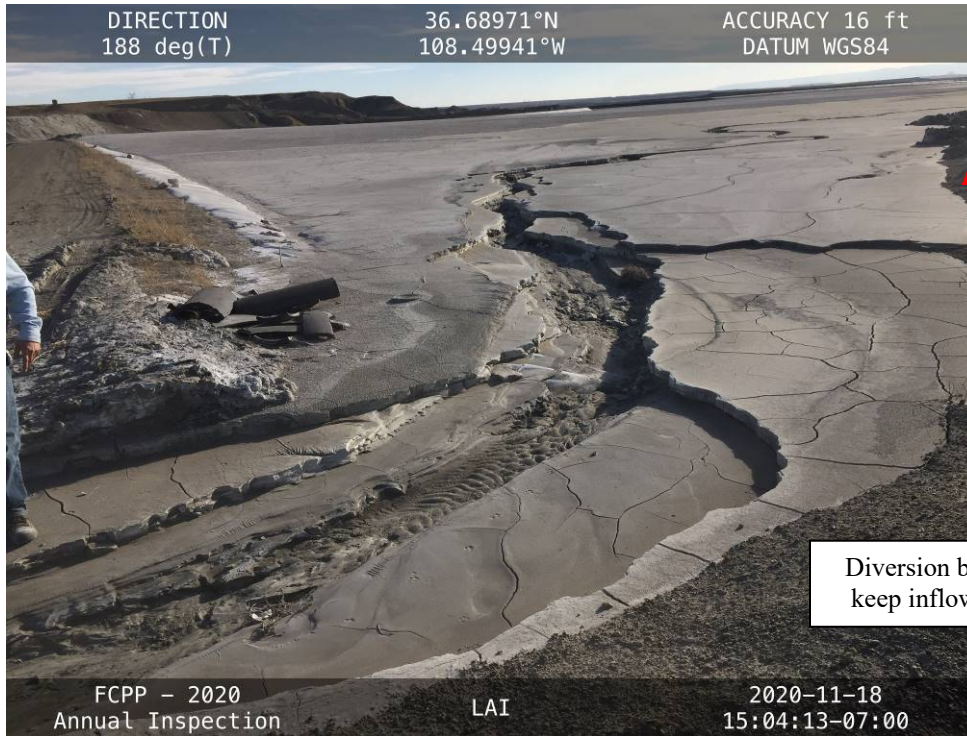
20201118 – IMG_3409 Deposition at the north V-ditch, facing south.
