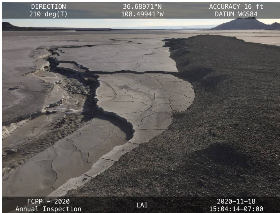
20201118 – IMG_3410 Diversion berm indicated in IMG_3409 constructed to keep inflows in the reservoir.
