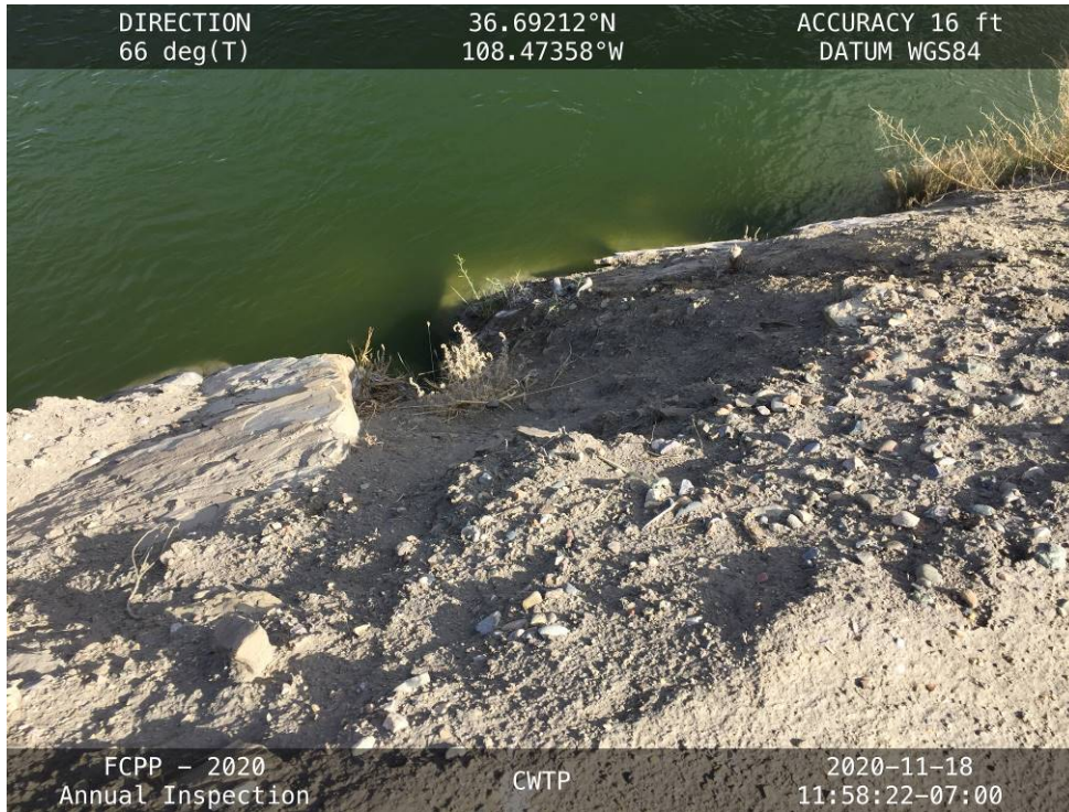
20201118 – IMG_3257 Erosion in a portion of the downstream slope without riprap.
