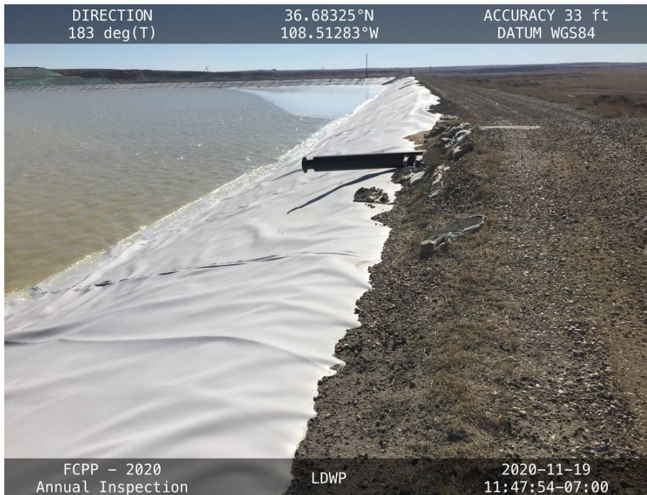
20201119 – IMG_3701 The upstream slope of the West Embankment, facing south toward the Pond 3 Pump House discharge pipe.
