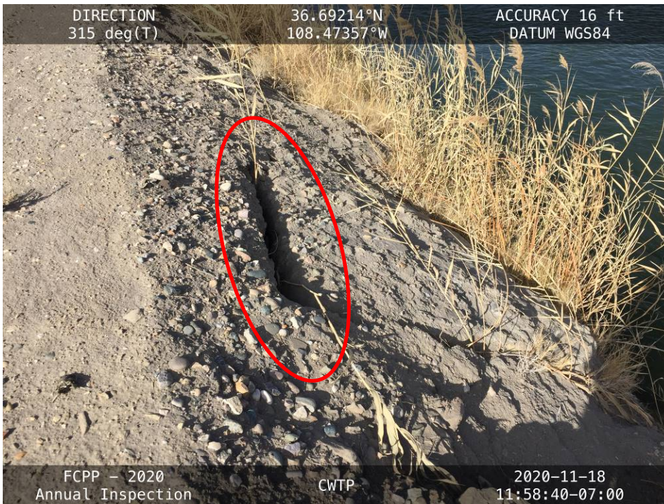
20201118 – IMG_3258 A riprap boulder separating from the rest of the slope, developing a 1-foot deep crack.
