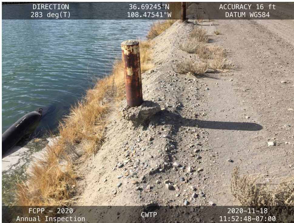
20201118 – IMG_3243 Erosion around the base of a bollard on the upstream slope.
