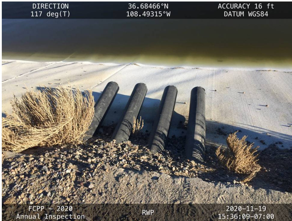
20201119 – IMG_3890 The FGD Pond cell Inlet Pipes.
