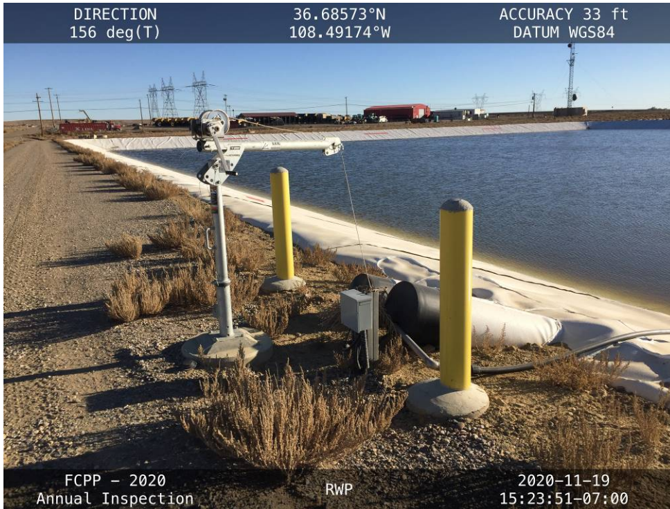
20201119 – IMG_3862 The LCRS riser pipes and crane on the north side of the RWP.
