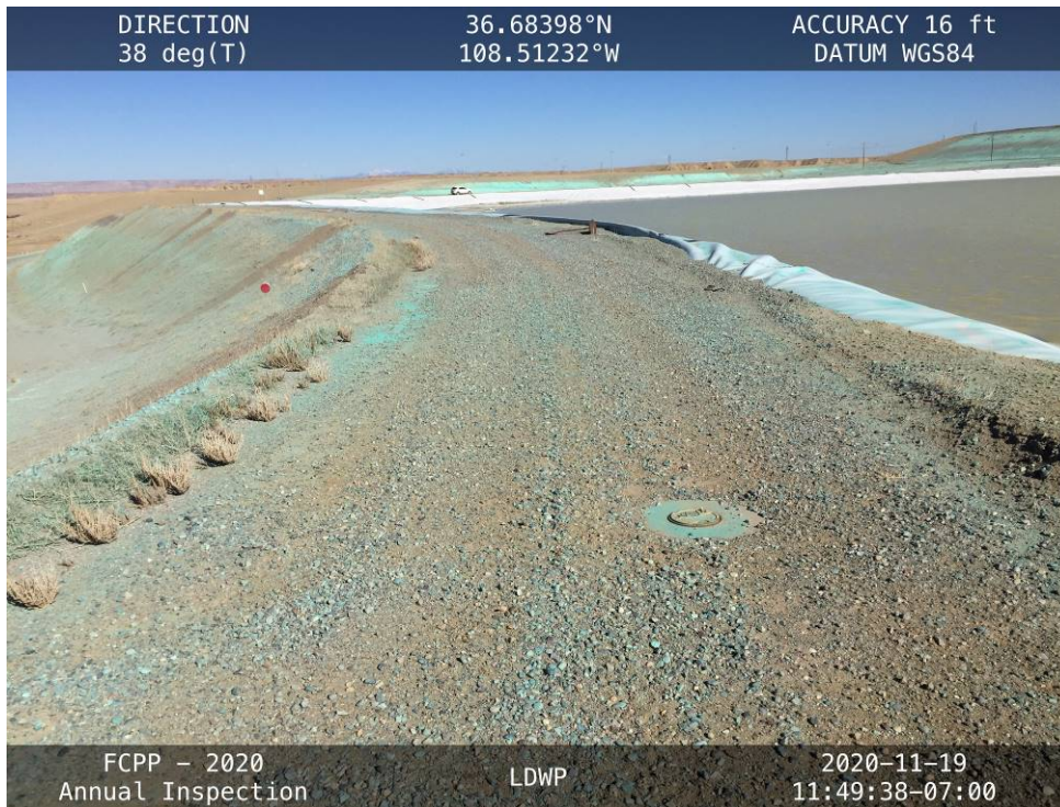
20201119 – IMG_3708 The liner pulling out of the anchor trench in the northern portion of the West Embankment.
