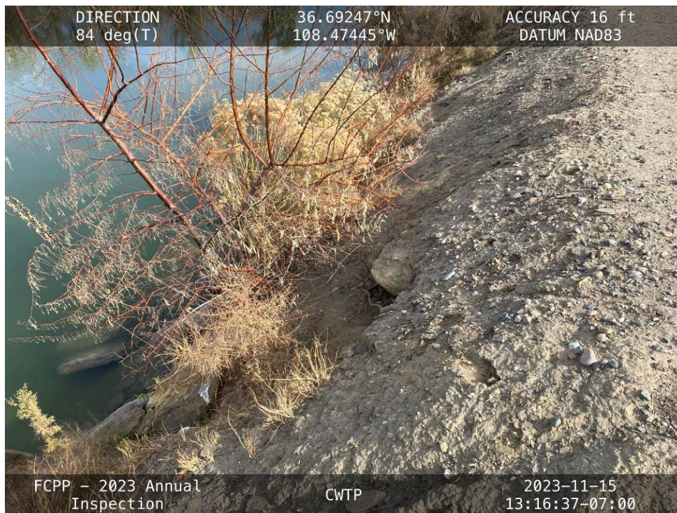
20231115 – IMG_2837 Erosion undermining a riprap boulder on the downstream slope of the North Embankment.
