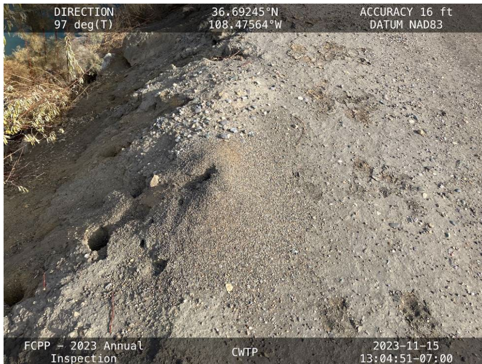
20231115 – IMG_2806 Shallow holes and an ant hill on the downstream shoulder of the North Embankment where there were depressions in 2021 and 2022 (2021 IMG_8448, 2022 IMG_3998).
