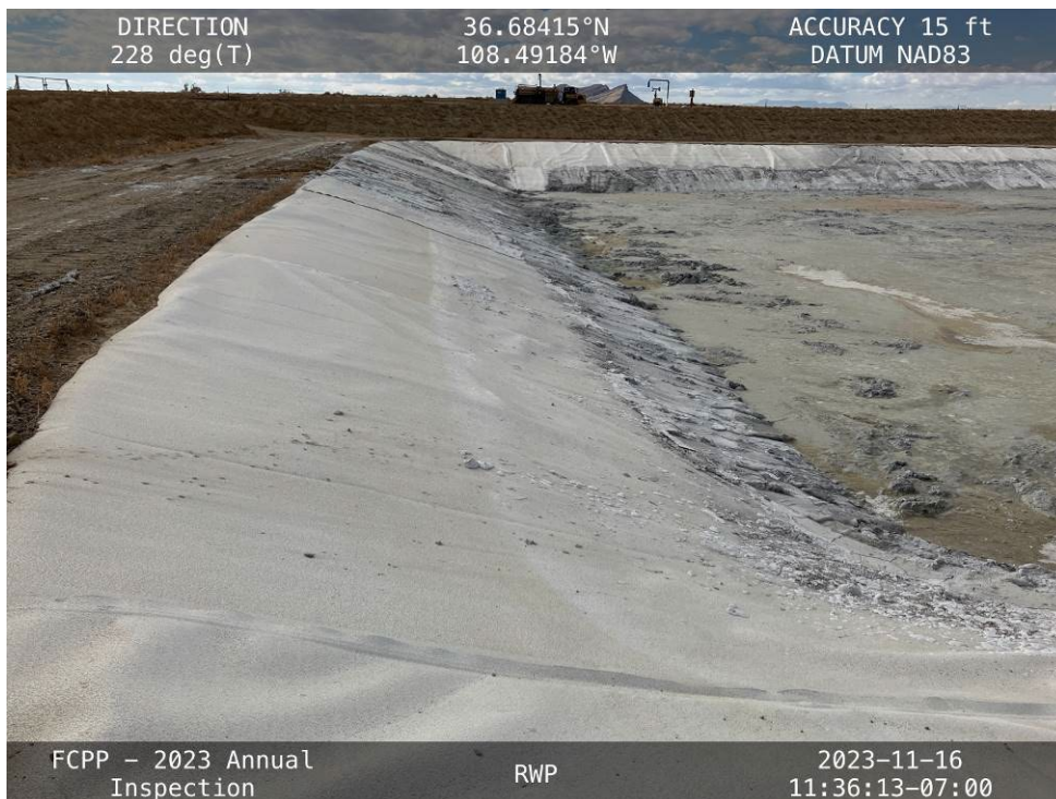
20231116 – IMG_3127 The upstream southeast slope of the FGD Pond cell, facing southwest.
