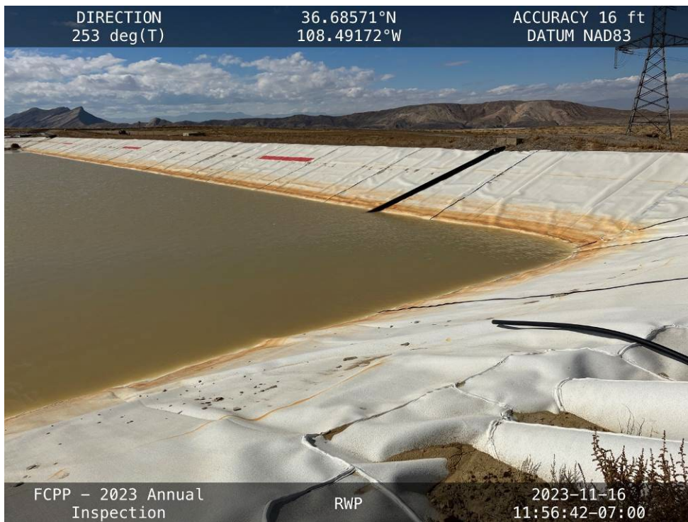
20231116 – IMG_3213 The upstream slope of the Northwest Embankment, facing southwest from the north corner.
