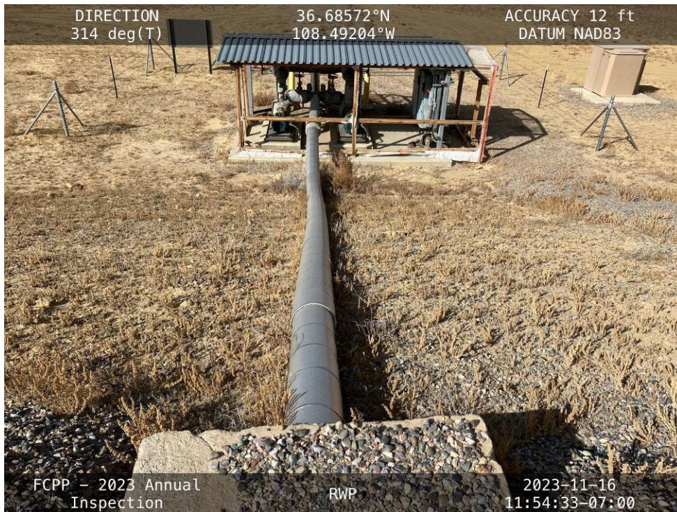
20231116 – IMG_3196 The return water pipe and pumps along the downstream slope of the Northwest Embankment.
