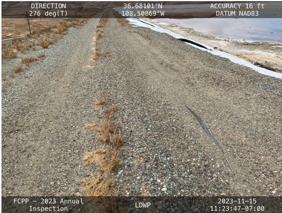
20231115 – IMG_2715 A rut in the crest of the South Embankment.
