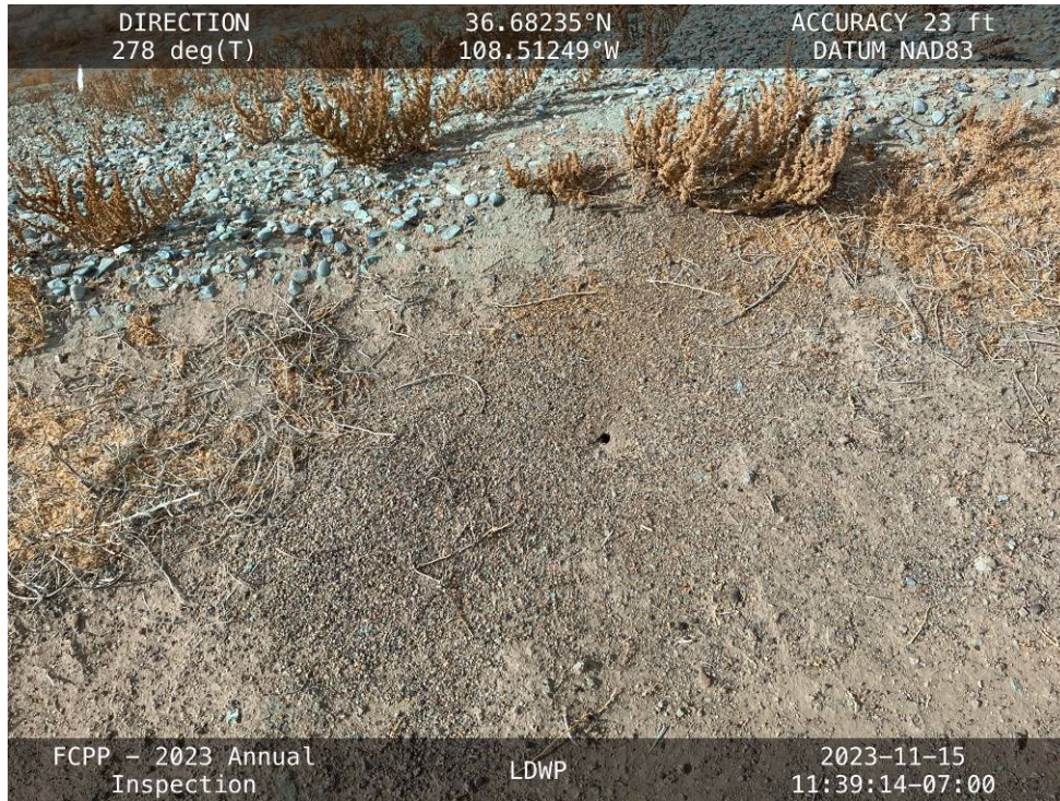
20231115 – IMG_2739 An ant hill on the downstream shoulder of the West Embankment.
