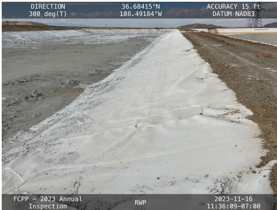
20231116 – IMG_3125 The upstream northeast slope of the FGD Pond Internal Embankment, facing northwest.
