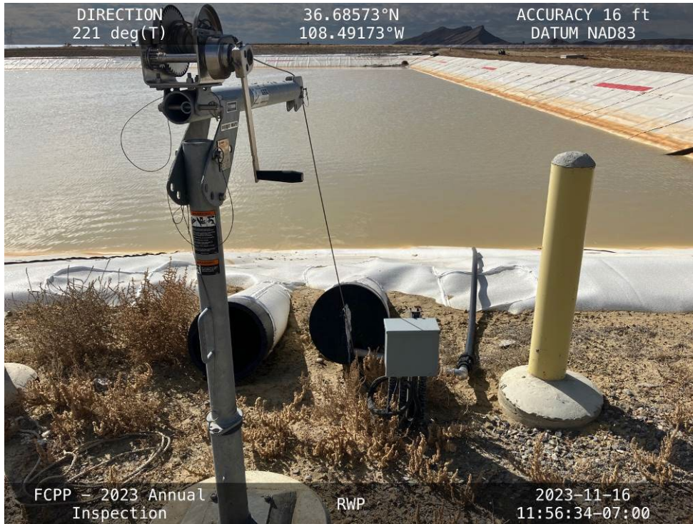
20231116 – IMG_3212 The LCRS riser pipes and crane on the north side of the RWP.
