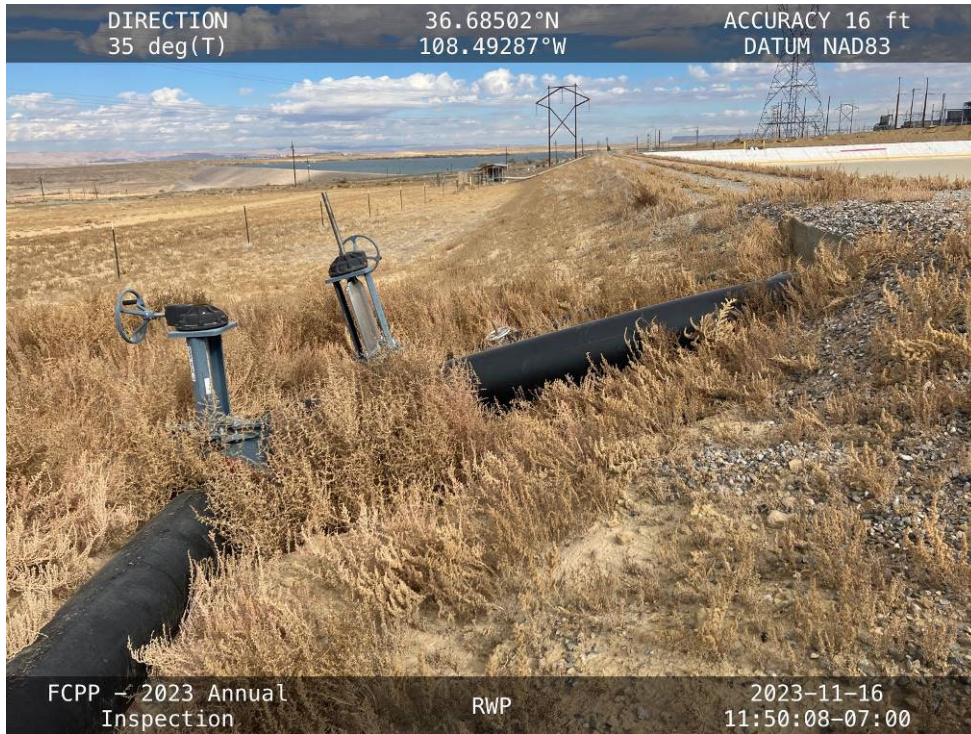
20231116 – IMG_3182 Connections for the new pipes between the RWP and FGD Pond cells.
