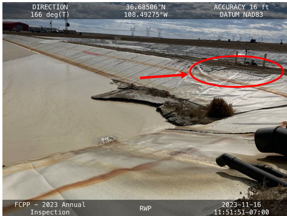
20231116 – IMG_3193 The western corner of the RWP cell Internal Embankment, with loose liner where previous construction activity took place (arrow).
