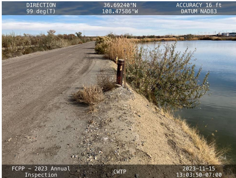
20231115 – IMG_2801 Vegetation to be removed from the upstream slope.
