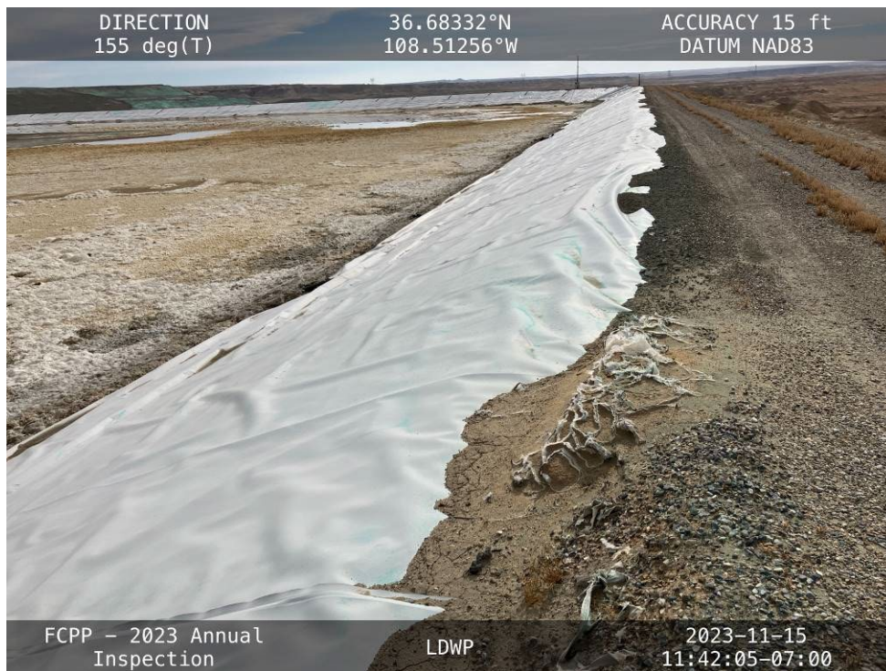
20231115 – IMG_2744 The upstream slope along the southern half of the West Embankment, facing south.
