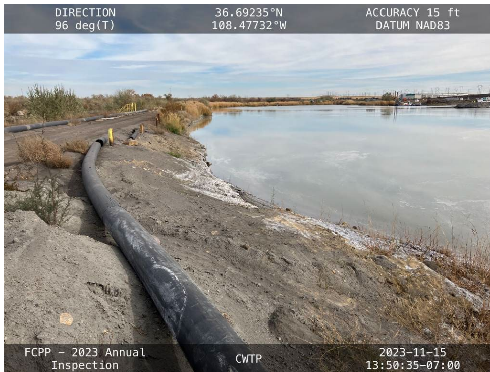
20231115 – IMG_2900 The upstream slope of the North Embankment, facing east from the Left Abutment.
