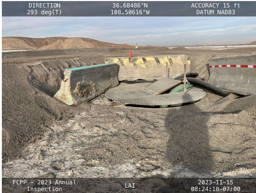
20231115 – IMG_2382 The Drop Inlet Structure, facing west from inside the LAI reservoir.
