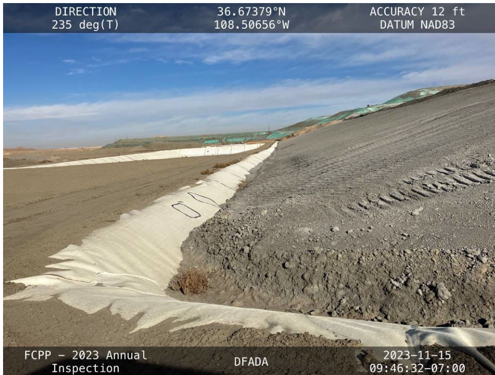
20231115 – IMG_2535 The western toe of Cell 4, facing north from the south end.
