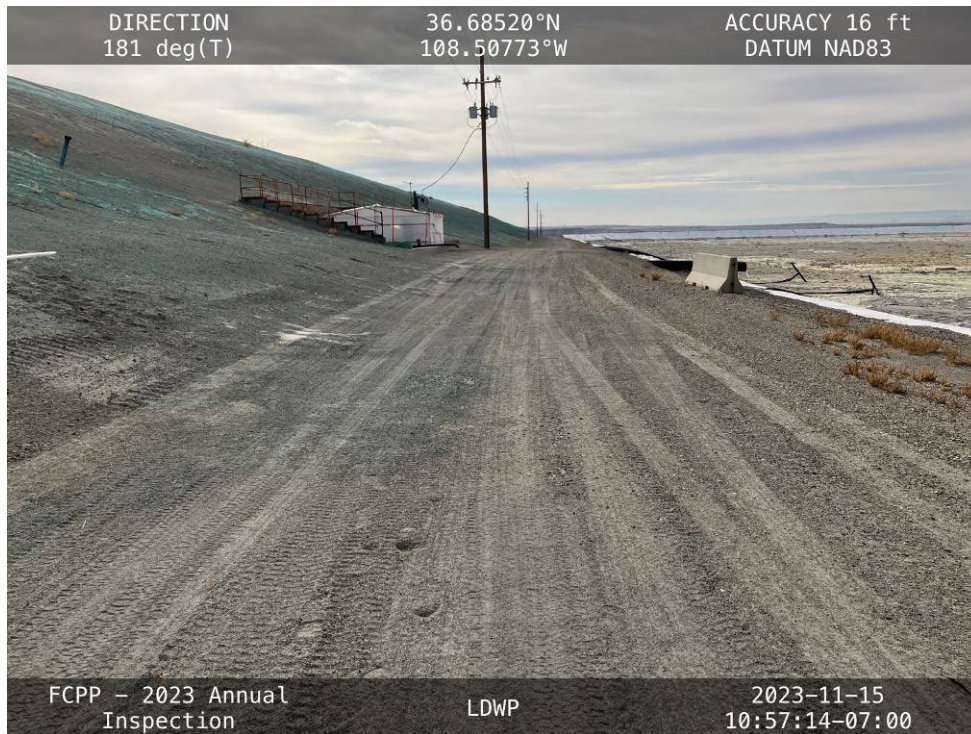
20231115 – IMG_2651 The crest of the East Embankment, facing south from the northeast corner.
