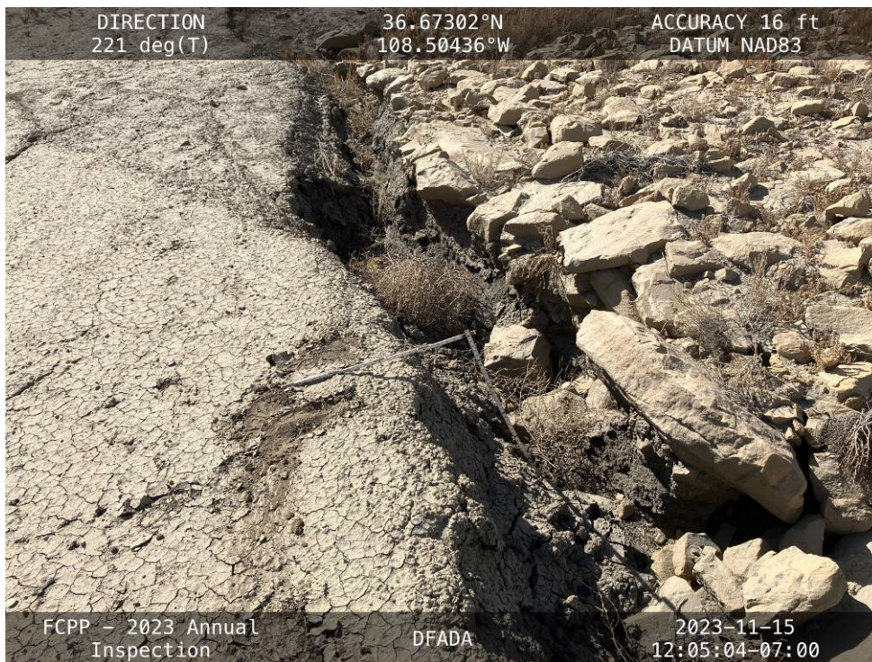
20231115 – IMG_2781 3.5 feet of erosion at the outlet for the Stormwater Diversion Channel.
