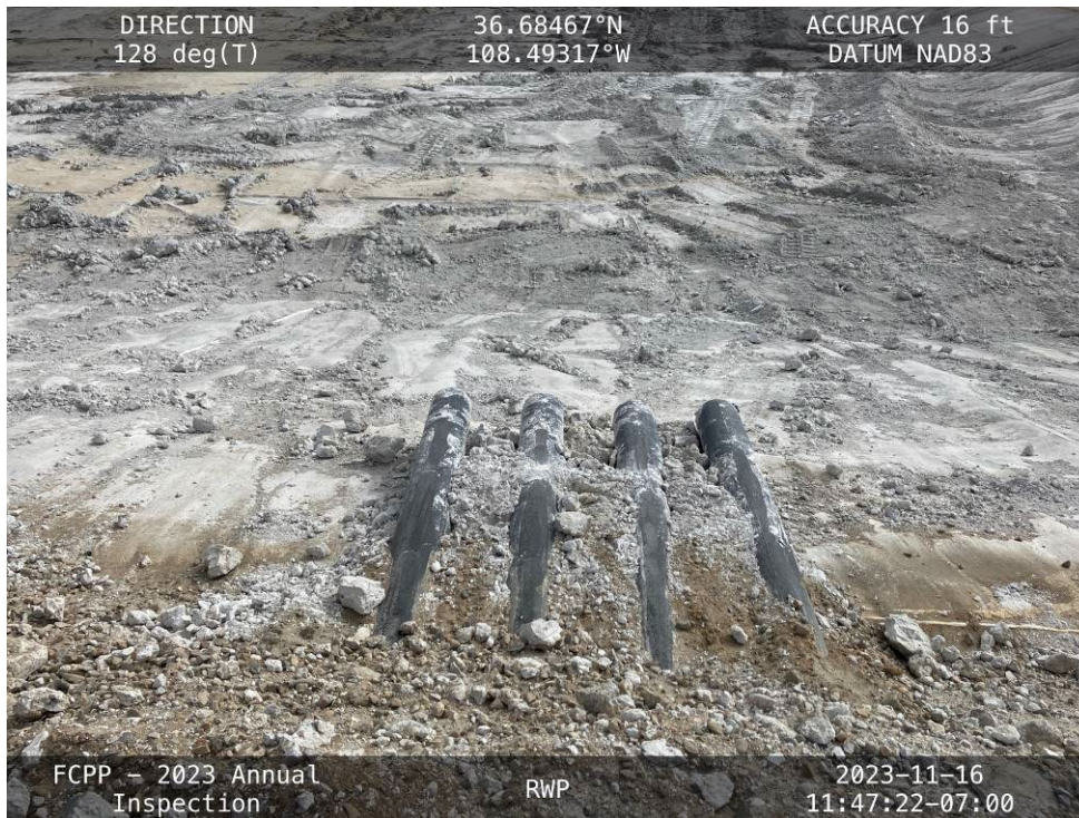
20231116 – IMG_3164 The FGD Pond Inlet Pipes.
