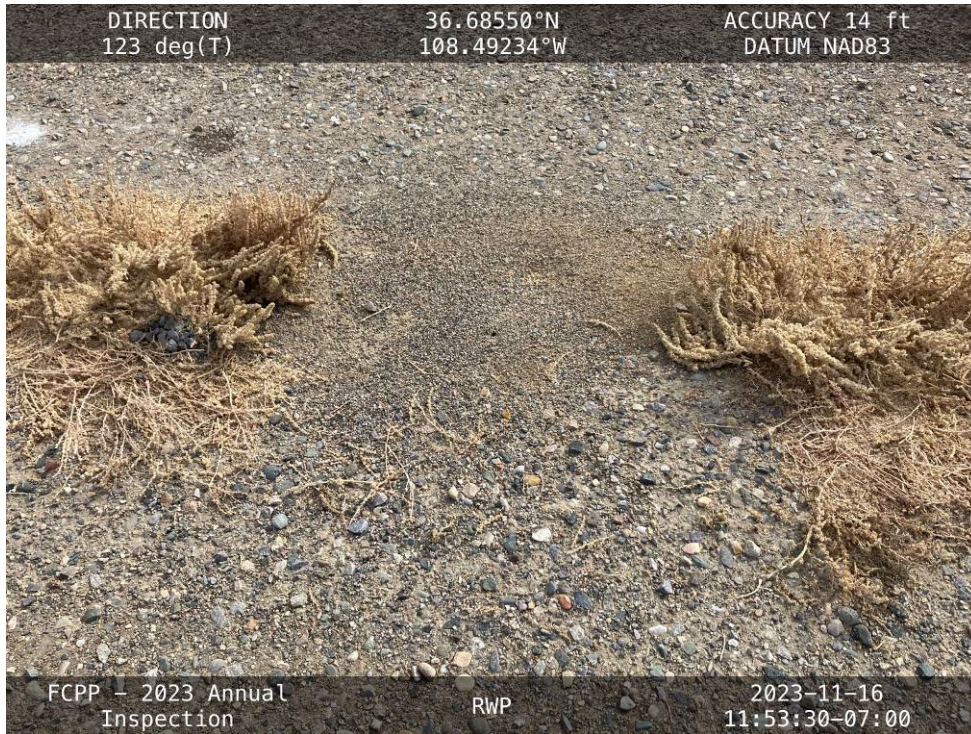
20231116 – IMG_3195 An ant hill on the RWP Northwest Embankment crest.
