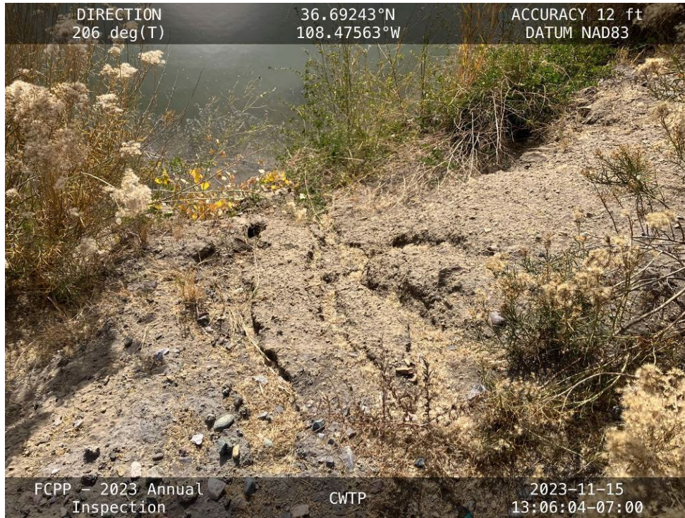
20231115 – IMG_2810 Erosion rills forming on the upstream slope.
