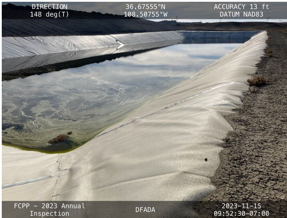
20231115 – IMG_2545 The Cell 4 leachate collection pond, as seen from its northwest corner.
