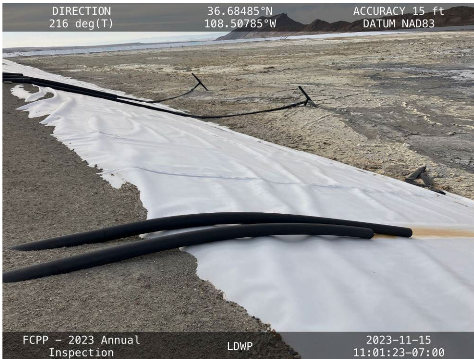
20231115 – IMG_2665 The suction intake lines in the northeast corner of the LDWP.
