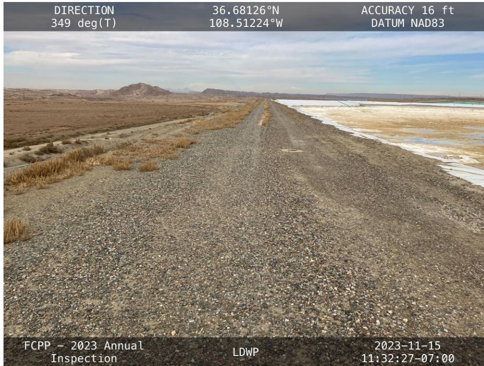
20231115 – IMG_2729 The crest of the West Embankment, facing north from the south end.
