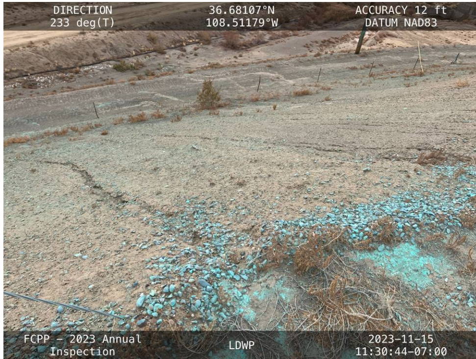
20231115 – IMG_2721 Shallow erosion rills on the downstream slope of the South Embankment.
