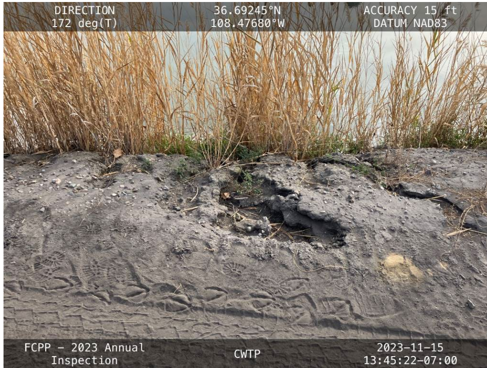
20231115 – IMG_2898 Erosion along the upstream slope of the North Embankment.
