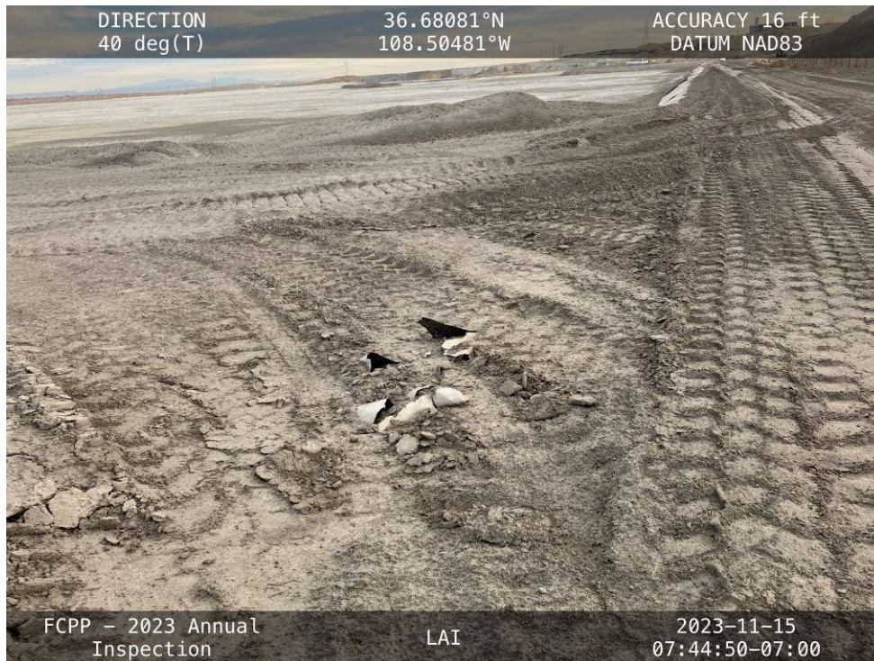
20231115 – IMG_2306 Liner tears at an access ramp into the reservoir.
