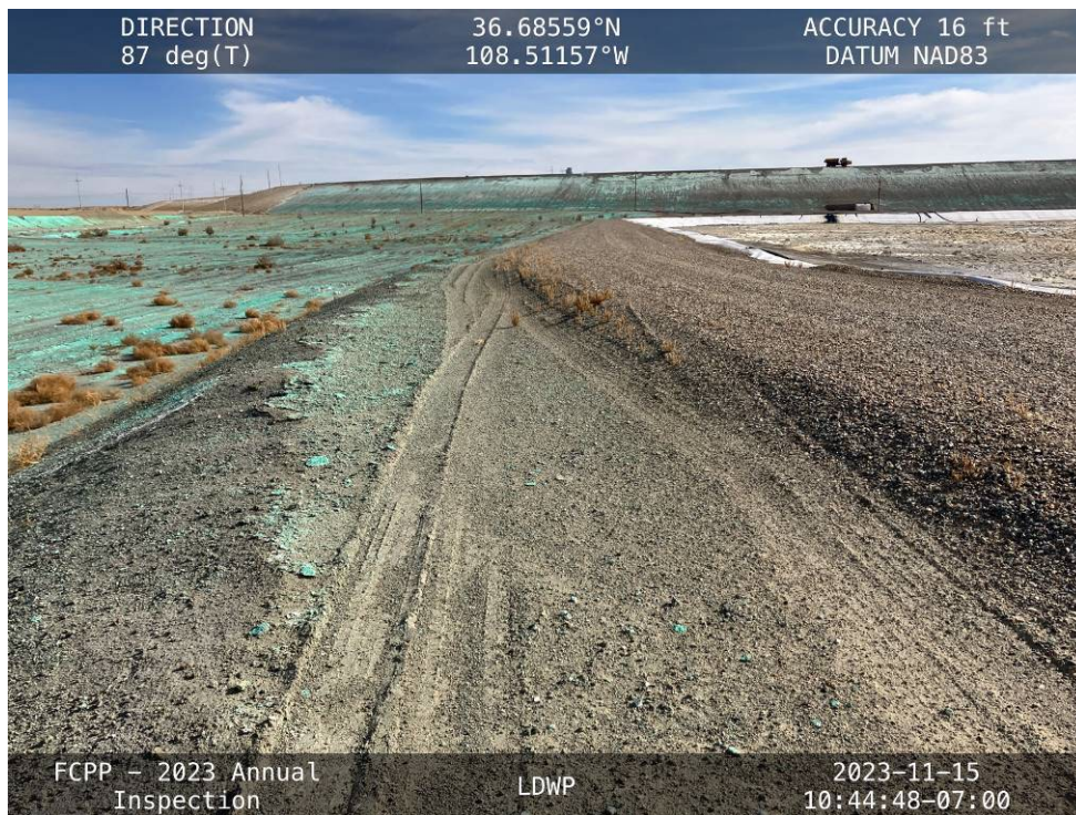
20231115 – IMG_2618 The crest of the North Embankment, facing east from the West Embankment.
