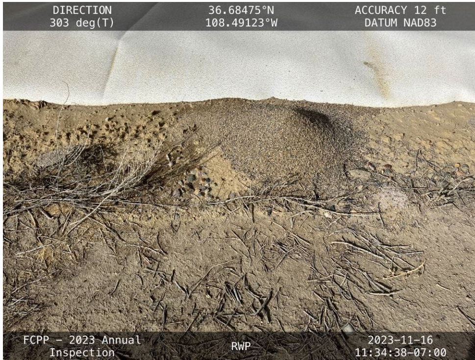
20231116 – IMG_3121 An ant hill on the crest of the Southeast Embankment.
