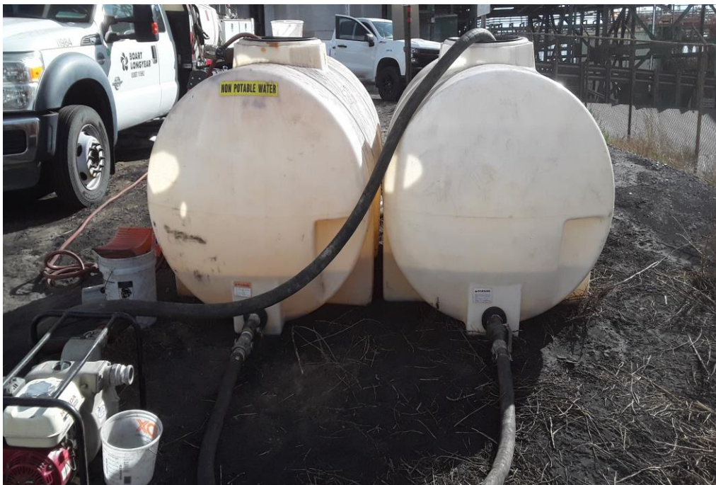
Photo 35: Discharge bins used during pumping at CM-01 and CM-02.
