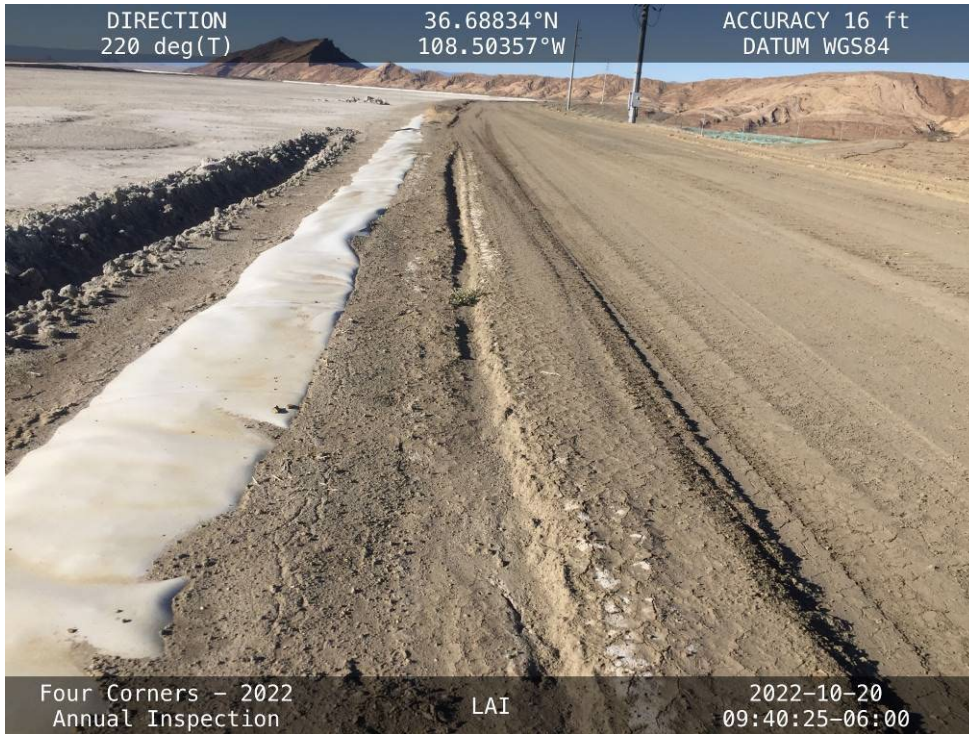
20221020 – IMG_4507 Ruts on the upstream side of the Northwest Embankment crest.
