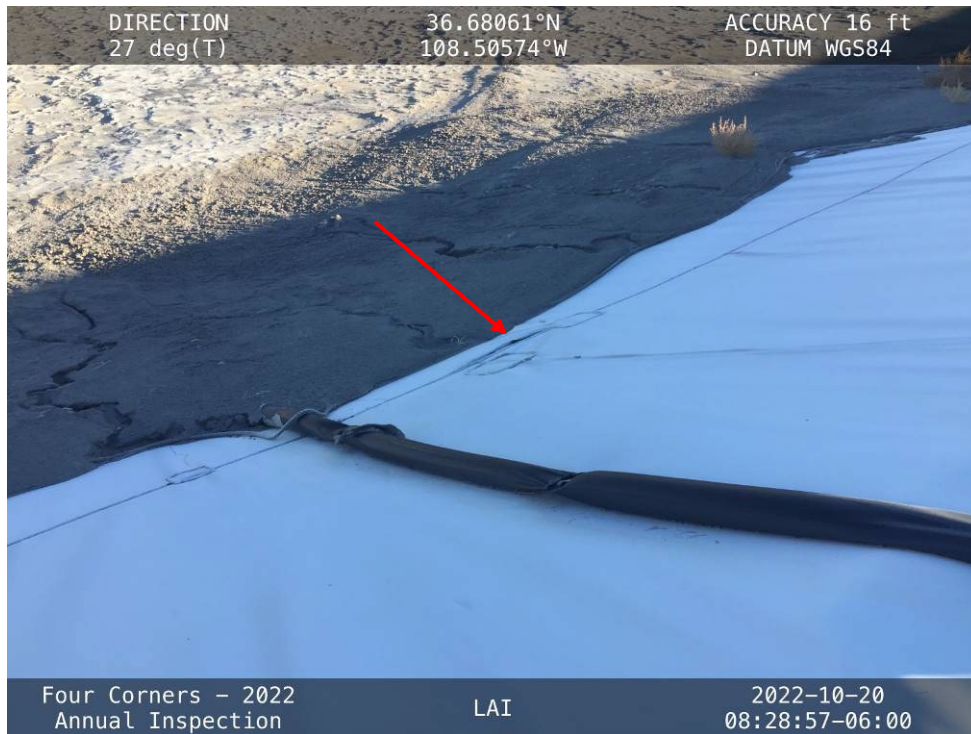
20221020 – IMG_4429 A tear along the horizontal seam in the liner.
