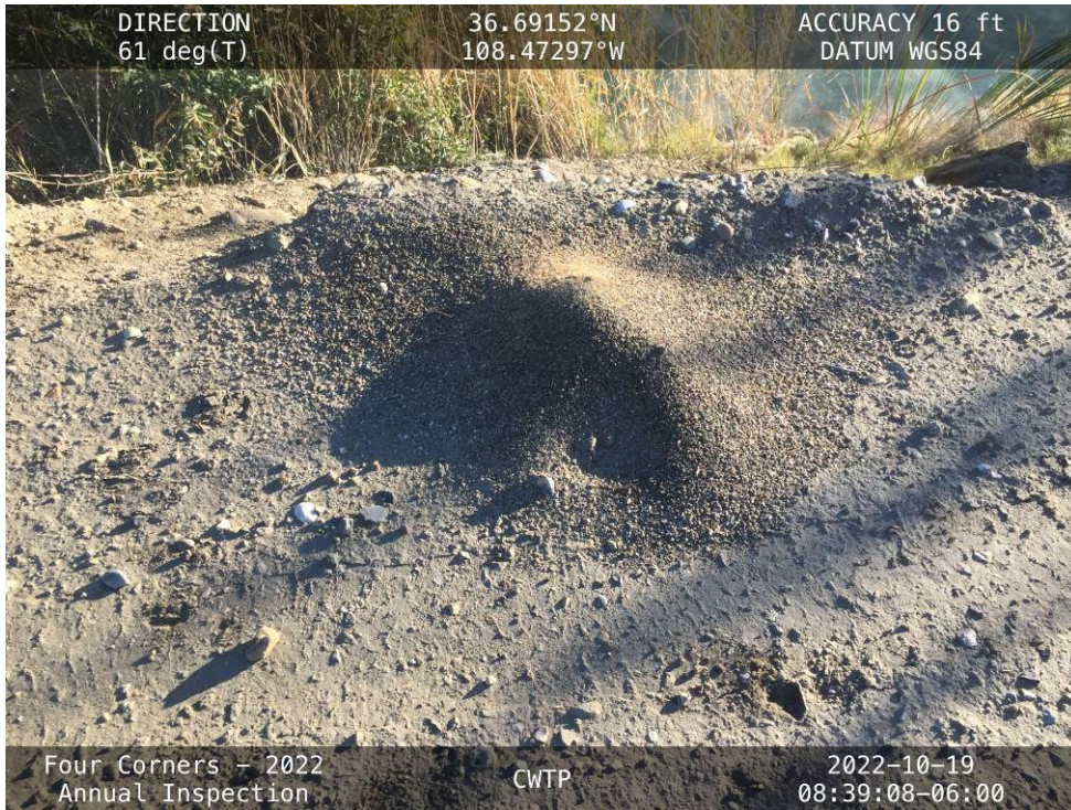
20221019 – IMG_4045 An ant hill on the downstream shoulder of the embankment.
