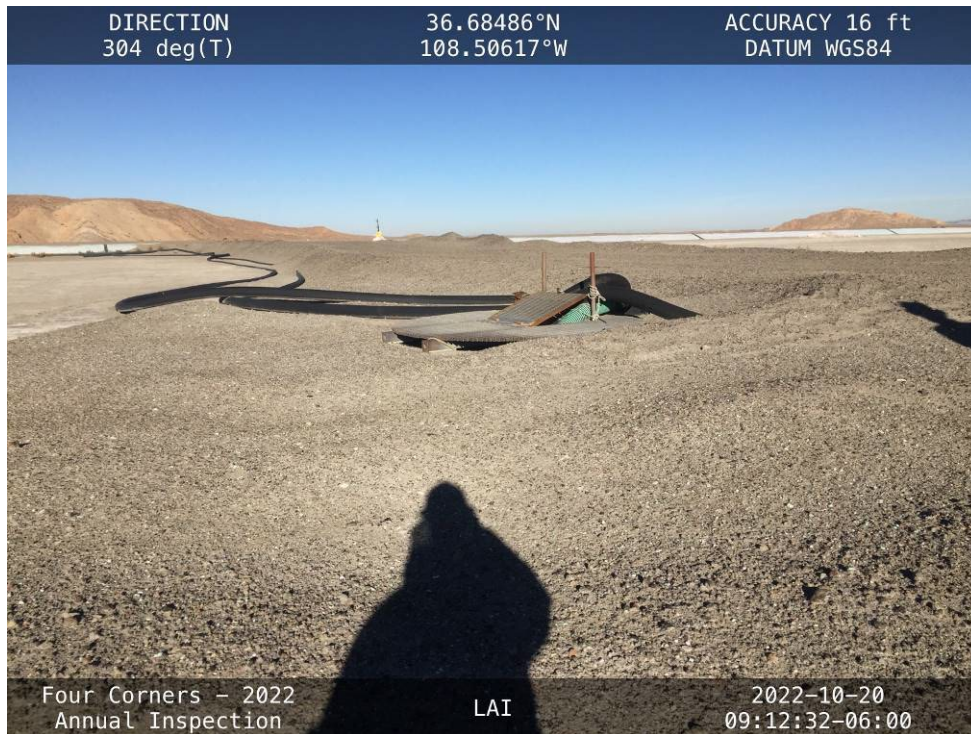
20221020 – IMG_4477 The Drop Inlet Structure, facing west from inside the LAI reservoir.
