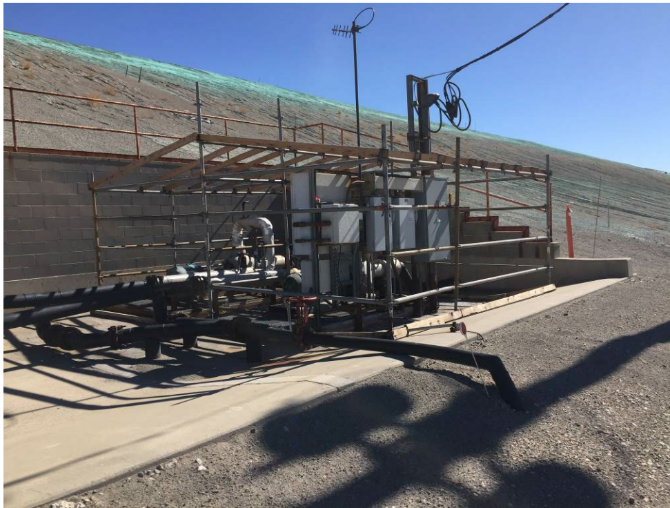
20221020 – IMG_4828 The LAI/LDWP pump station.
