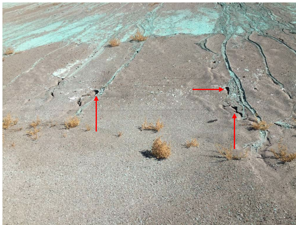
20221020 – IMG_4876 Erosion rills on the West Embankment, undermined beneath the dust suppressant.
