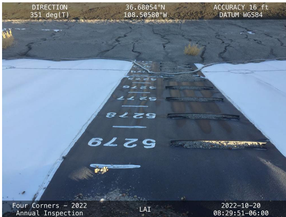
20221020 – IMG_4430 The LAI staff gage at STA 36+00 at the time of the inspection.
