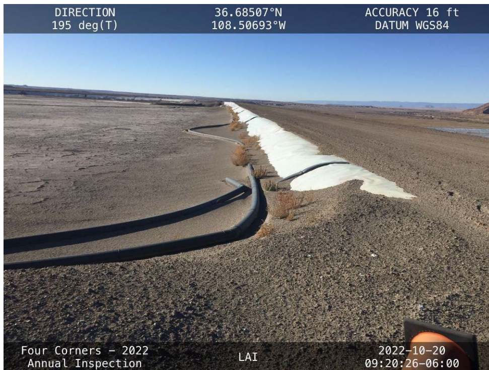
20221020 – IMG_4484 The upstream slope of the West Embankment, facing south from the Drop Inlet Structure ramp.
