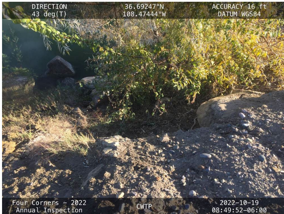
20221019 – IMG_4087 Erosion and vegetation to be removed from the downstream slope.
