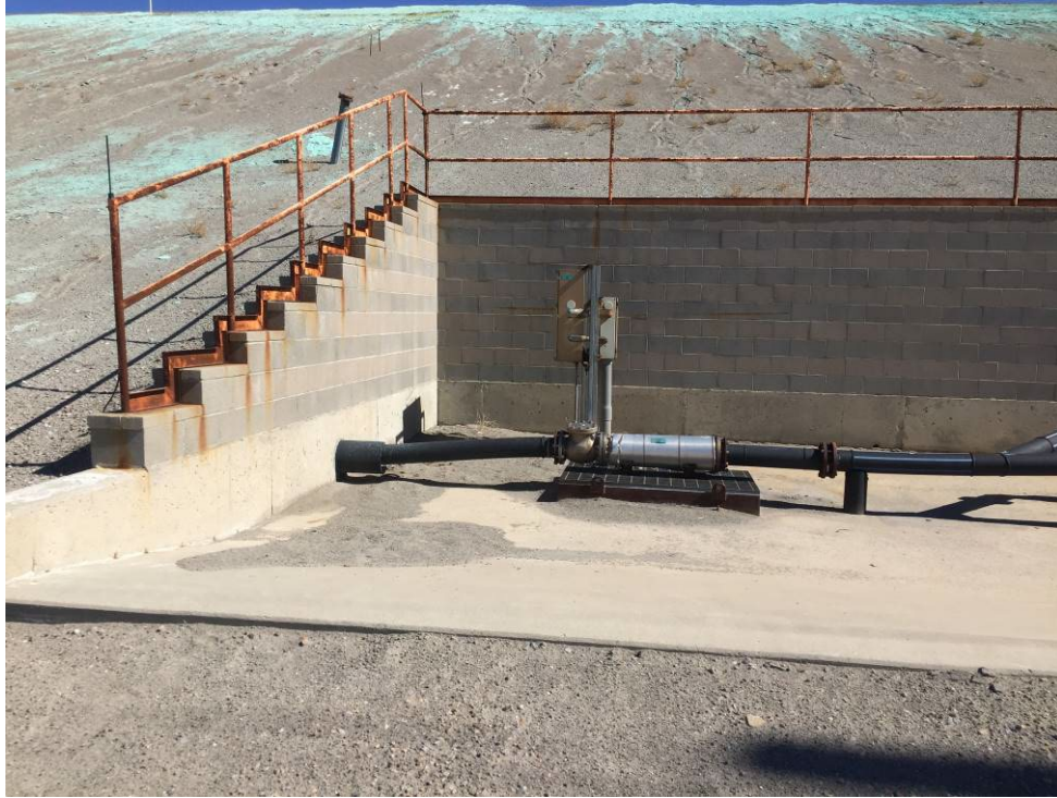
20221020 – IMG_4826 The LAI/LDWP pump station.
