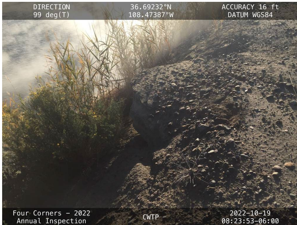
20221019 – IMG_4017 Erosion beneath a riprap boulder on the downstream slope.
