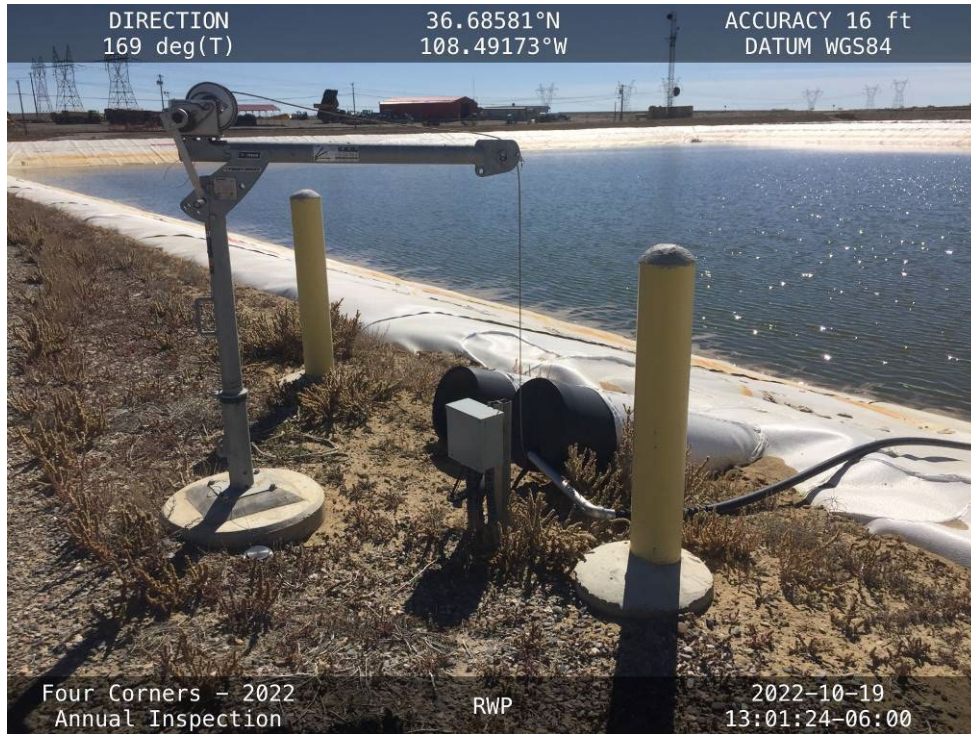
20221019 – IMG_4320 The LCRS riser pipes and crane on the north side of the RWP.
