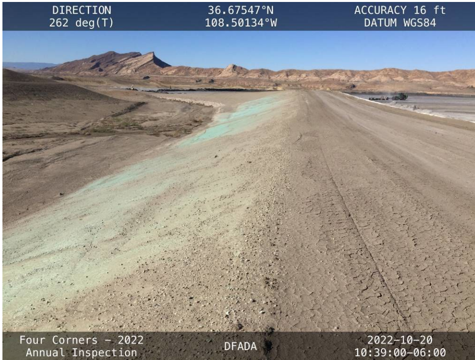
20221020 – IMG_4591 The crest road along the south side of Cell 4, facing west.
