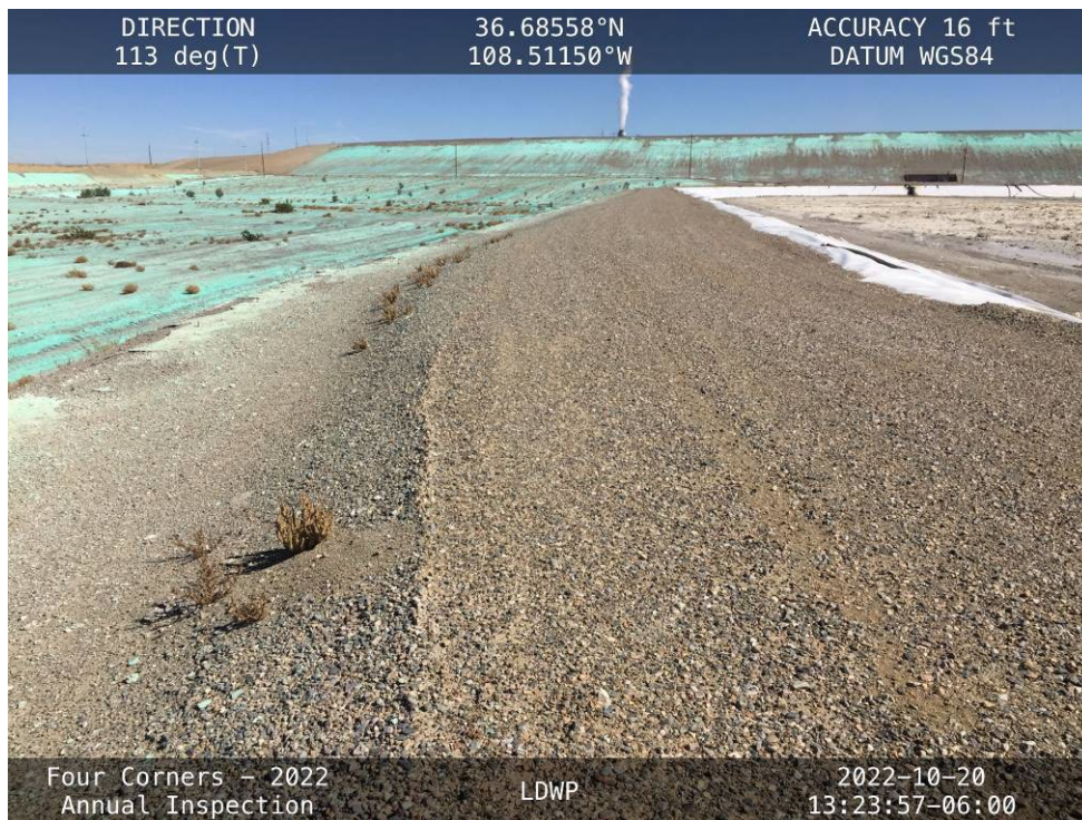
20221020 – IMG_4807 The crest of the North Embankment, facing east from the West Embankment.
