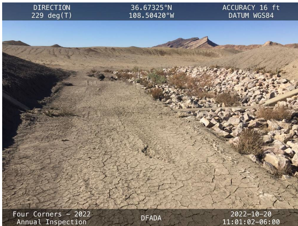
20221020 – IMG_4628 The headwall at the new outlet for the Stormwater Diversion Channel, buried in sediment.
