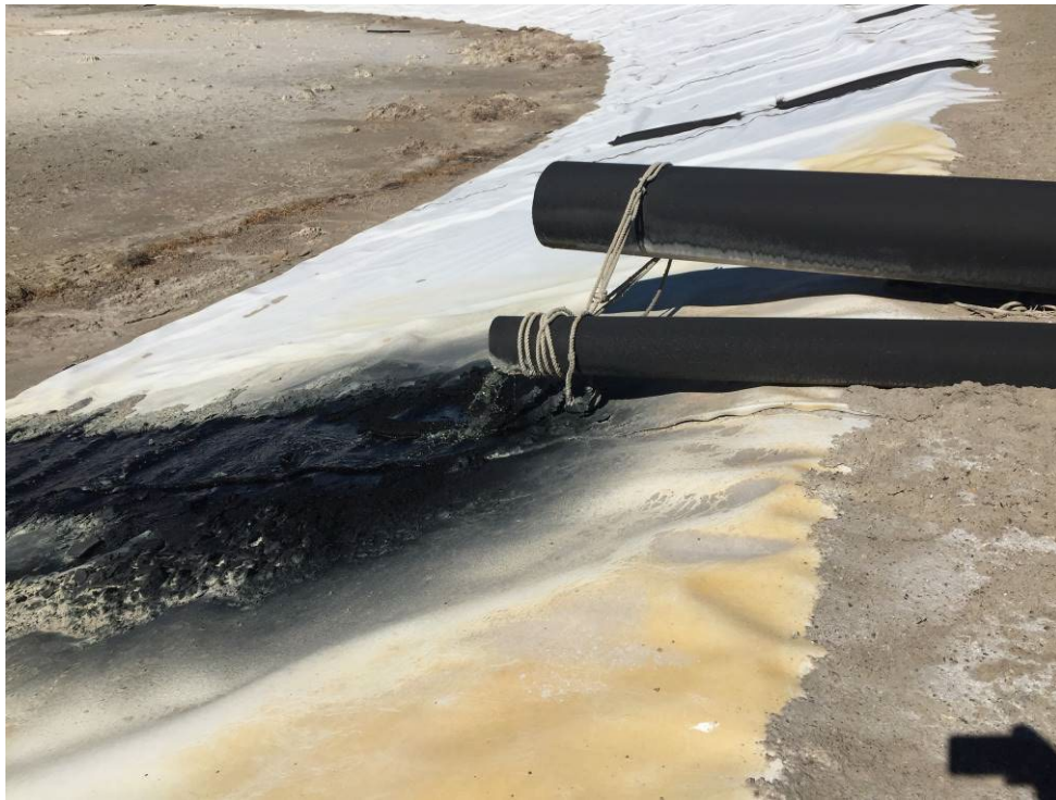
20221020 – IMG_4830 The 8-inch and 16-inch HDPE outlet pipes used to convey decant water from the LAI.
