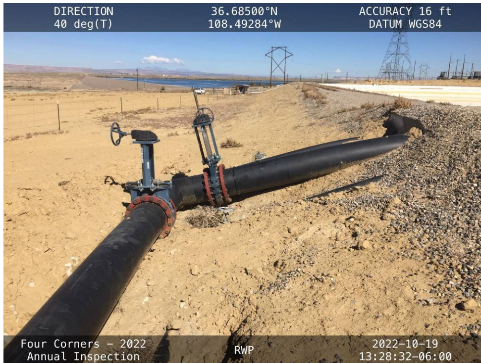
20221019 – IMG_4377 Connections for the new pipes between the RWP and FGD Pond cells.
