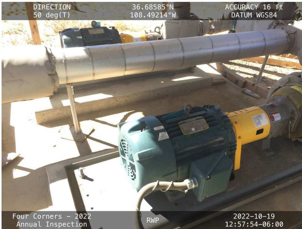
20221019 - IMG_4300 The RWP pumps, no longer leaking.
