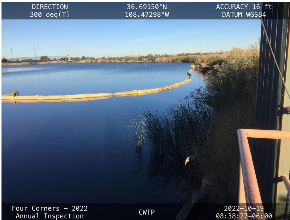
20221019 – IMG_4044 The reservoir and vegetation along the upstream slope of the embankment, facing northwest.
