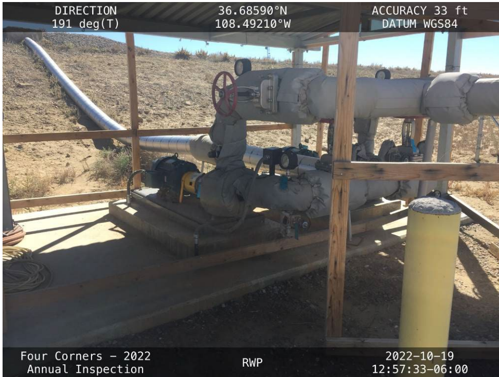
20221019 - IMG_4297 The RWP pumps.
