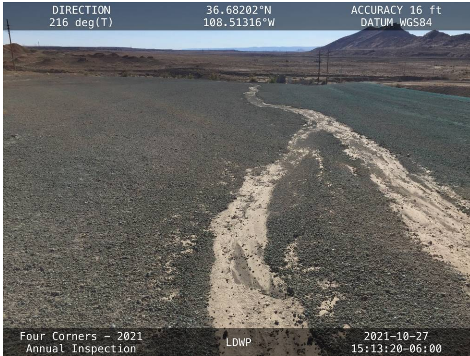
20211027-IMG_8017 Runout channels from the erosion shown in IMG_8015 and IMG_8018.
