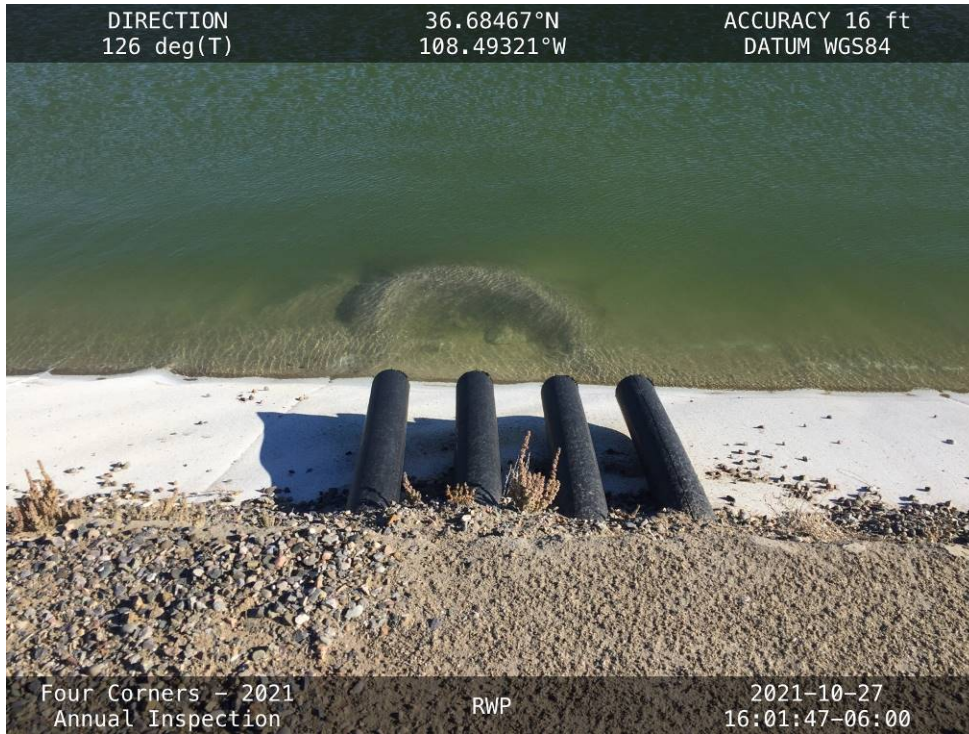
20211027-IMG_8088 The FGD Pond cell Inlet Pipes.
