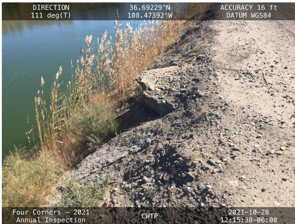
20211028 – IMG_8393 Erosion beneath a riprap boulder on the downstream slope.
