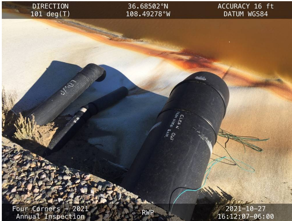
20211027-IMG_8115 The RWP cell inlet pipes.
