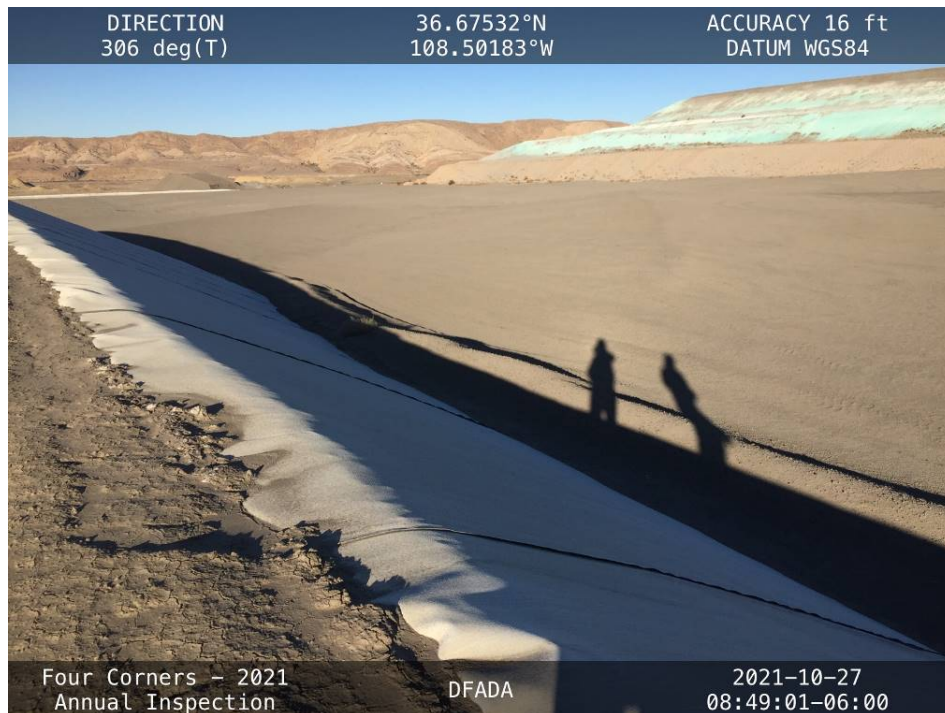
20211027 – IMG_7538 The surface of Cell 4 with the downstream slope of Cell 1 in the background, facing west from the south side of Cell 4.
