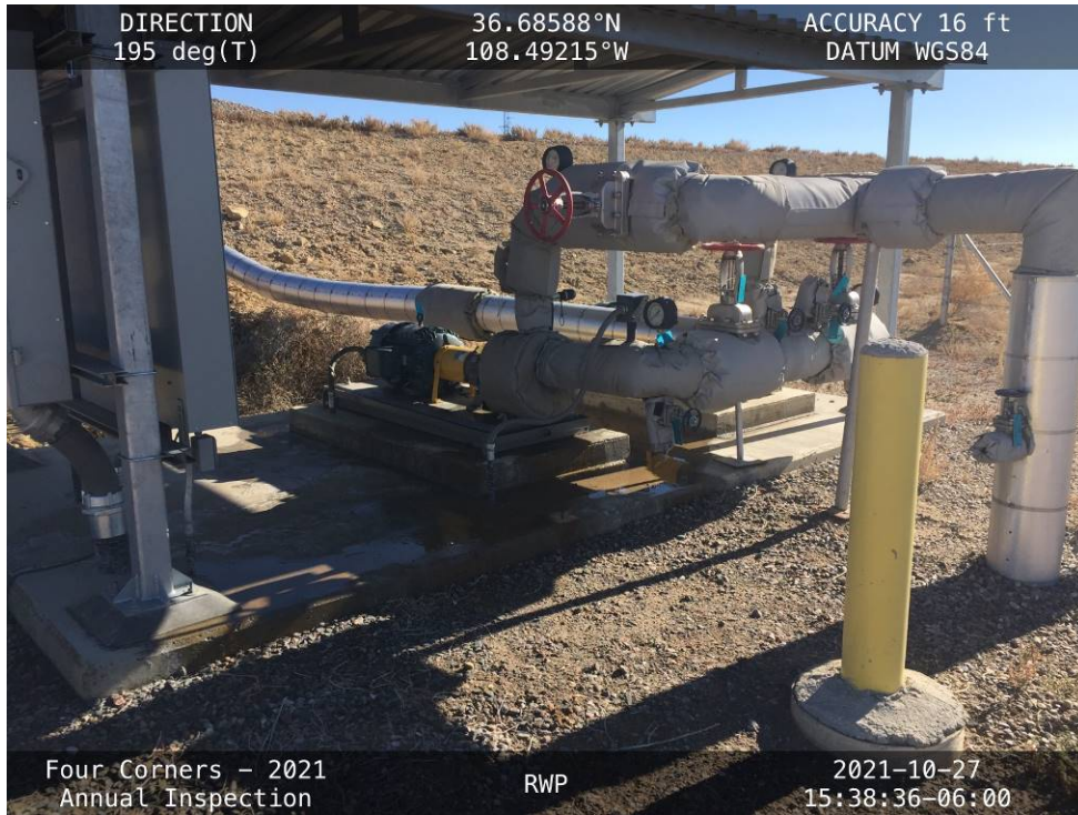
20211027-IMG_8023 The RWP pumps.
