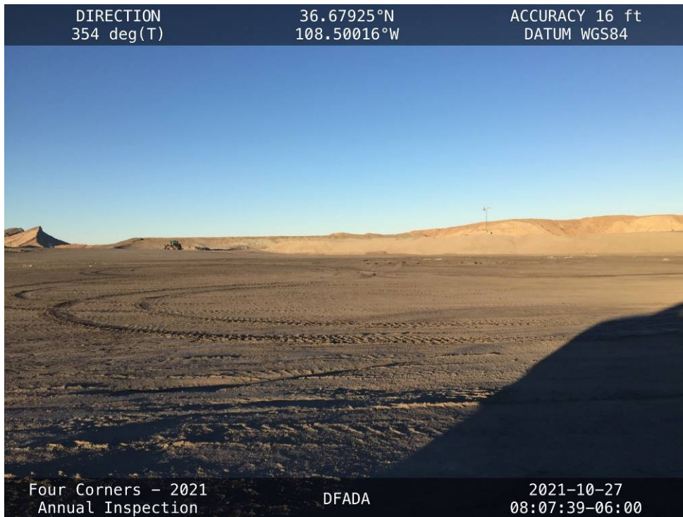
20211027-IMG_7500 The surface of Cell 2, facing north from the middle of the cell.
