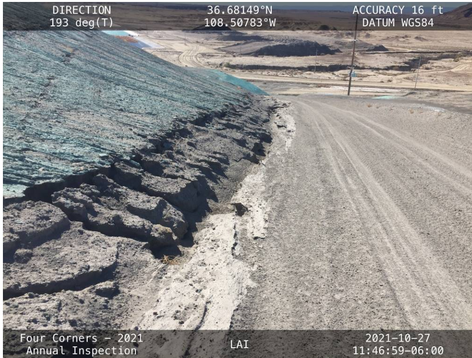
20211027-IMG_7753 Erosion on the LDWP access ramp, facing south.
