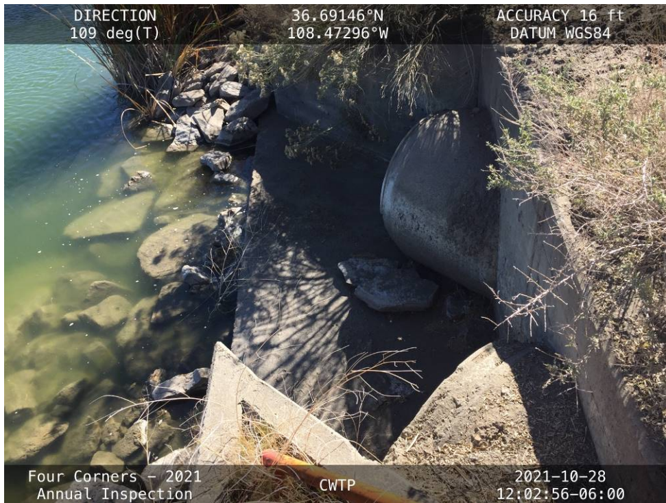
20211028-IMG_8350 The 30-inch RCP outfall from the CWTP to the discharge canal.
