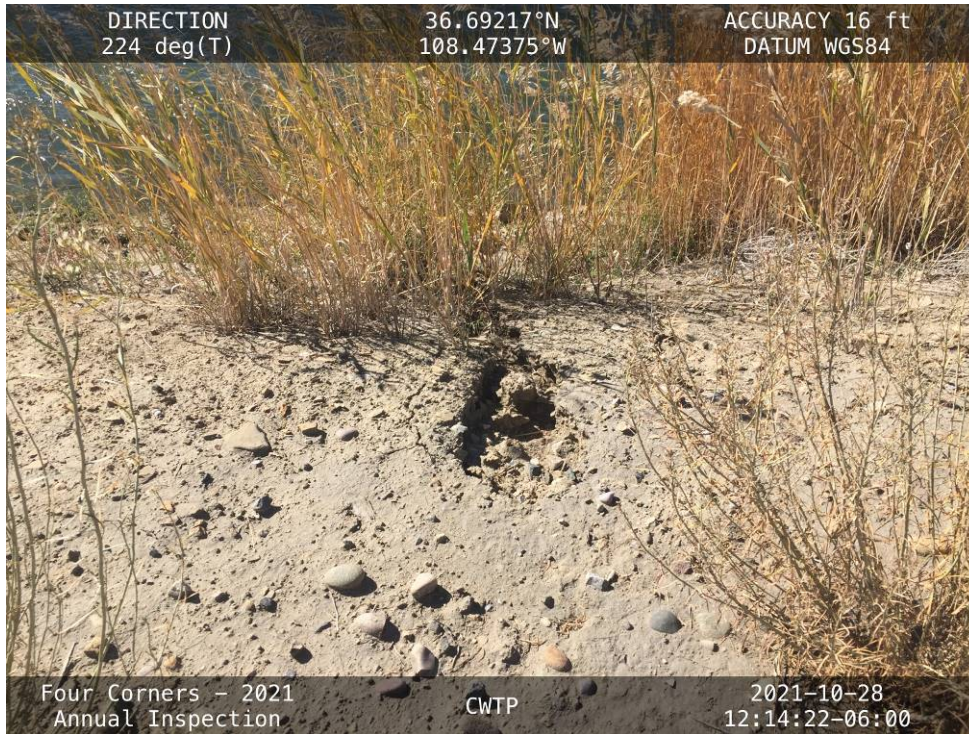
20211028 – IMG_8389 An incipient erosion rill on the upstream slope of the embankment.
