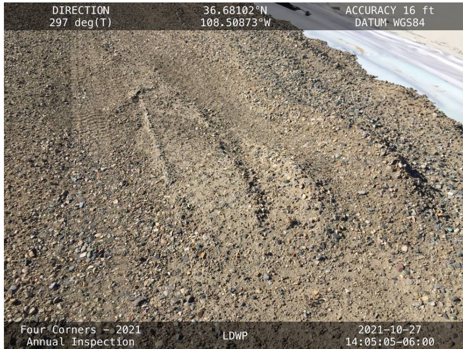
20211027 – IMG_7918 A rut in the crest of the South Embankment.
