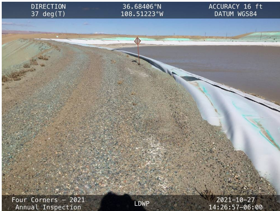
20211027-IMG_7954 The liner pulling out of the anchor trench in the northern portion of the West Embankment.
