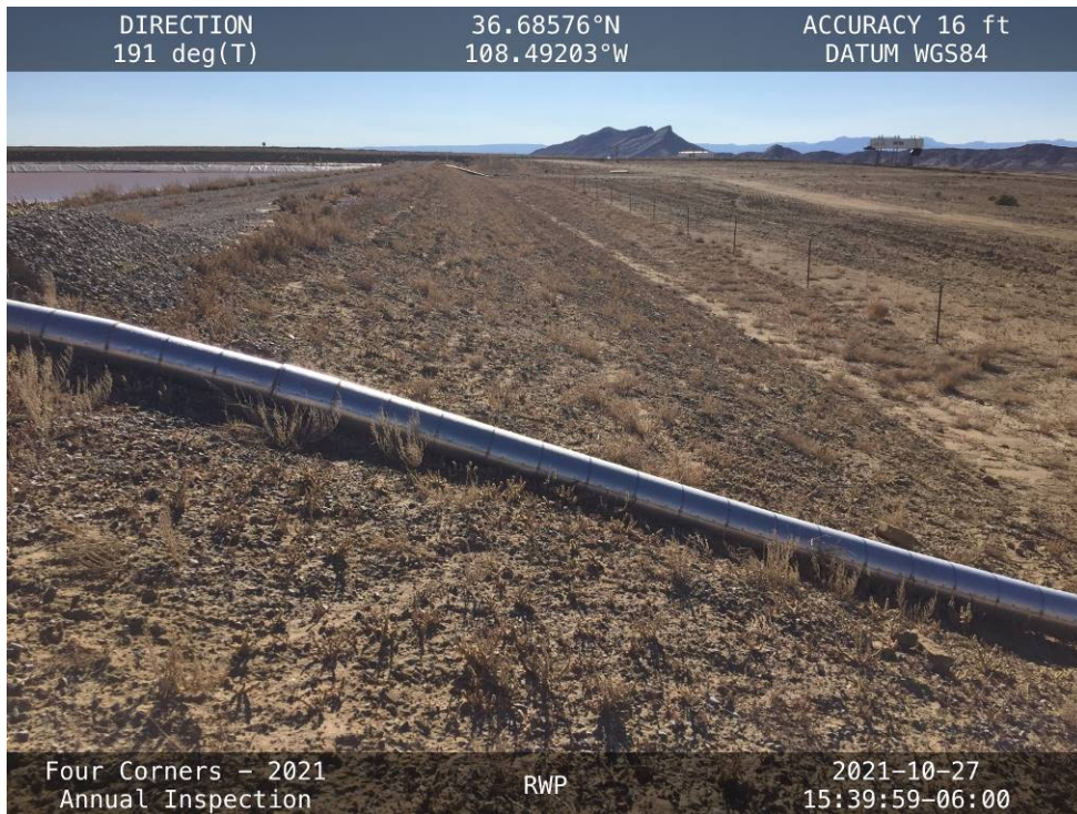
20211027-IMG_8027 The downstream slope of the Northwest Embankment, facing southwest from the north corner.
