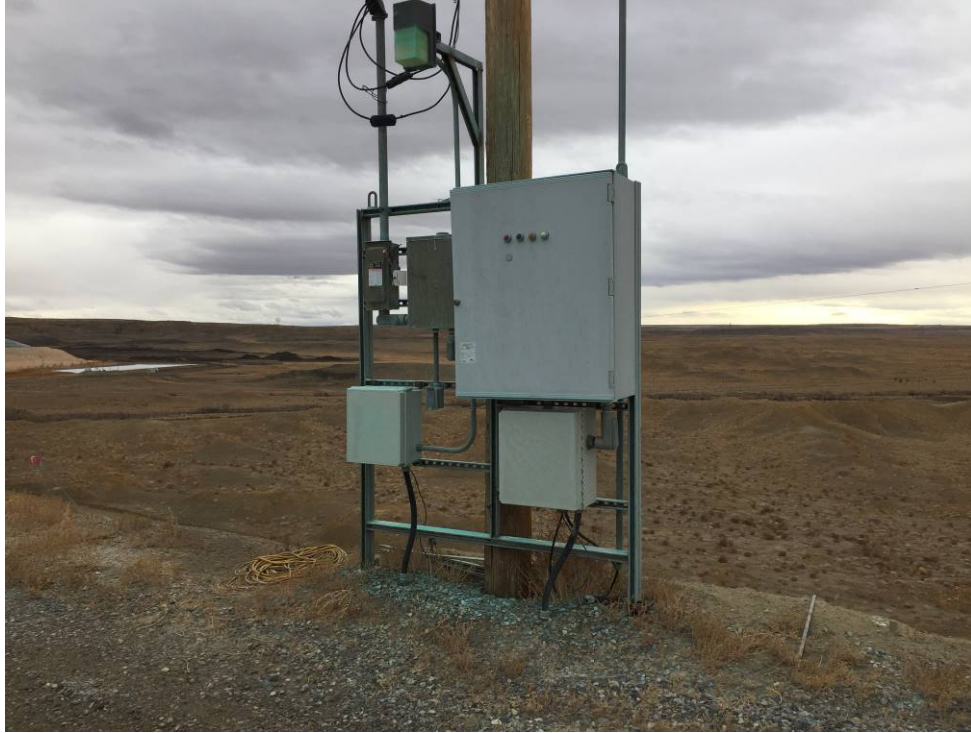
20191120 – IMG_6689 The Interstitial Evacuation Pump control panel.
