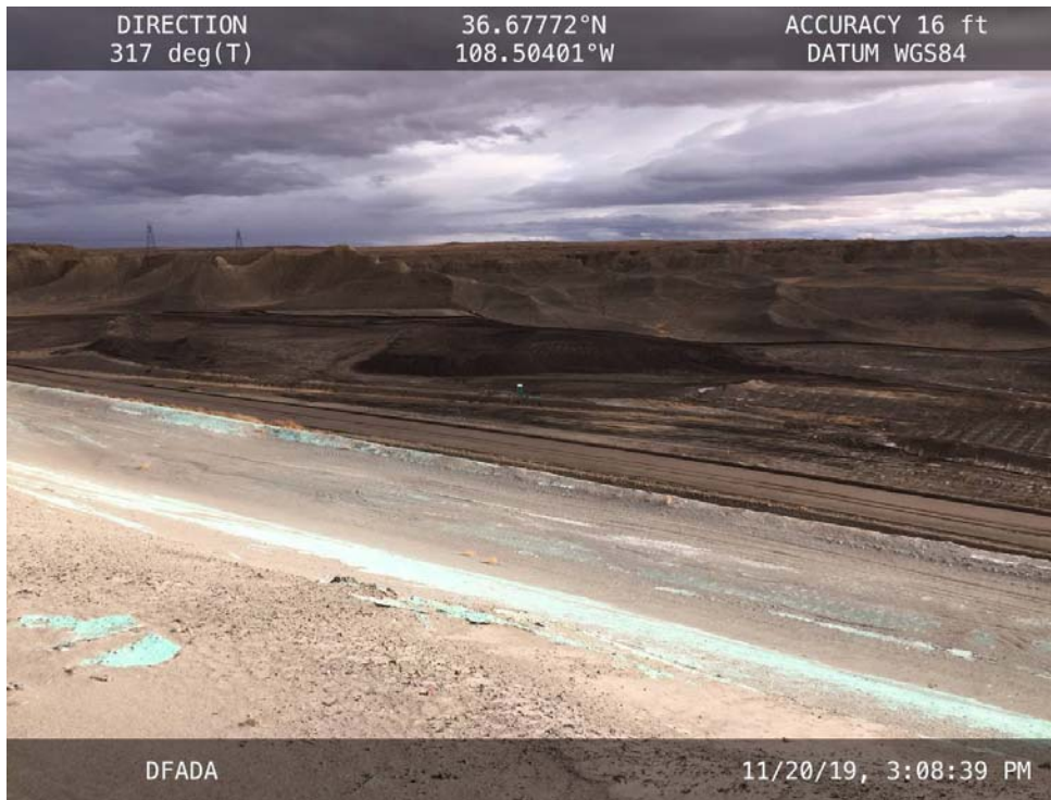
20191120 – IMG_6839 Subgrade preparation in the footprint of the proposed DFADA Site 4, facing south from Cell 1.
