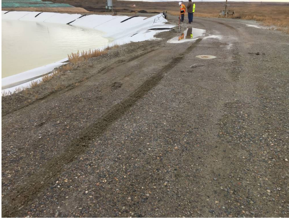
20191120 – IMG_6671 Water ponding on the crest near the Interstitial Evacuation Pump.
