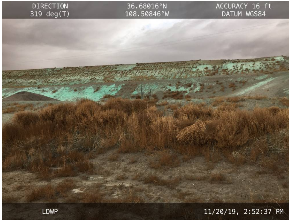
20191120 – IMG_6794 The South Embankment of the LDWP and Ash Pond 3, facing north from the toe.
