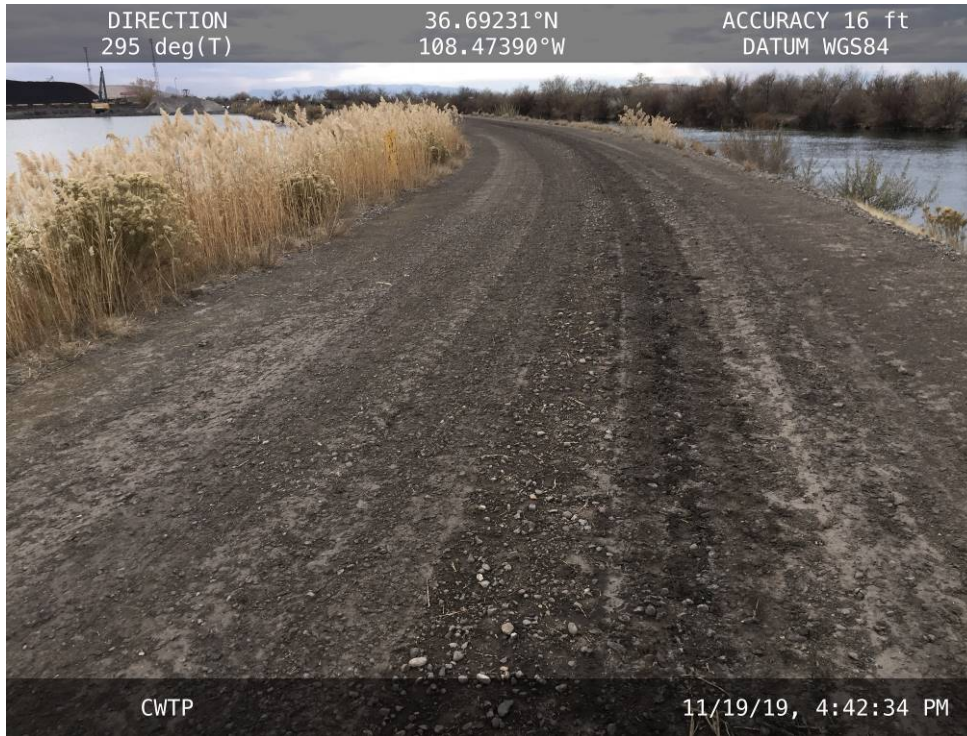
20191119 – IMG_6270 The crest of the CWTP embankment, facing northwest at the curve.
