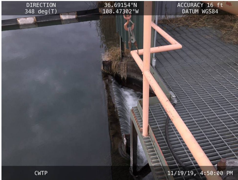
20191119 – IMG_6293 Water flowing over the overflow weir to the outfall.
