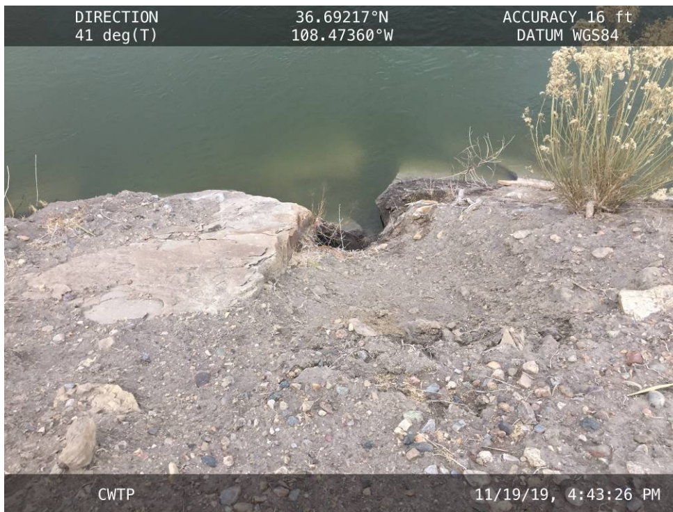
20191119 – IMG_6272 Erosion around the riprap on the downstream slope along the eastern portion of the embankment.
