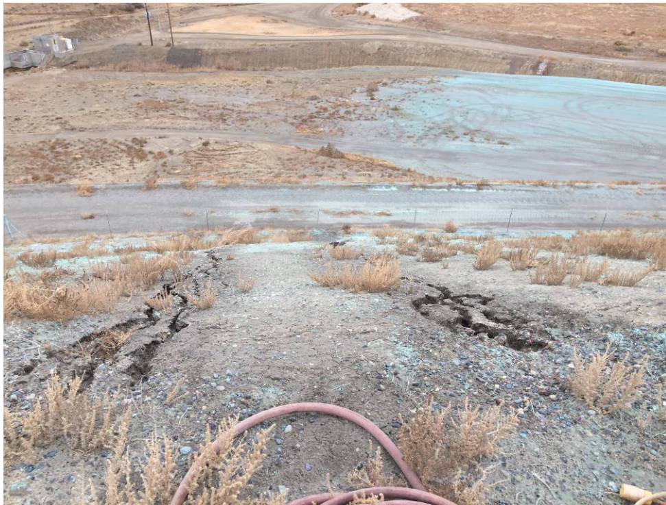
20191120 – IMG_6674 Erosion rills on the downstream slope at the southwest corner of the LDWP.
