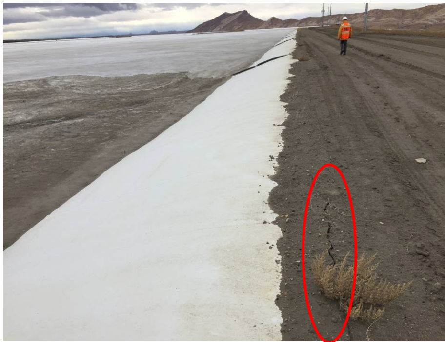
20191120 – IMG_6622 The upstream slope of the Northwest Embankment and a crack in the anchor trench, facing southwest.
