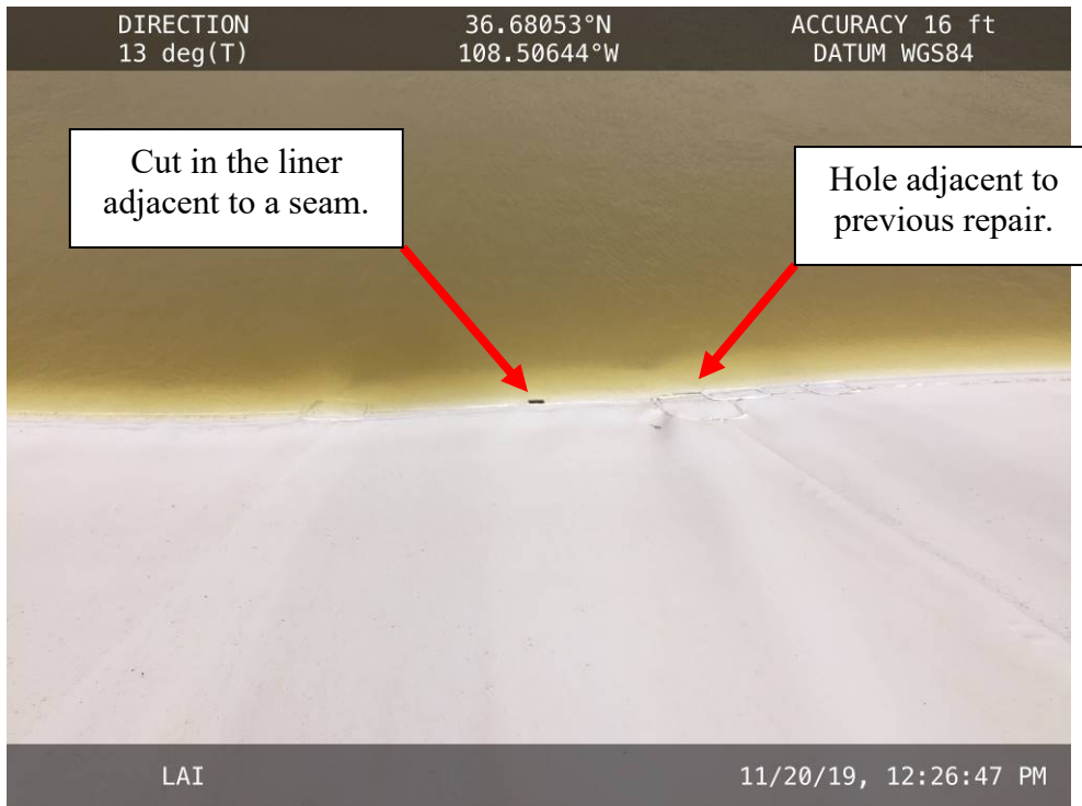
20191120 – IMG_6506 Two holes in the liner along the upstream slope on the South Embankment.
