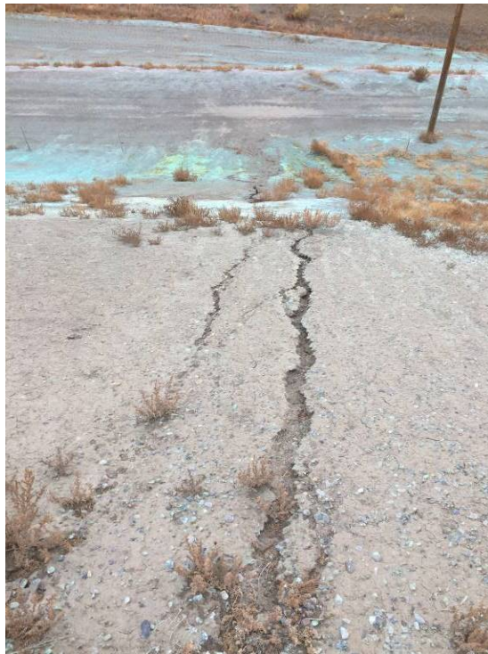
20191120 – IMG_6700 Erosion rills forming in an area of prior repair on the upper half of the South Embankment.
