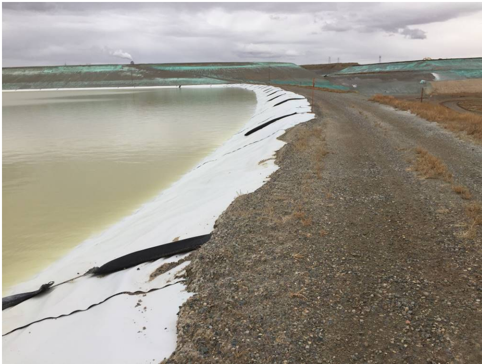
20191120 – IMG_6688 The upstream slope of the South Embankment, facing west from the southwest corner.
