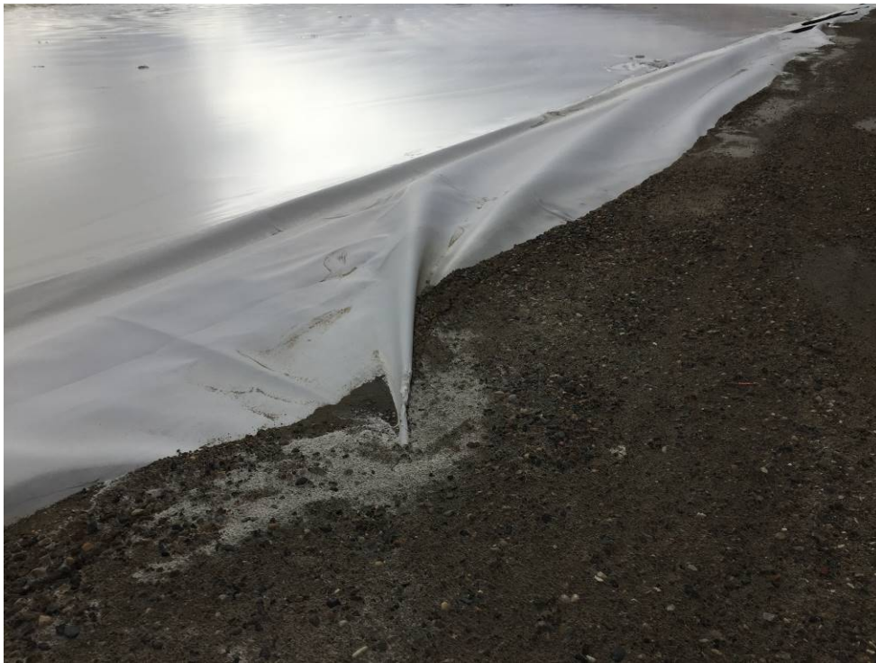
20191120 – IMG_6766 Small tears in the liner along the North Embankment repaired since the 2018 inspection.
