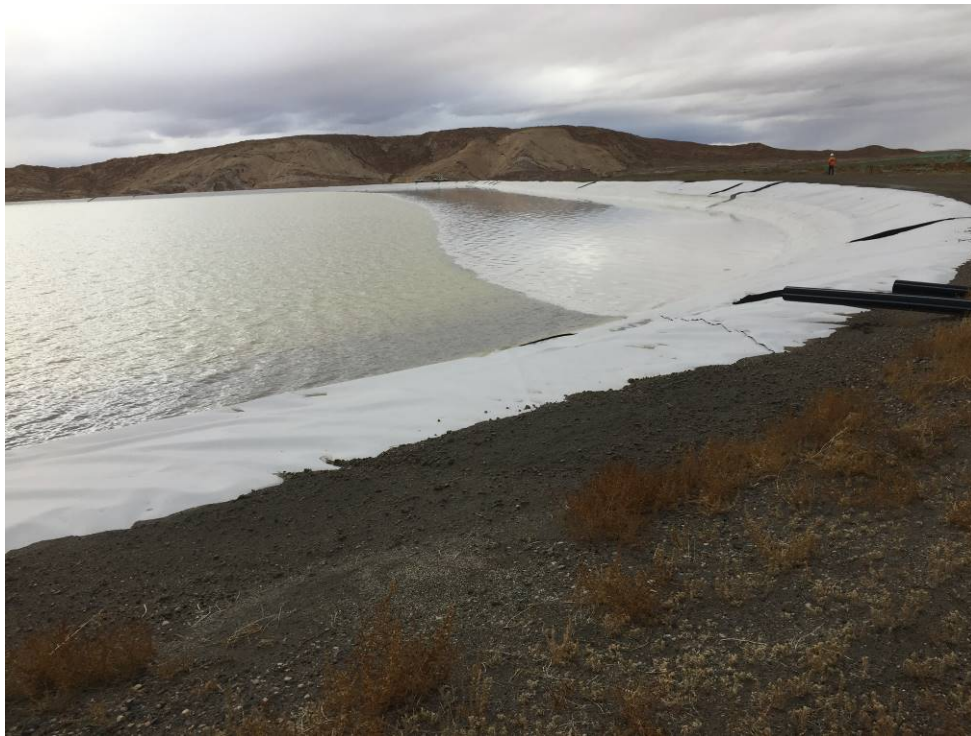
20191120 – IMG_6751 The upstream slope of the North Embankment, facing west from the East Embankment.
