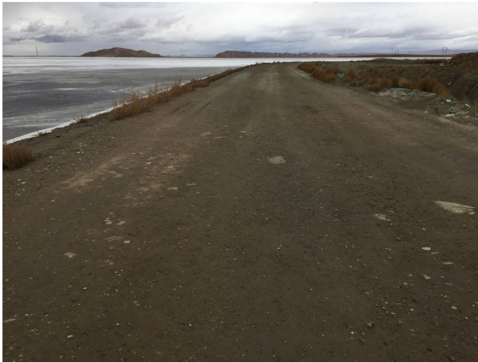
20191120 – IMG_6541 The crest of the East Embankment, facing north from the ash stockpile in the southeast corner.
