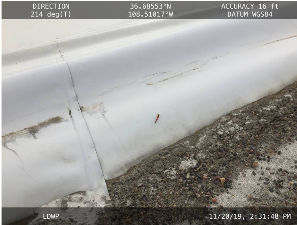
20191120 – IMG_6768 A hole in the liner along the North Embankment marked with a pin flag.
