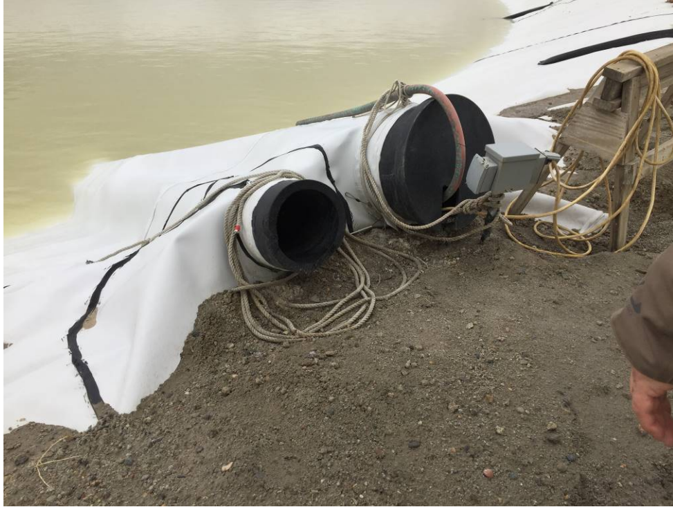
20191120 – IMG_6684 The HDPE pipes associated with the Interstitial Evacuation Pump.
