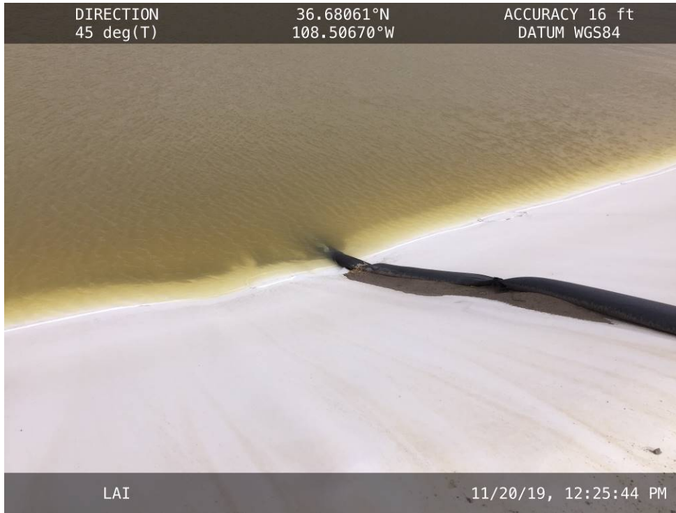
20191120 – IMG_6504 Uneven section of the upstream liner along the South Embankment.
