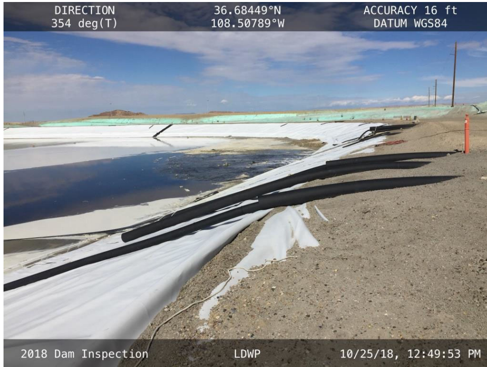
20181025 – IMG_1564 The liner pulling out of the anchor trench in the East Embankment.
