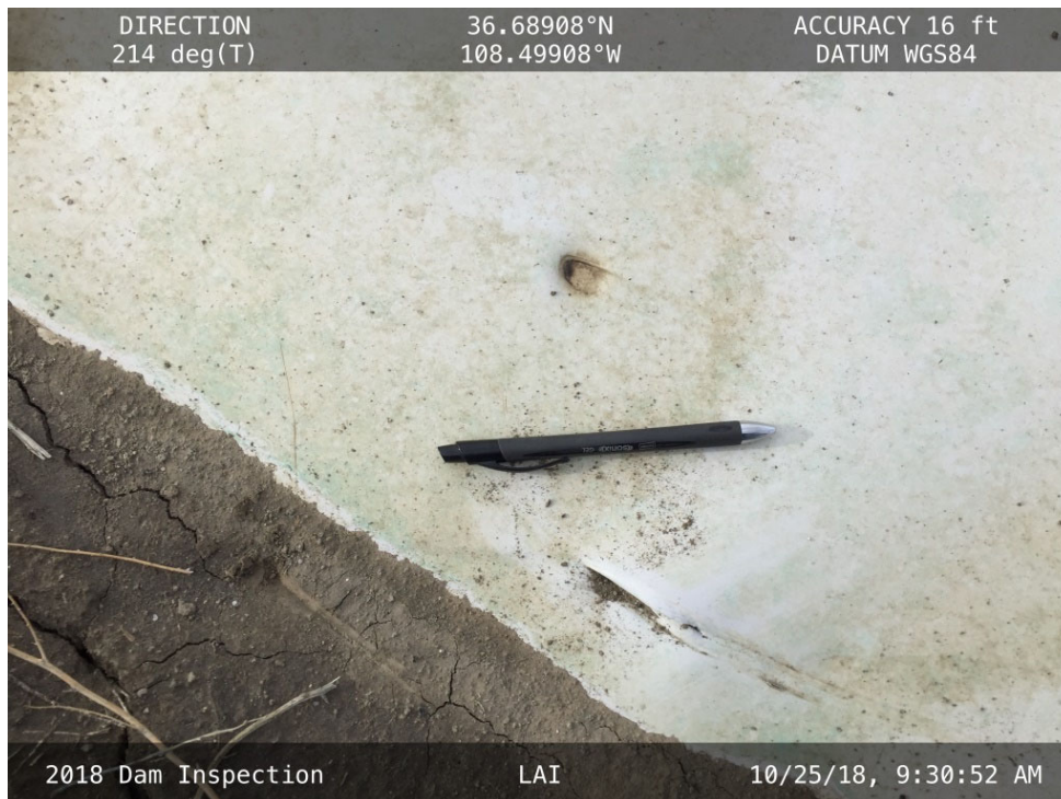
20181025 – IMG_1358 A small scratch and indentation in the liner along the East Embankment.
