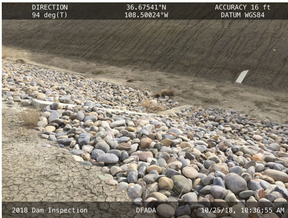
20181025 – IMG_1423 Sediment in the Stormwater Diversion Channel near the outlet.
