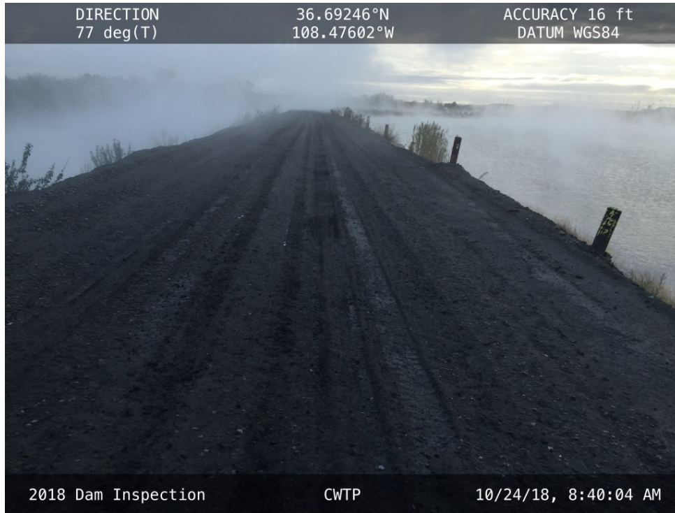
20181024 – IMG_0908 The crest of the CWTP, facing east from the West Abutment.
