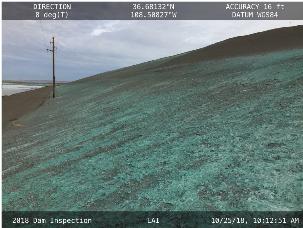
20181025 – IMG_1388 The downstream slope of the West Embankment, facing north along the toe.
