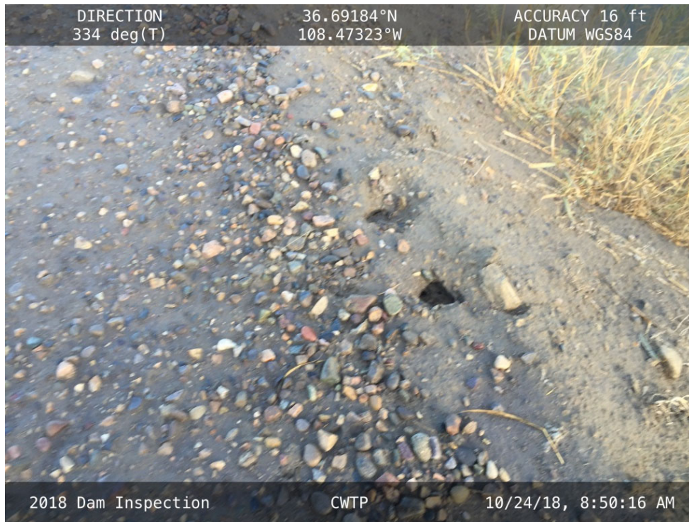
20181024 – IMG_0931 Erosion holes along the downstream shoulder of the crest.
