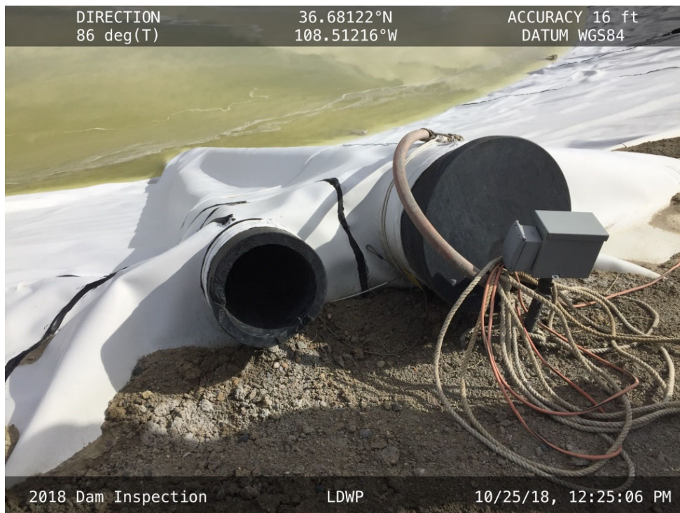
20181025 – IMG_1471 The HDPE pipes associated with the Interstitial Evacuation Pump.
