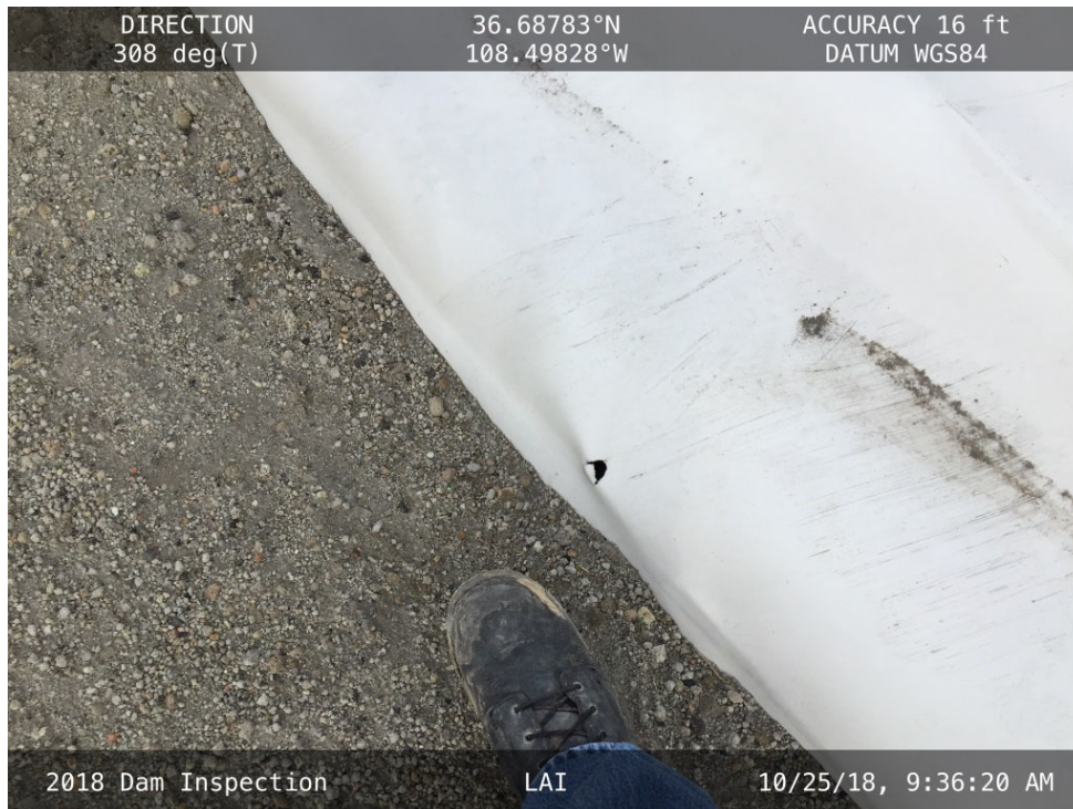
20181025 – IMG_1375 A small hole in the liner near the V-ditch at the East Embankment.
