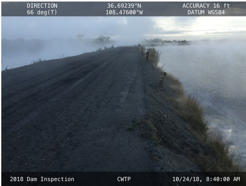
20181024 – IMG_0907 The crest and upstream slope of the CWTP, facing east from the West Abutment.
