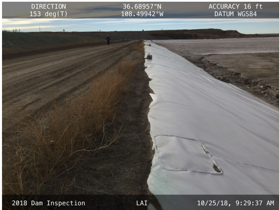
20181025 – IMG_1357 The crest and upstream slope of the East Embankment, facing southeast.
