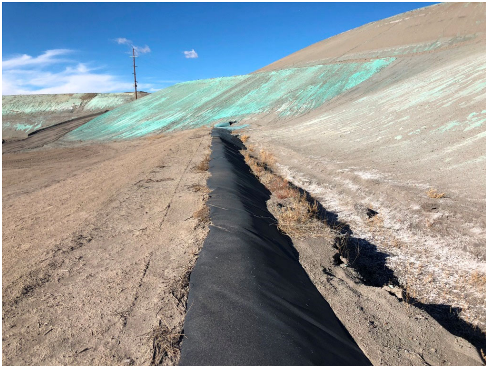
20181024 – IMG_0937 Area of additional erosion along the western toe of Cell 3 north of IMG_0933, facing north.
