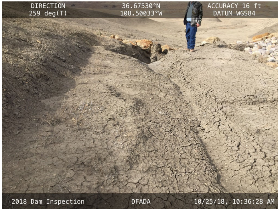
20181025 – IMG_1422 Erosion at the Stormwater Diversion Channel outlet, facing west.
