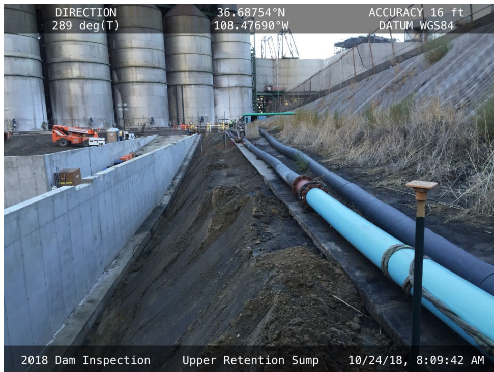
20181024 – IMG_0886 The north side of the Upper Retention Sump footprint, facing west.
