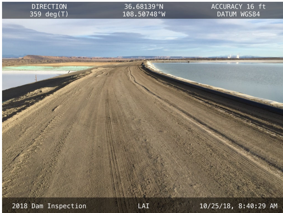
20181025 – IMG_1255 The crest of the West Embankment, facing north from the Southwest Corner.
