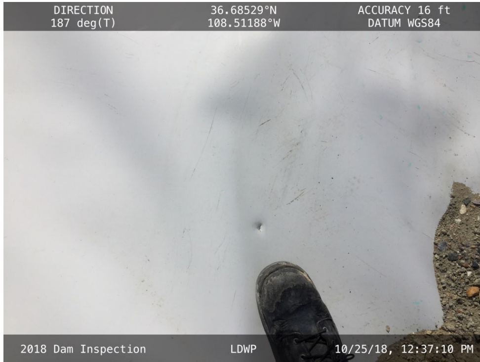
20181025 – IMG_1521 A shallow dent in the liner in the northwest corner of the LDWP.
