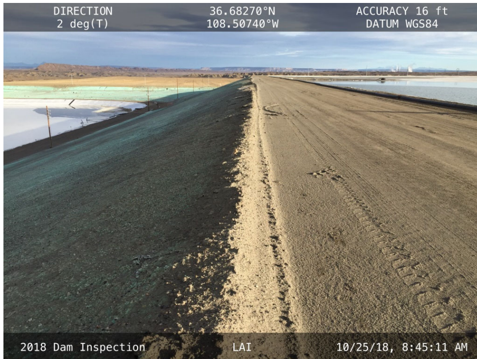
20181025 – IMG_1267 The downstream slope and crest of the West Embankment, facing north.
