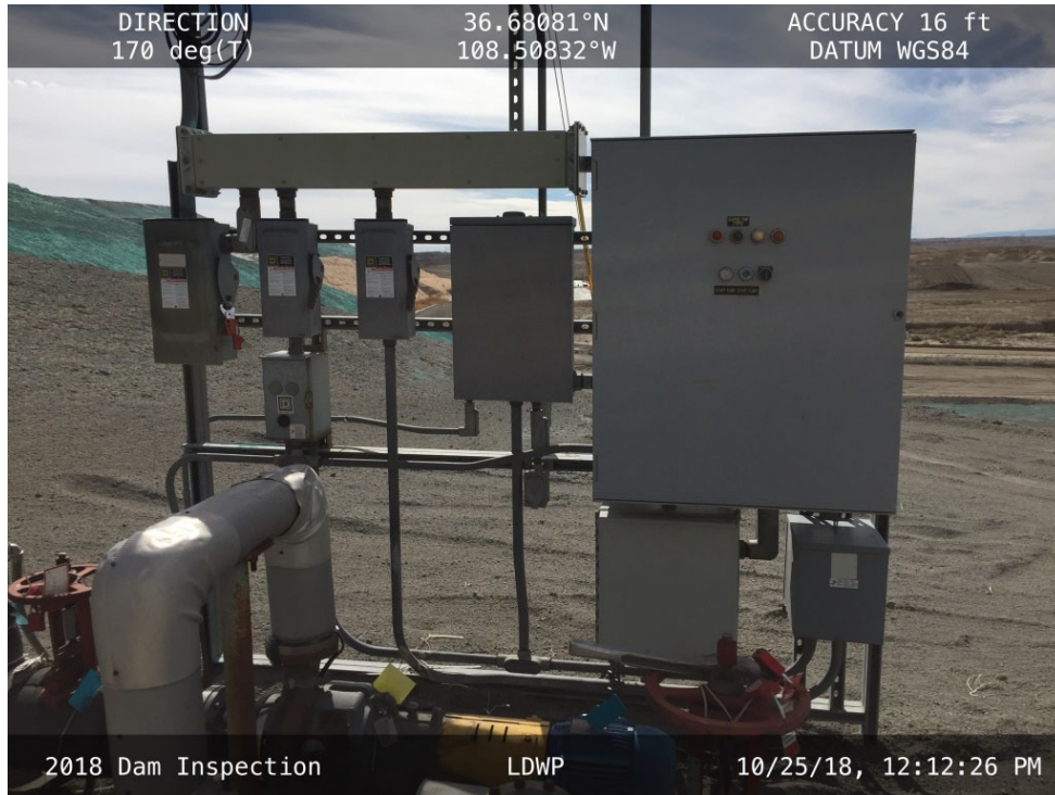
20181025 – IMG_1445 The Deadpool Sump control panels (no longer in use).
