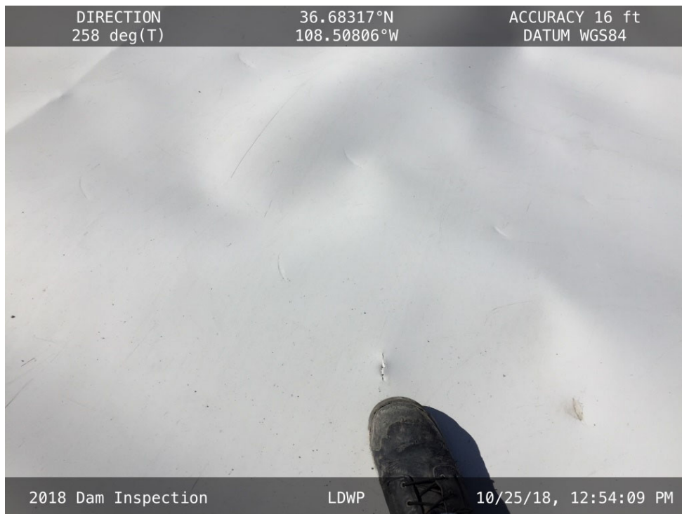
20181025 – IMG_1572 Shallow dents in the liner along the upstream slope of the East Embankment.
