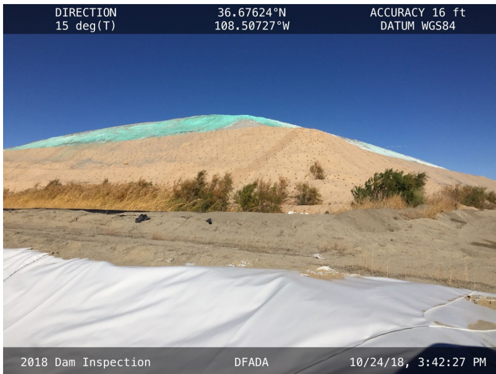
20181024 – IMG_1136 Woody vegetation growing through the Pyramat in the southwest corner of Cell 1.
