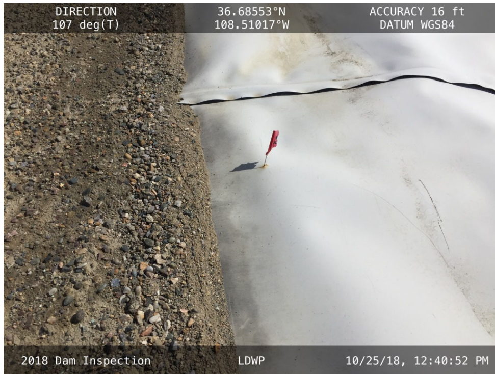
20181025 – IMG_1529 A hole in the liner along the North Embankment already marked with a pin flag.
