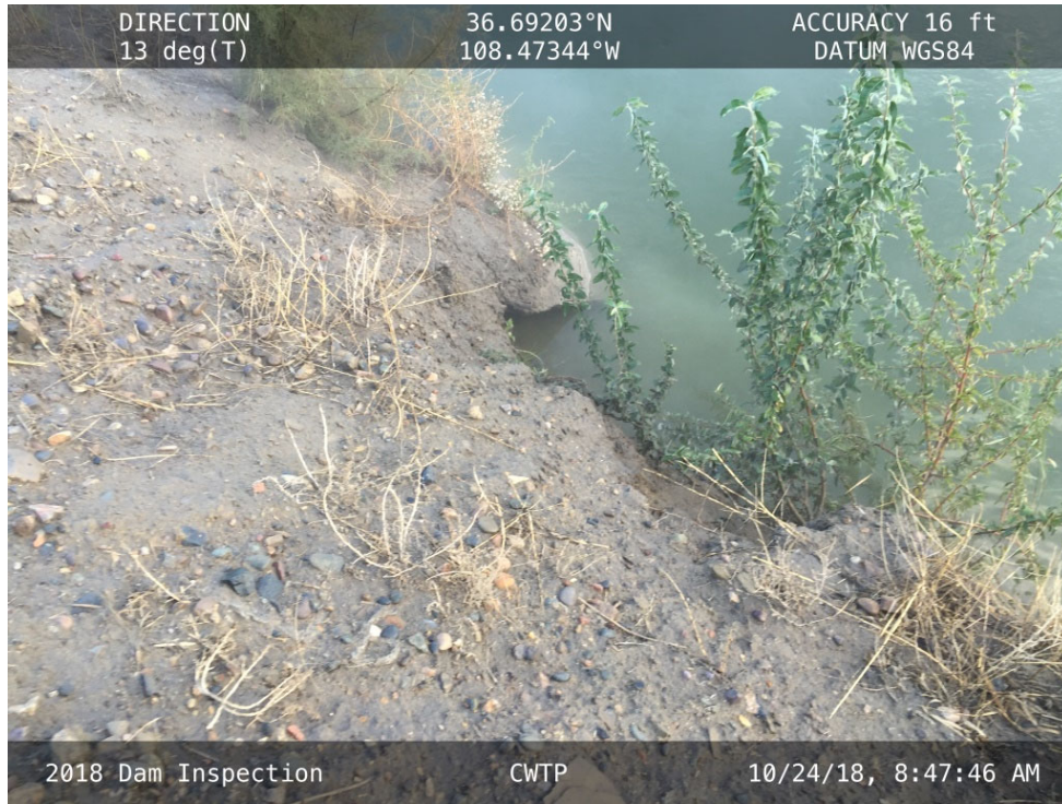
20181024 – IMG_0927 Erosion at the waterline along the downstream slope.
