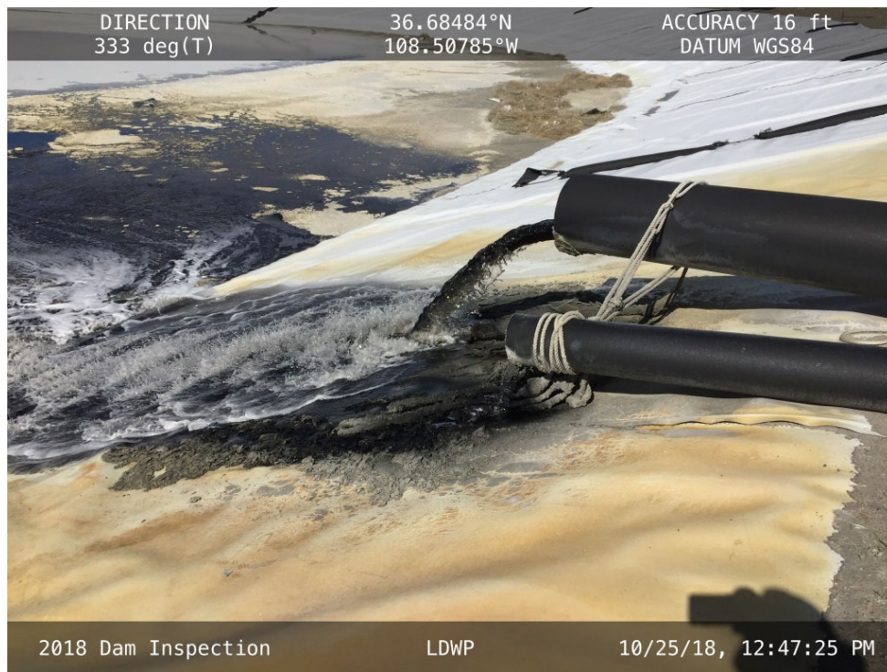
20181025 – IMG_1547 The 8-inch and 16-inch HDPE outlet pipes conveying decant water from the LAI.
