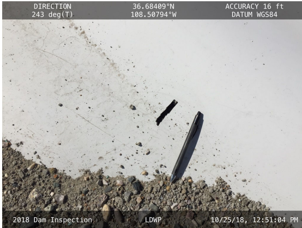
20181025 – IMG_1571 A tear in the liner along the East Embankment (also observed during the 2017 inspection).
