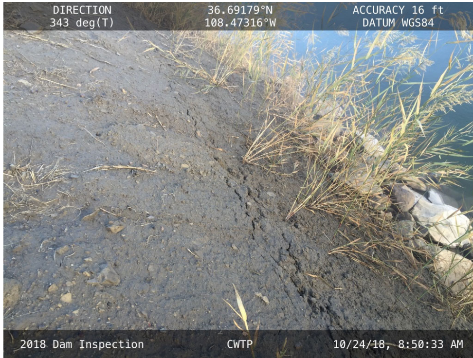
20181024 – IMG_0933 Longitudinal cracks on the downstream slope of the CWTP embankment.
