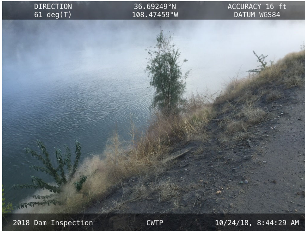
20181024 – IMG_0921 Woody vegetation to be removed from the downstream slope.
