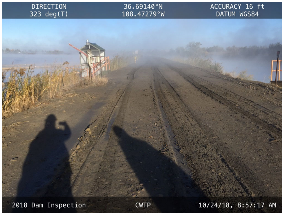
20181024 – IMG_0947 The crest of the CWTP embankment, facing northwest from the South Abutment.
