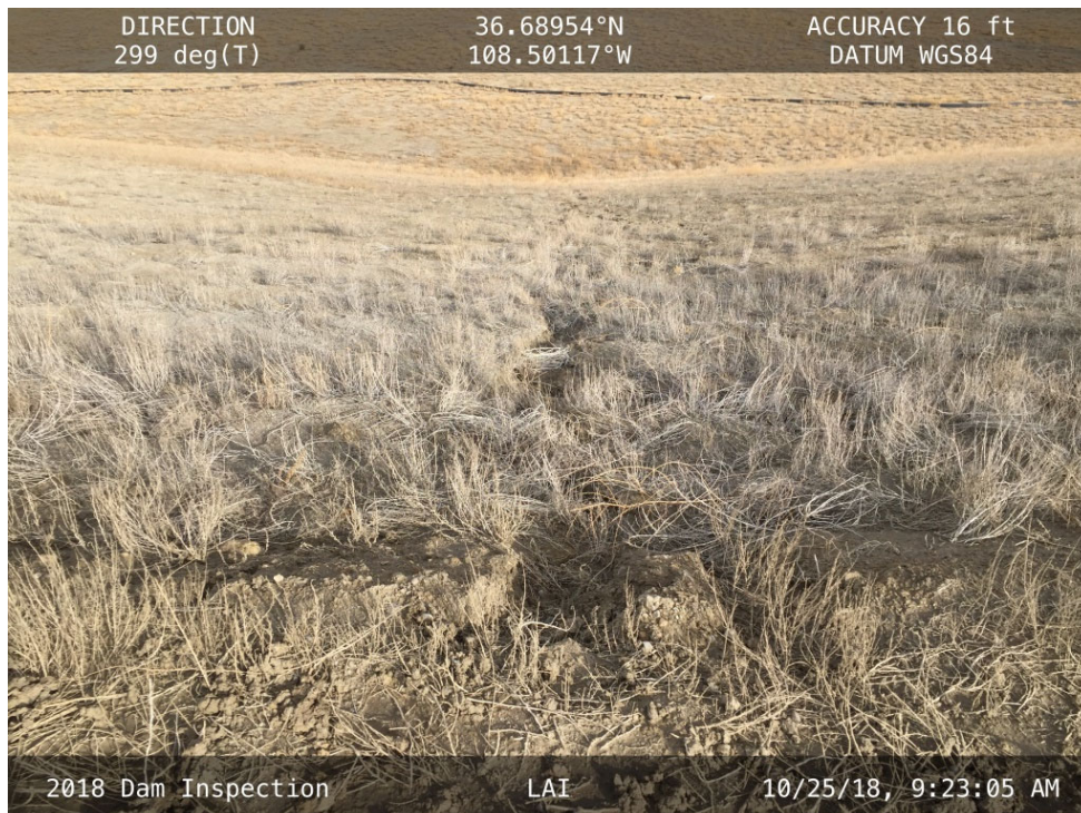
20181025 – IMG_1338 Shallow erosion rill in the groin of the Northwest Embankment along the north end of the LAI.
