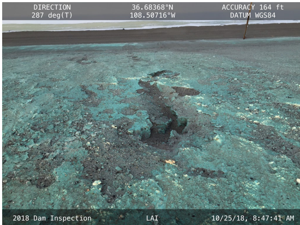
20181025 – IMG_1269 Minor erosion on the downstream slope of the West Embankment.
