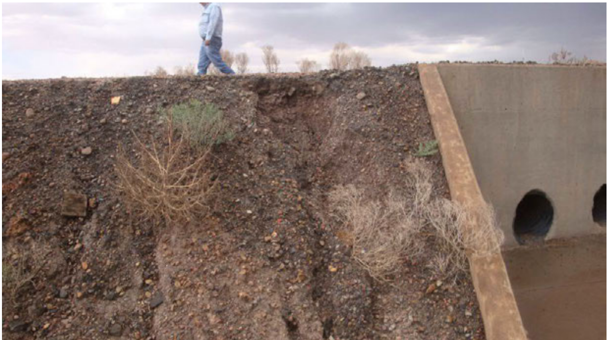
20151016 – Photo 4 Downstream slope. Minor erosion rills.
