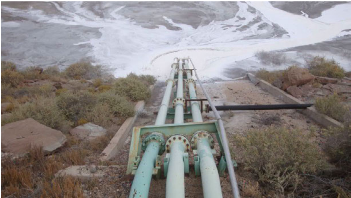
20151016 – Photo 12 Upstream slope. FGD/ash lines. Discharge to impoundment.
