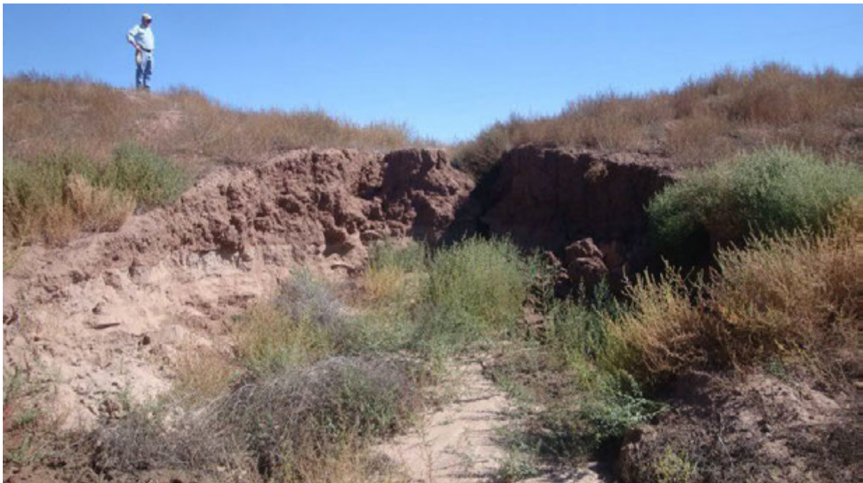
20151016 – Photo 12 Run-on detention basin. Head-cutting at inlet.
