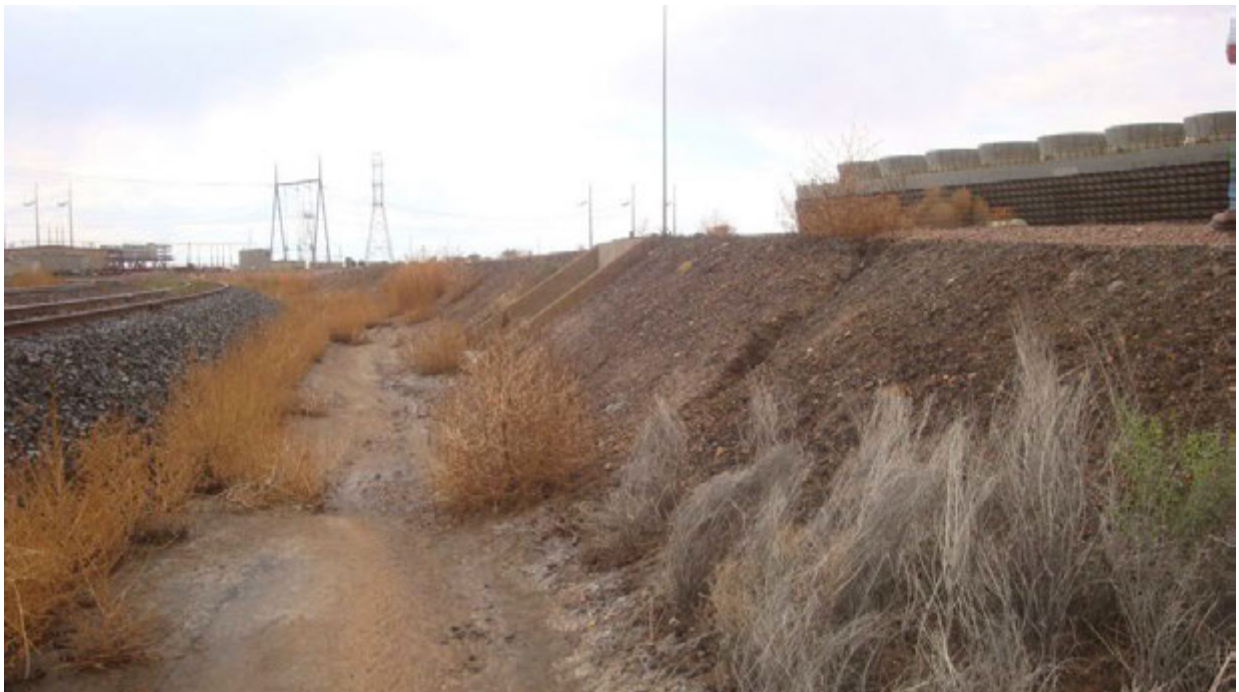
20151016 – Photo 2 West Embankment. Downstream slope. Minor erosion rills.
