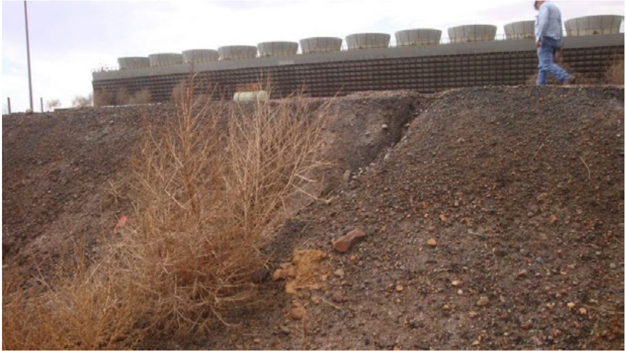
20151016 – Photo 5 Downstream slope. Minor erosion rills.
