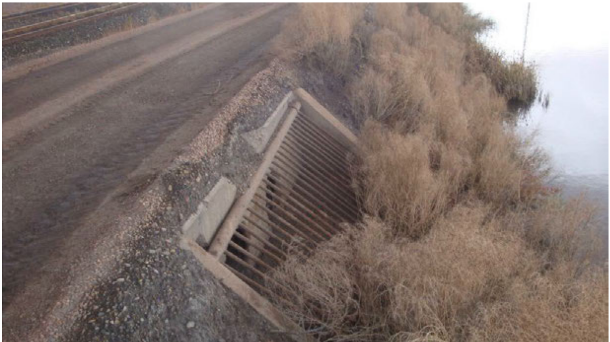
20151016 – Photo 11 Upstream slope. Gated inlet, partially blocked by vegetation.
