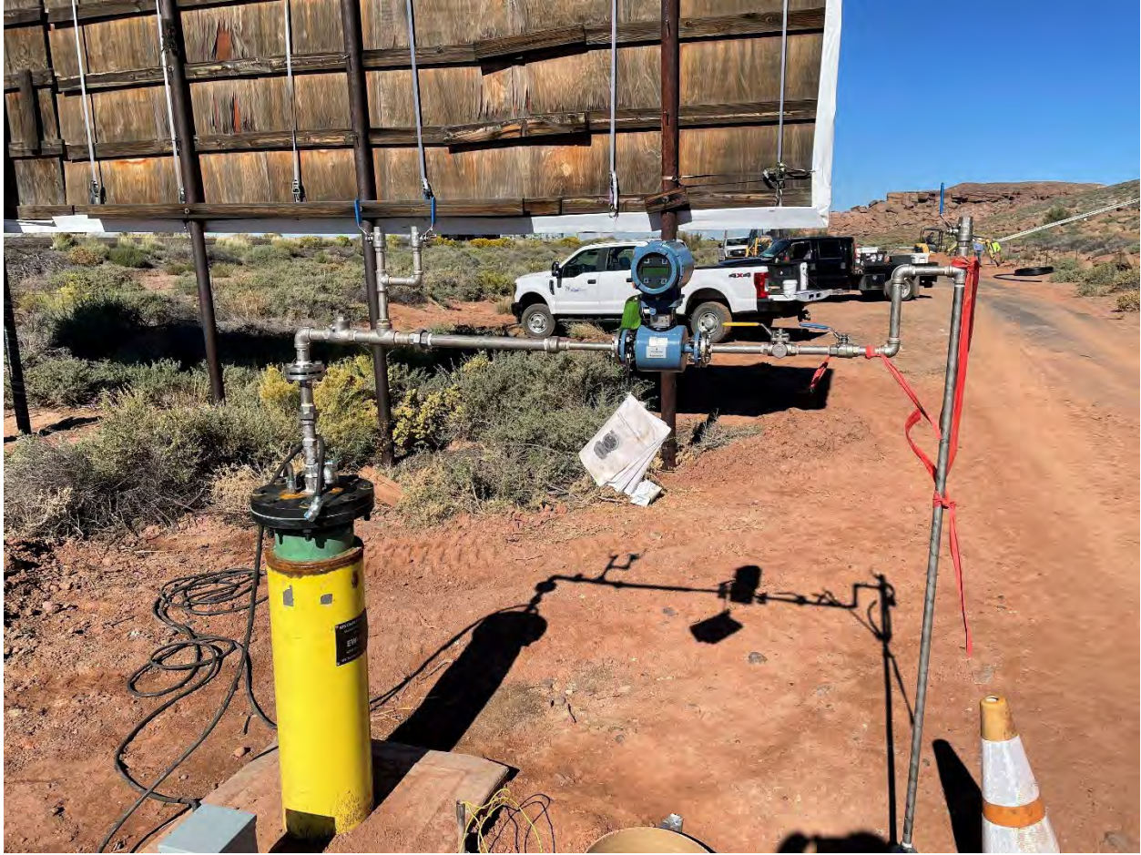
Figure 5: EW-02 piping, No Insulation
