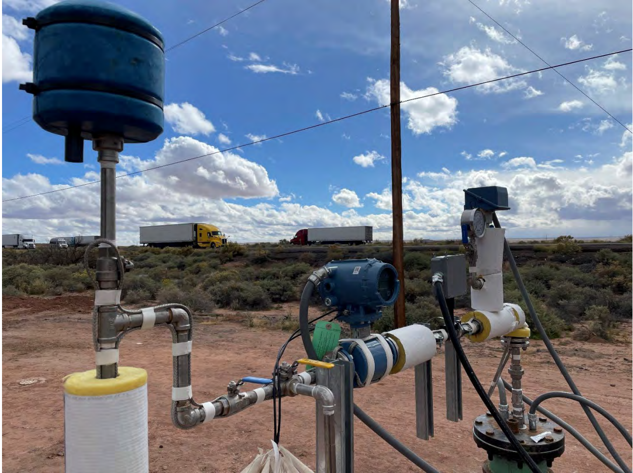
Figure 7: EW-04 piping, Some Insulation
