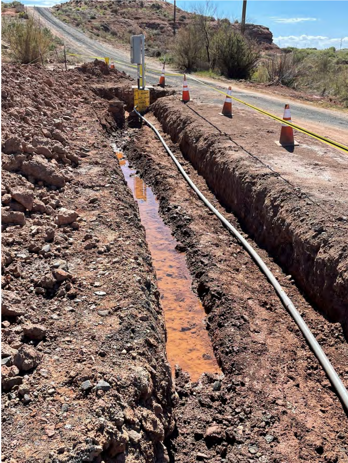
Figure 3: Flooded Trench looking east towards EW-04
