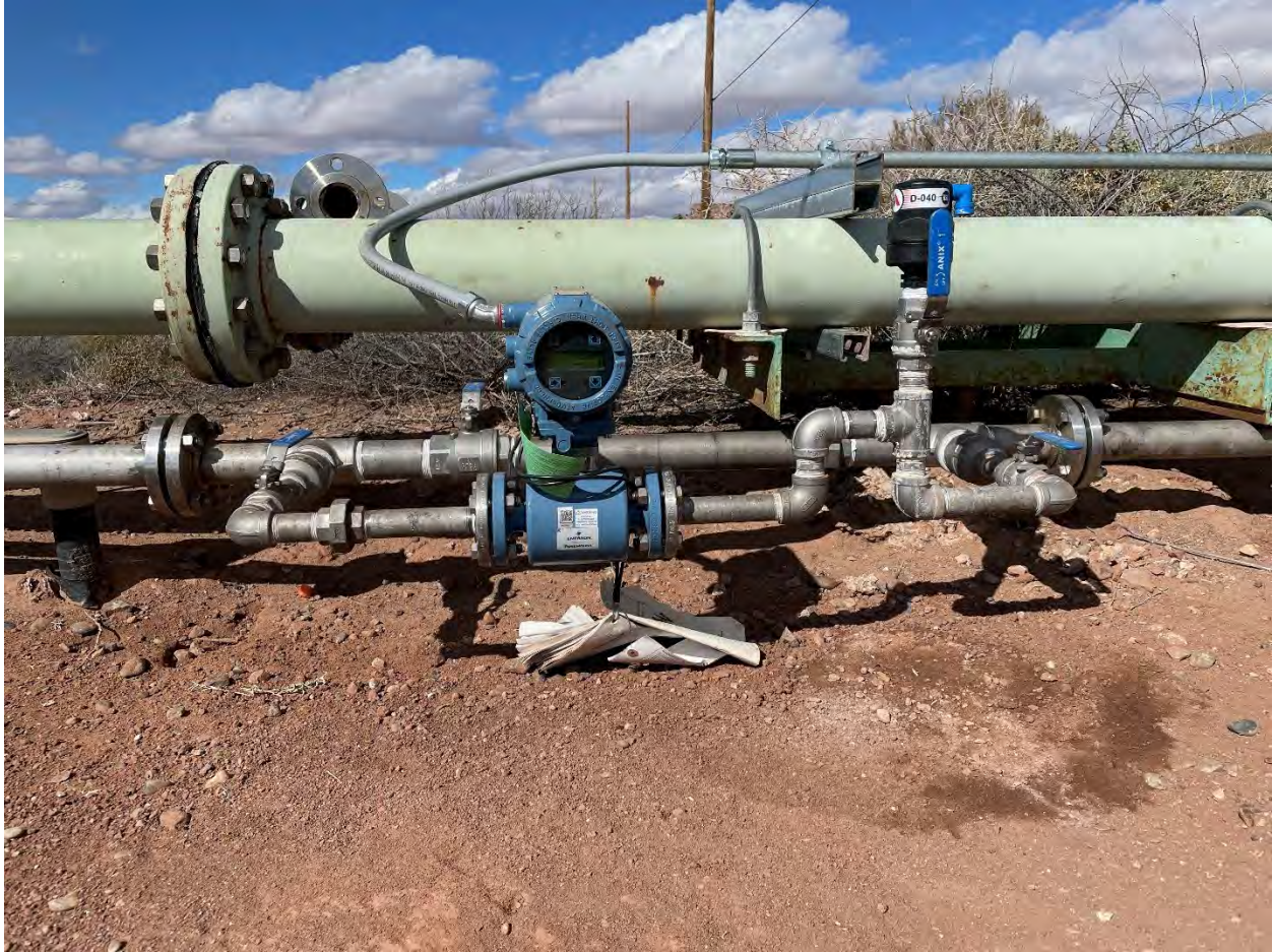
Figure 9: Hunt flow meter No Insulation
