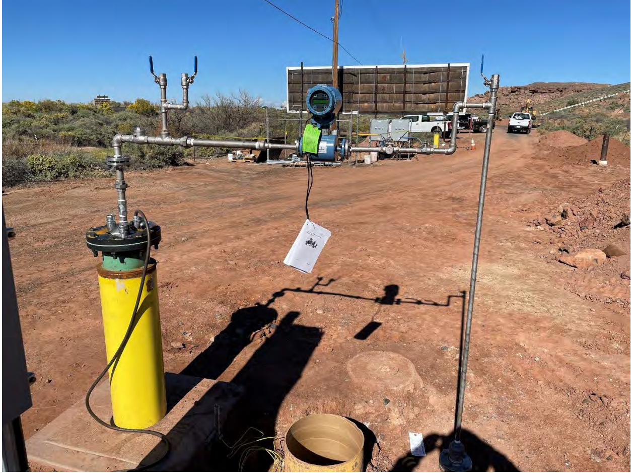
Figure 6: EW-03 piping, No Insulation
