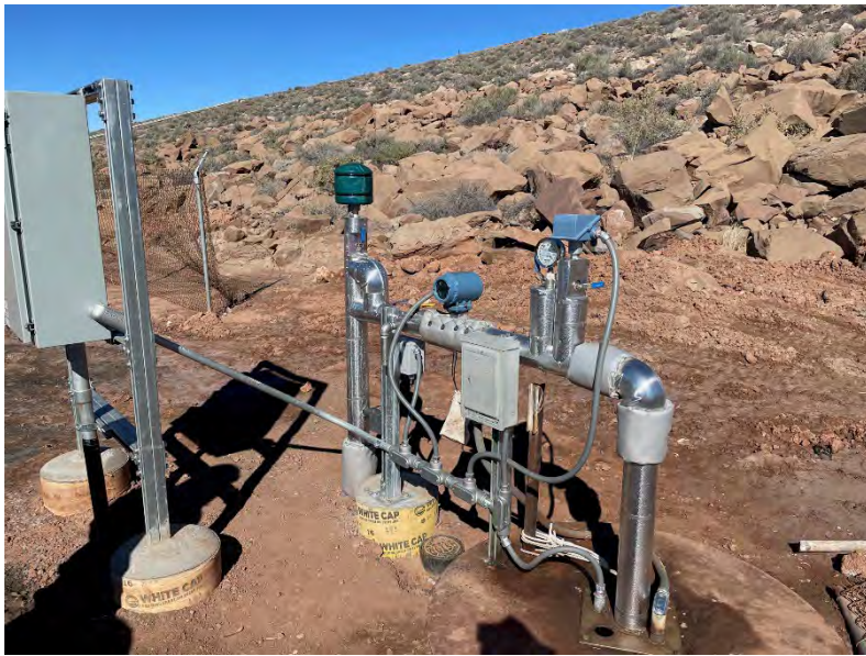
Leaking at GSX-3
