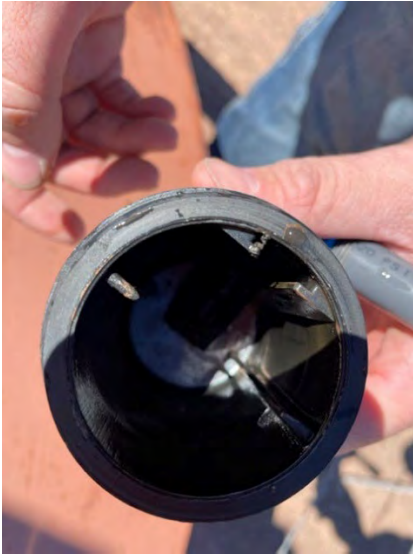
cleaned out ARV
