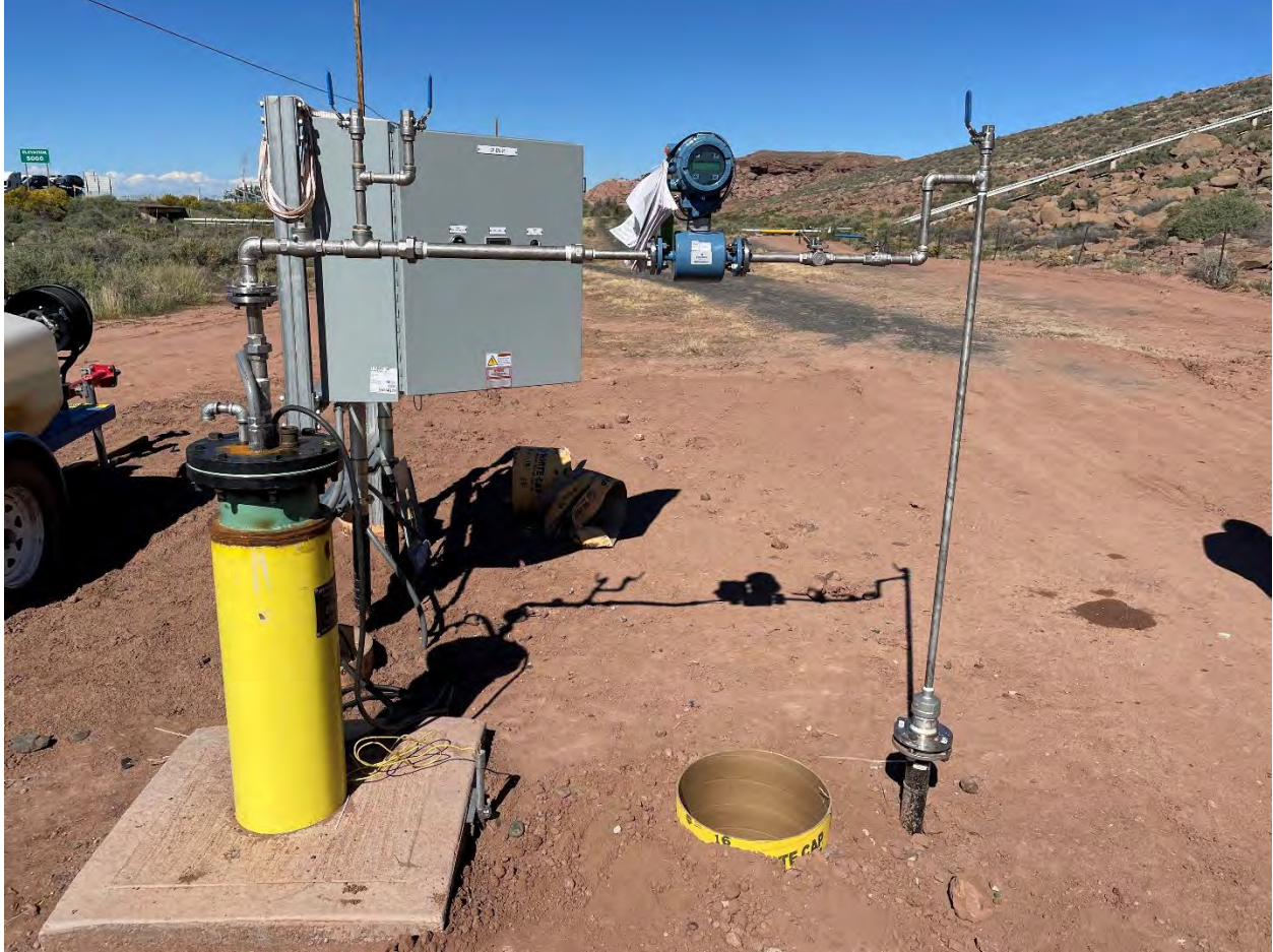
Figure 4: EW-01 piping, No Insulation
