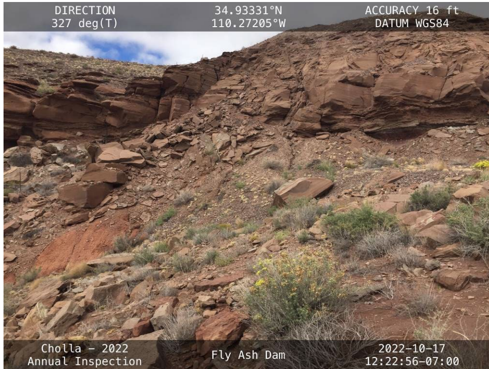
20221017 – IMG_3459 Erosion on the downstream side of the Right Abutment contact.
