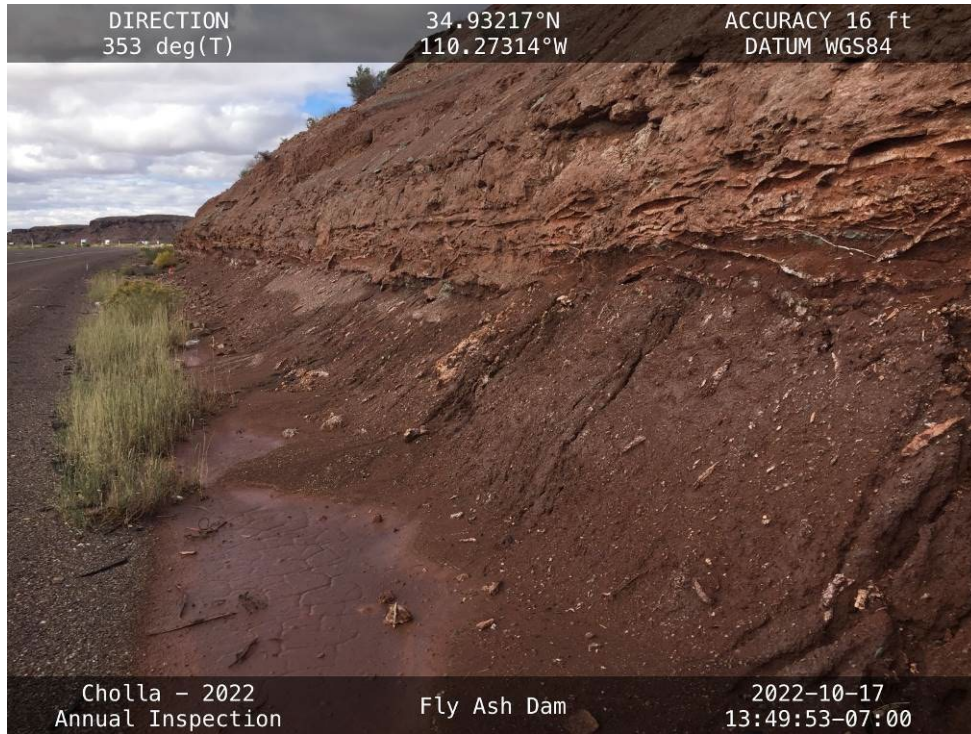
20221017 - IMG_3554 The I-40 seep.
