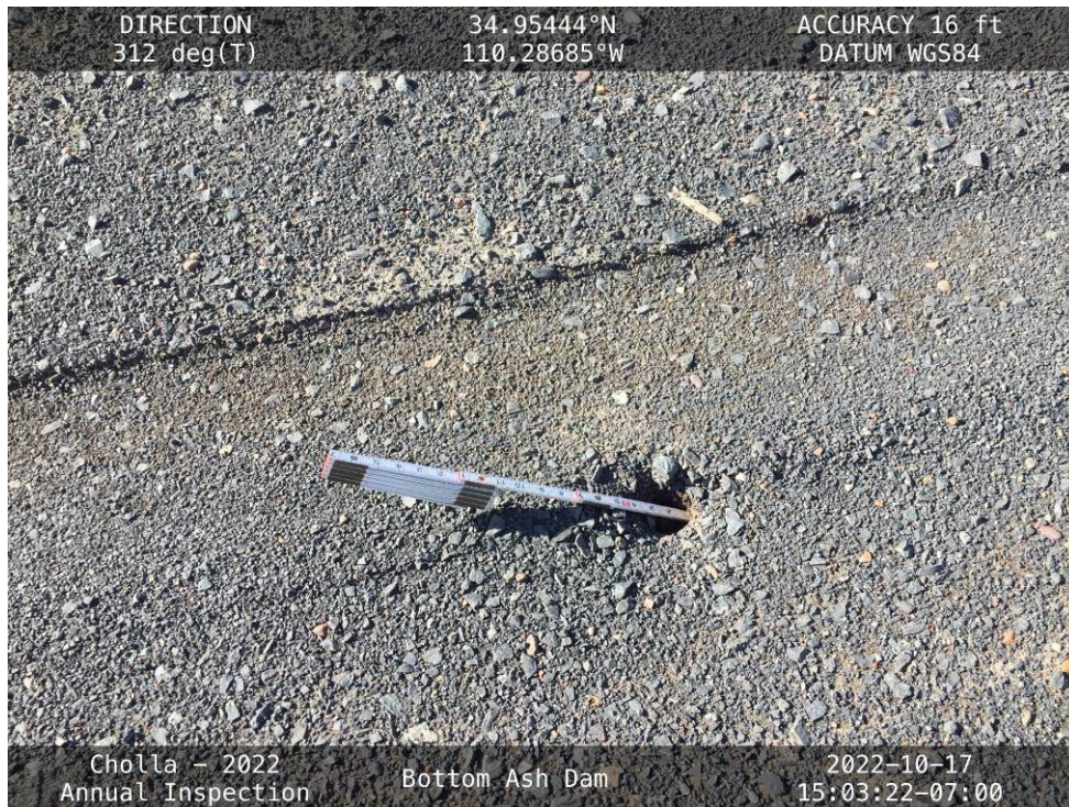
20221017 – IMG_3629 A hole in the crest of the East Embankment, approximately 4 inches deep.
