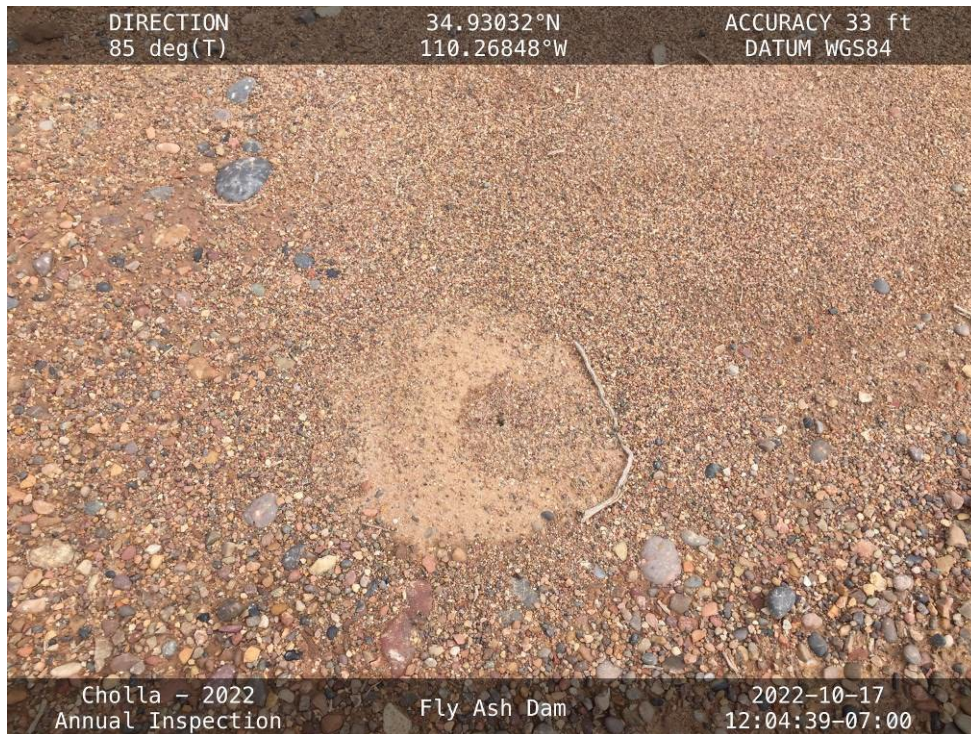
20221017 – IMG_3449 An ant hill on the embankment crest near the inlet lines.
