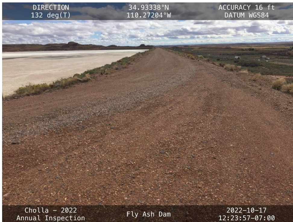
20221017 – IMG_3464 The crest of the Fly Ash Dam, facing southeast from the Right Abutment.
