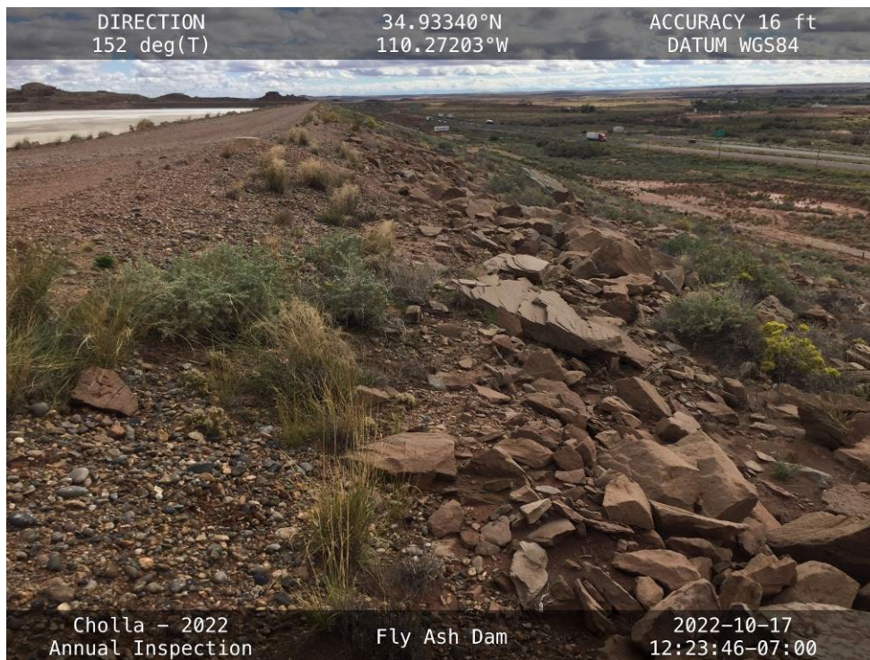
20221017 – IMG_3462 The downstream slope of the Fly Ash Dam, facing southeast from the Right Abutment.
