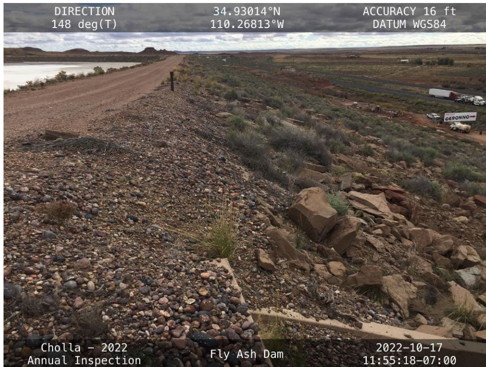
20221017 – IMG_3437 The downstream slope along the southern half of the West Embankment, facing southeast.
