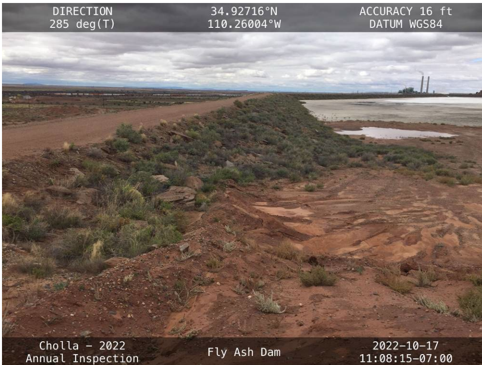
20221017 – IMG_3390 The upstream slope of the South Embankment, facing west from the Left Abutment.
