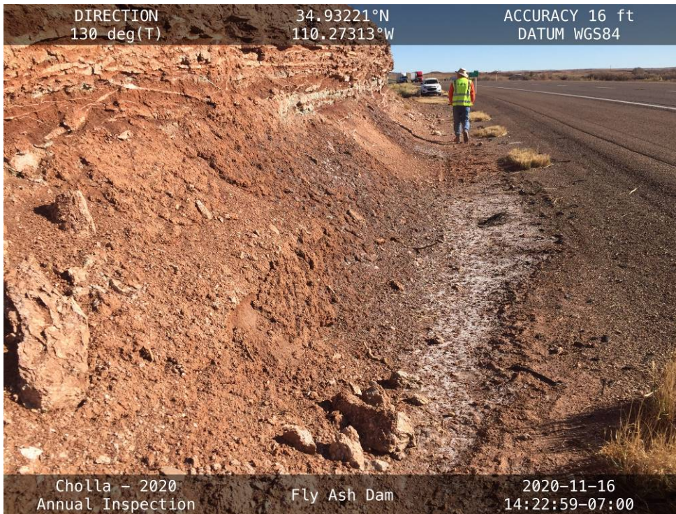
20201116 – IMG_2584 The I-40 seep.
