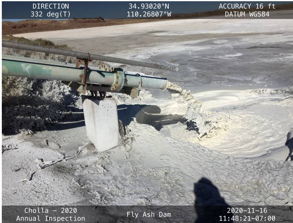
20201116 – IMG_2299 The inlet pipe depositing CCR into the impoundment.
