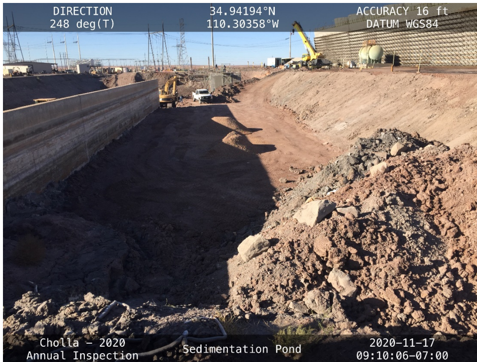
20201117 – IMG_2933 The North Cell, facing southwest from the east side. CCR stockpiled on the right side of the image.
