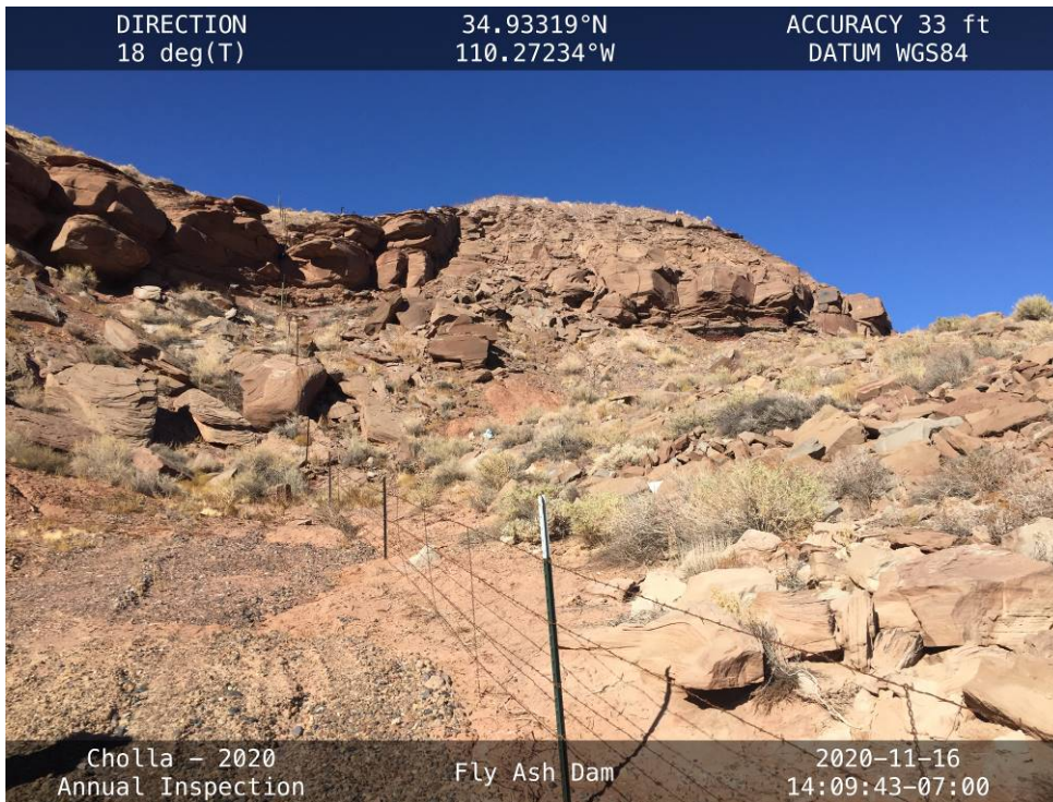
20201116 – IMG_2560 The Northwest Abutment contact and area of historic erosion, facing north from the toe.
