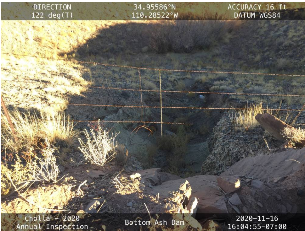
20201116 – IMG_2748 An erosion gully on the downstream slope along the northern half of the East Embankment.
