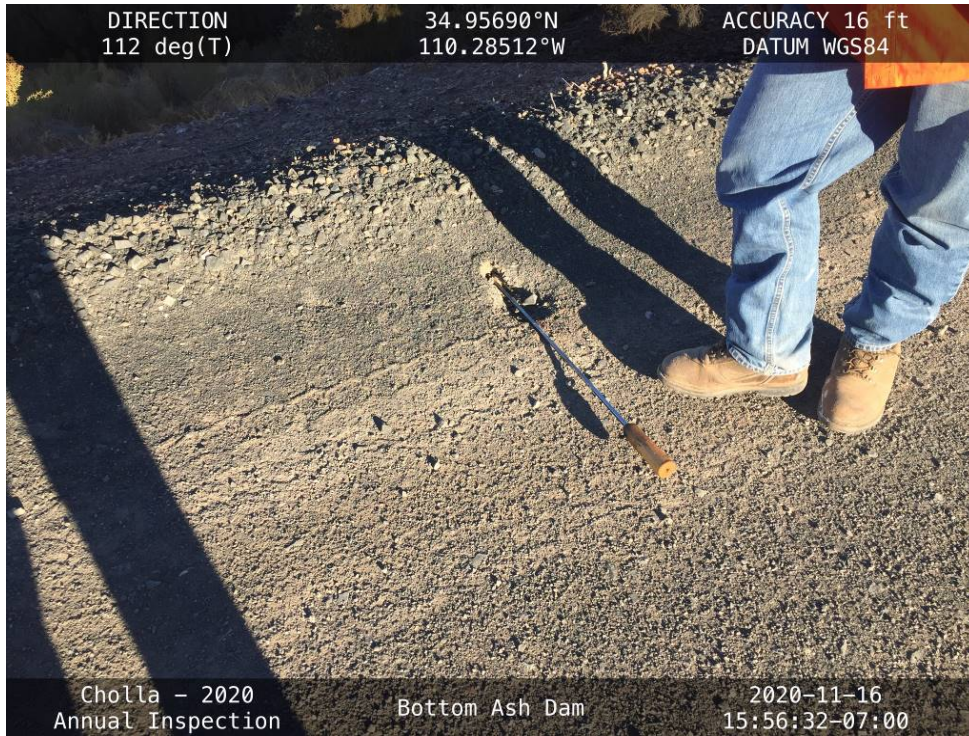
20201116 – IMG_2718 A hole on the upstream shoulder of the East Embankment.
