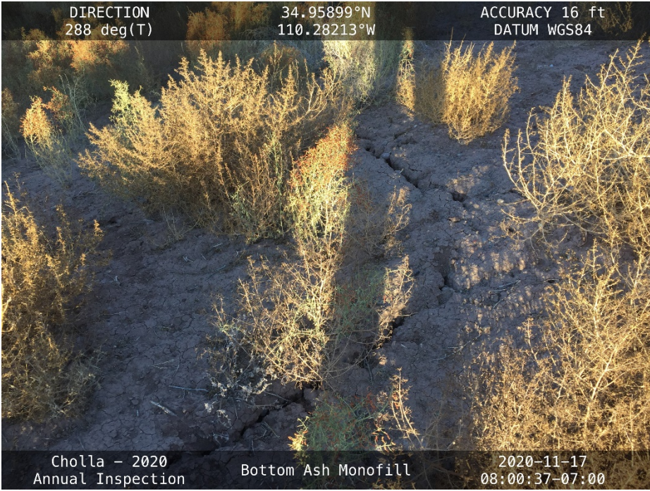
20201117 – IMG_2866 An incipient erosion rill where erosion was previously repaired in the northeast corner of the Stormwater Detention Basin.
