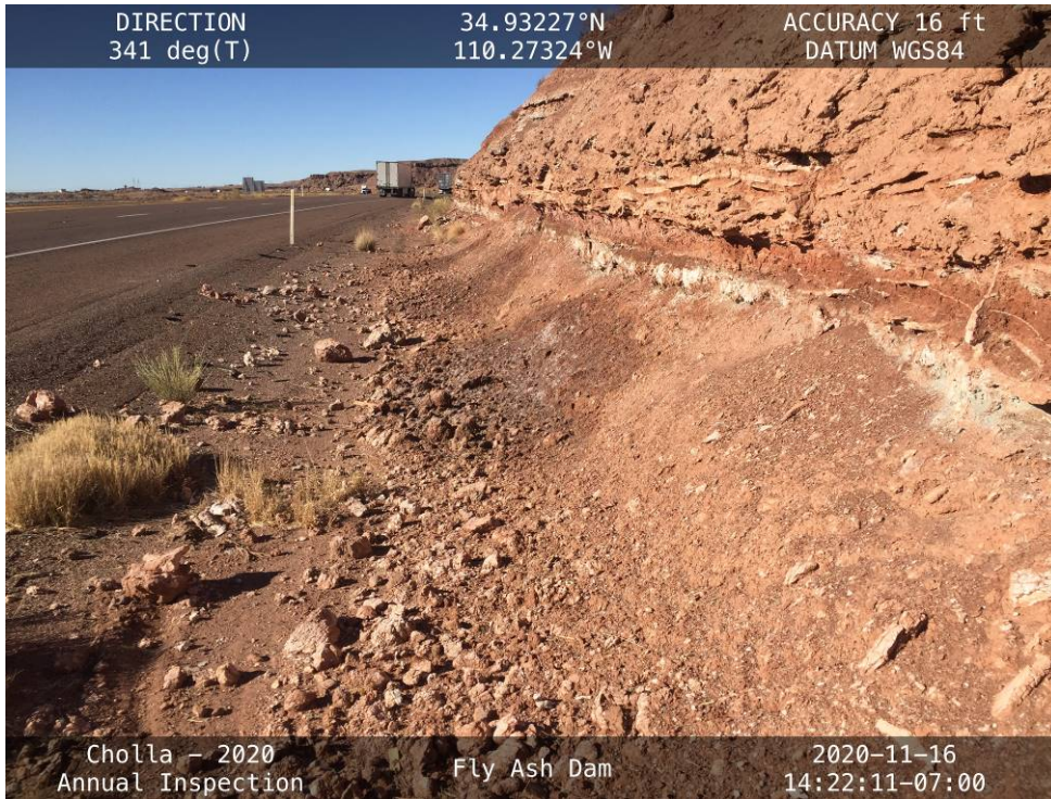
20201116 – IMG_2580 The I-40 seep.
