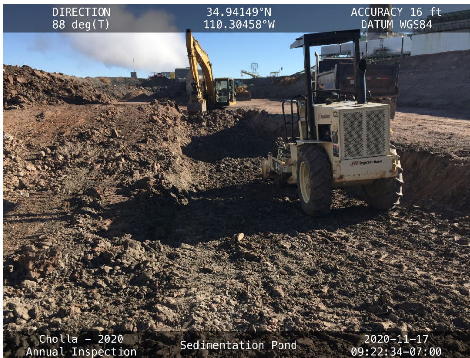
20201117 – IMG_2967 The Sedi Tank contractor removing the Divider Wall and compacting structural fill in the void.
