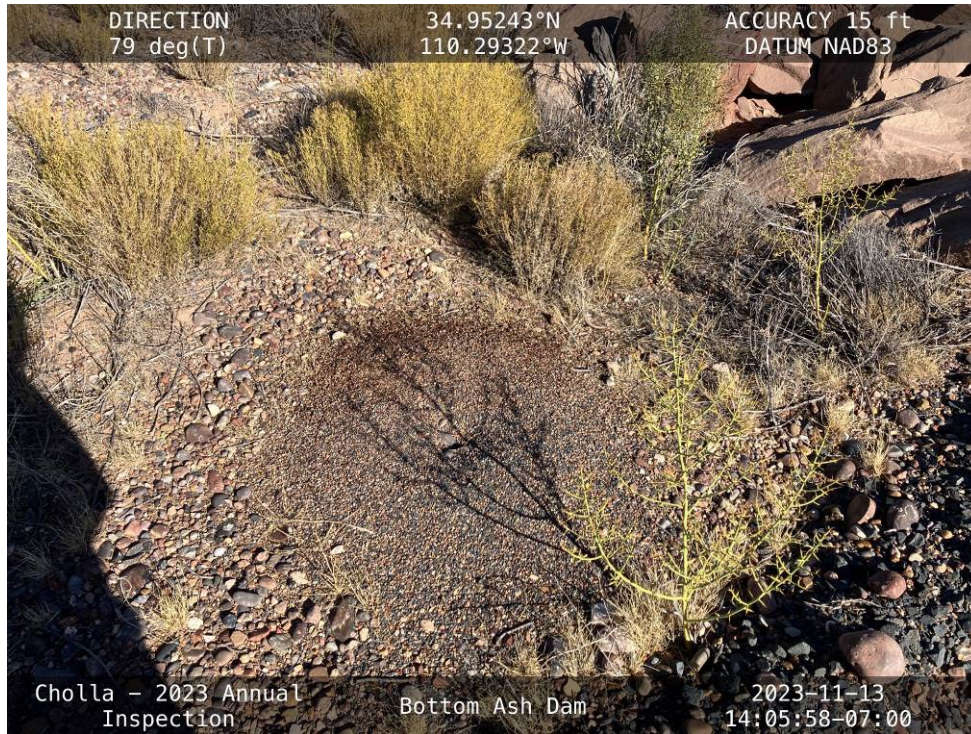
20231113 – IMG_1610 An ant hill on the upstream shoulder at the Right Abutment.
