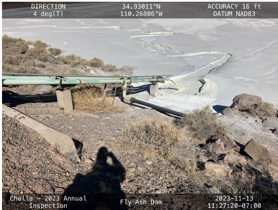
20231113 – IMG_1452 The inlet pipe depositing CCR into the impoundment.
