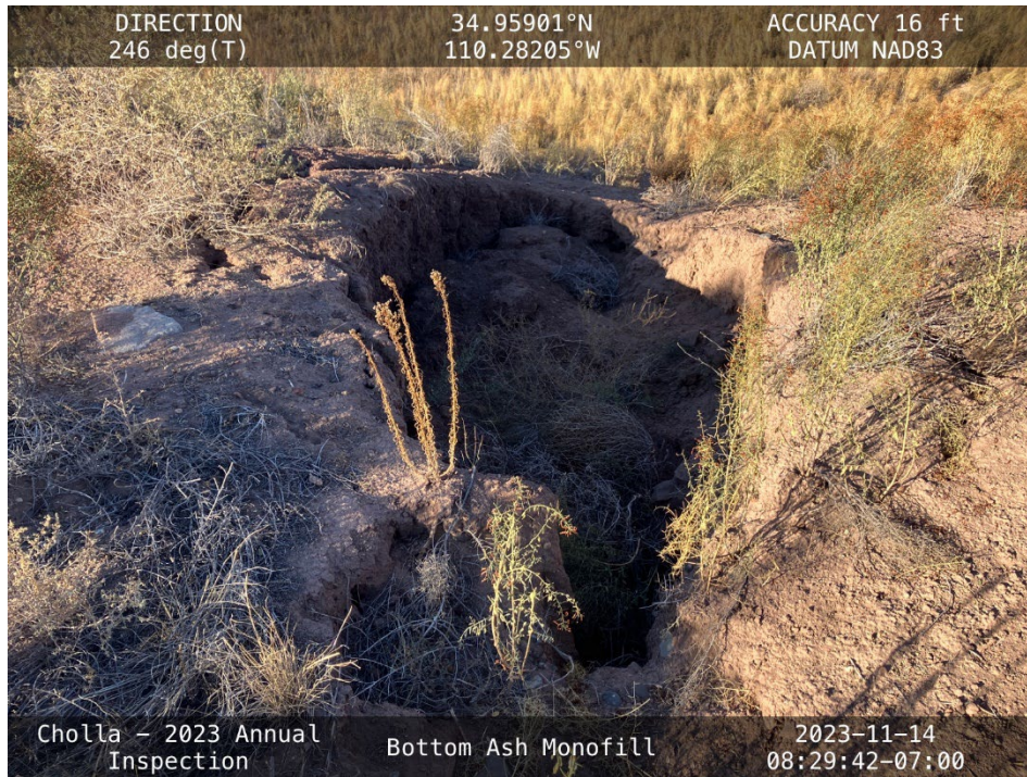
20231114 – IMG_1949 Erosion on the east side of the Stormwater Detention Basin.
