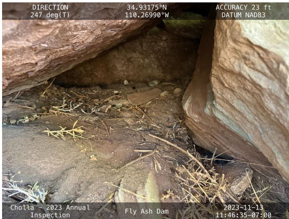
20231113 – IMG_1469 A 1.5-foot-deep gap formed as soil erodes away between riprap on the upstream slope.
