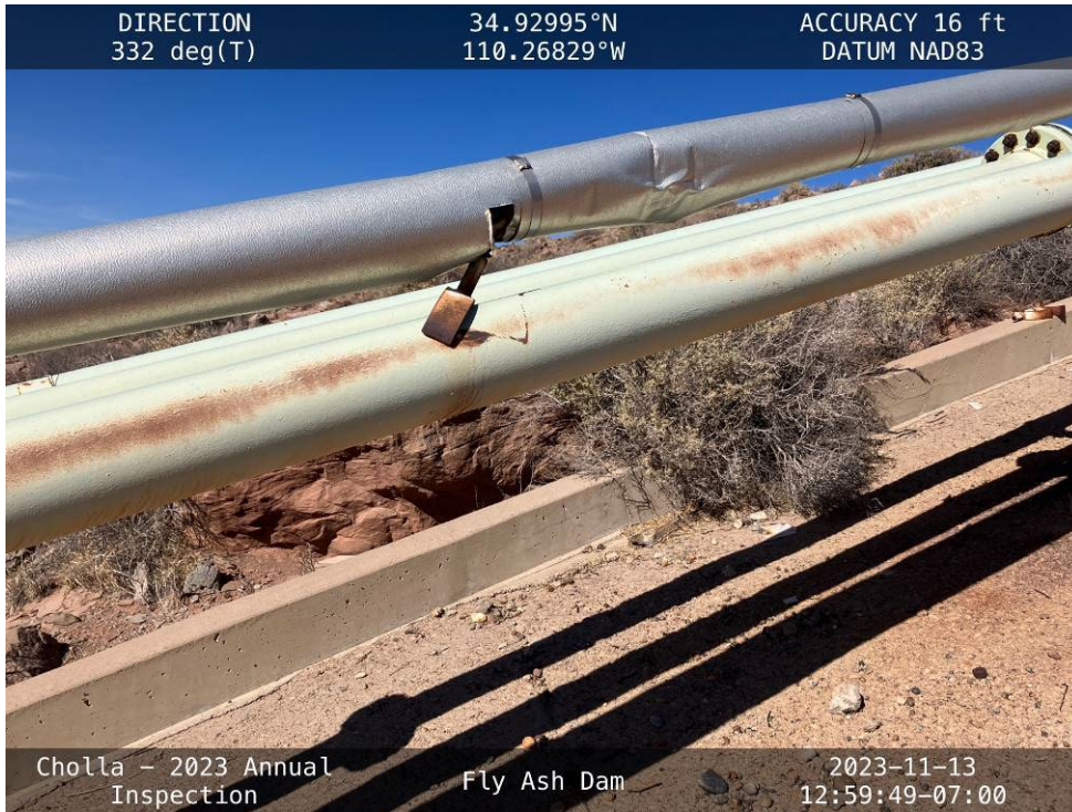
20231113 – IMG_1573 A broken pipe support along the inlet lines.
