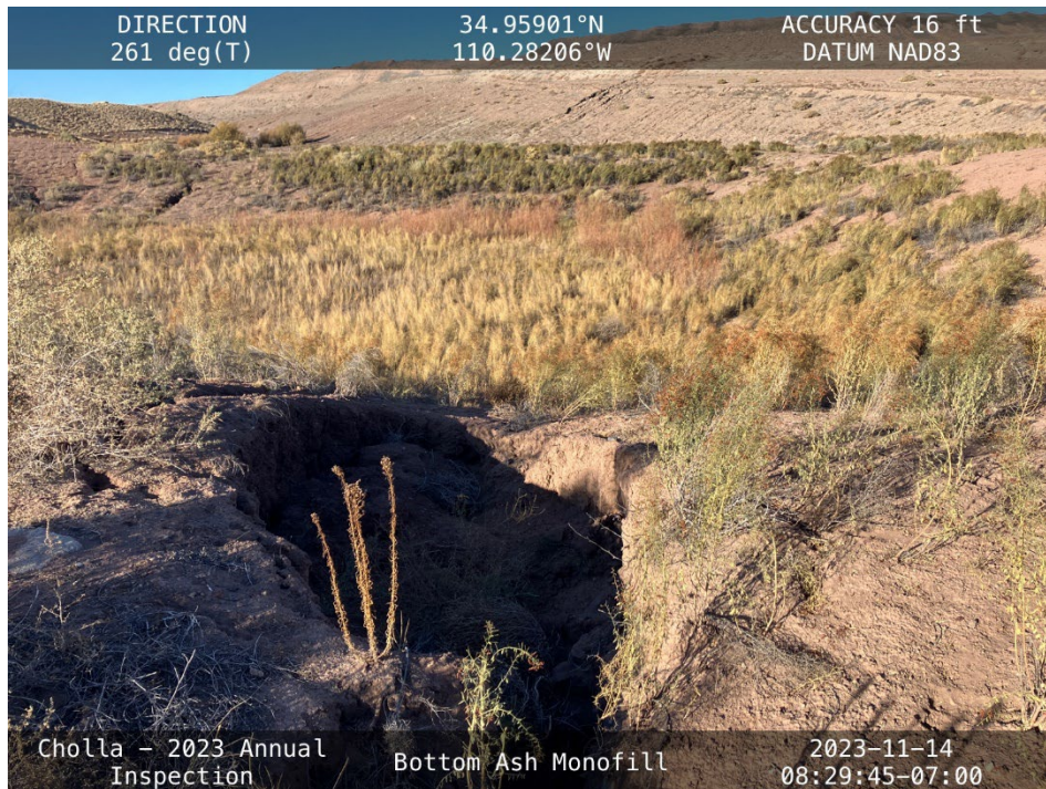
20231114 – IMG_1950 The west side of the Stormwater Detention Basin and the southern end of the BAM, facing west from the east side of the Stormwater Detention Basin.
