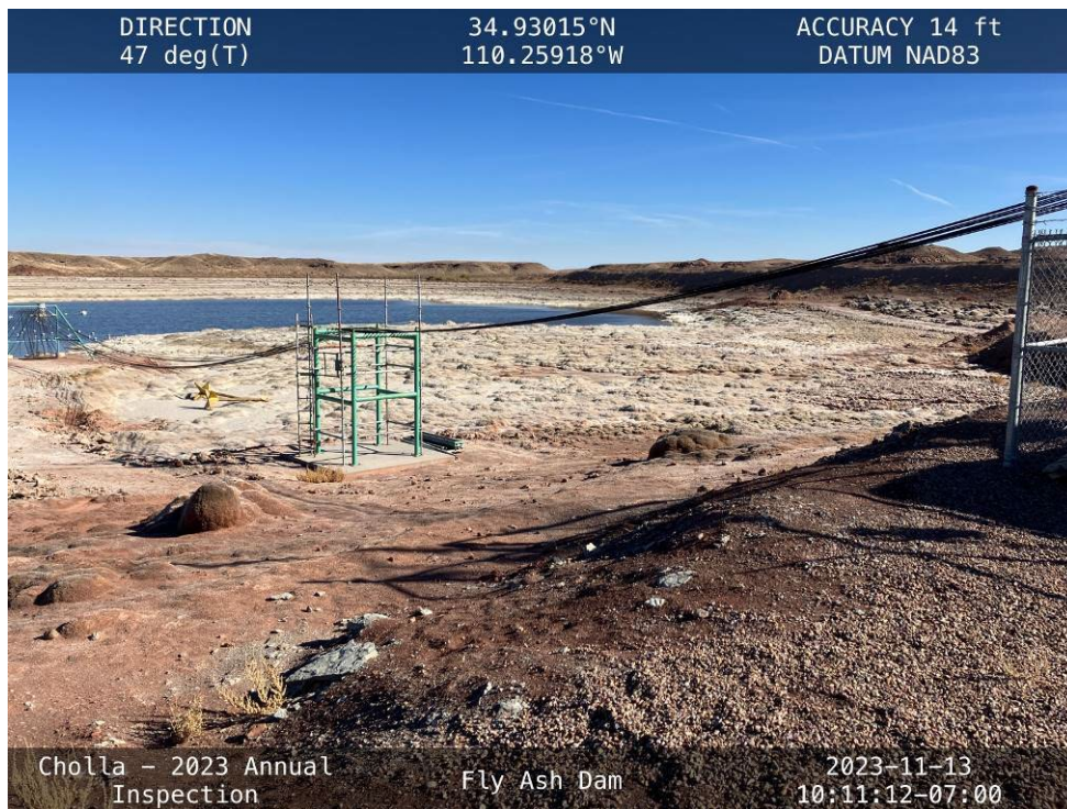
20231113 – IMG_1366 Downdraft evaporators in the Fly Ash Pond. One evaporator being removed for repairs.
