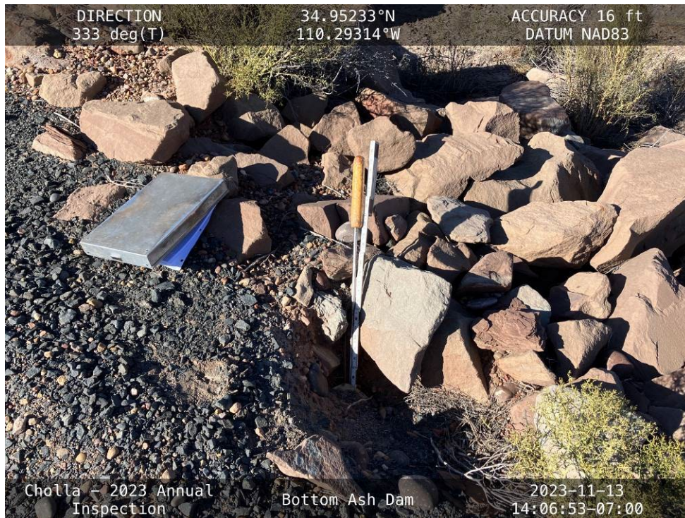
20231113 – IMG_1611 12 inches of erosion on the upstream side of the South Embankment shoulder.
