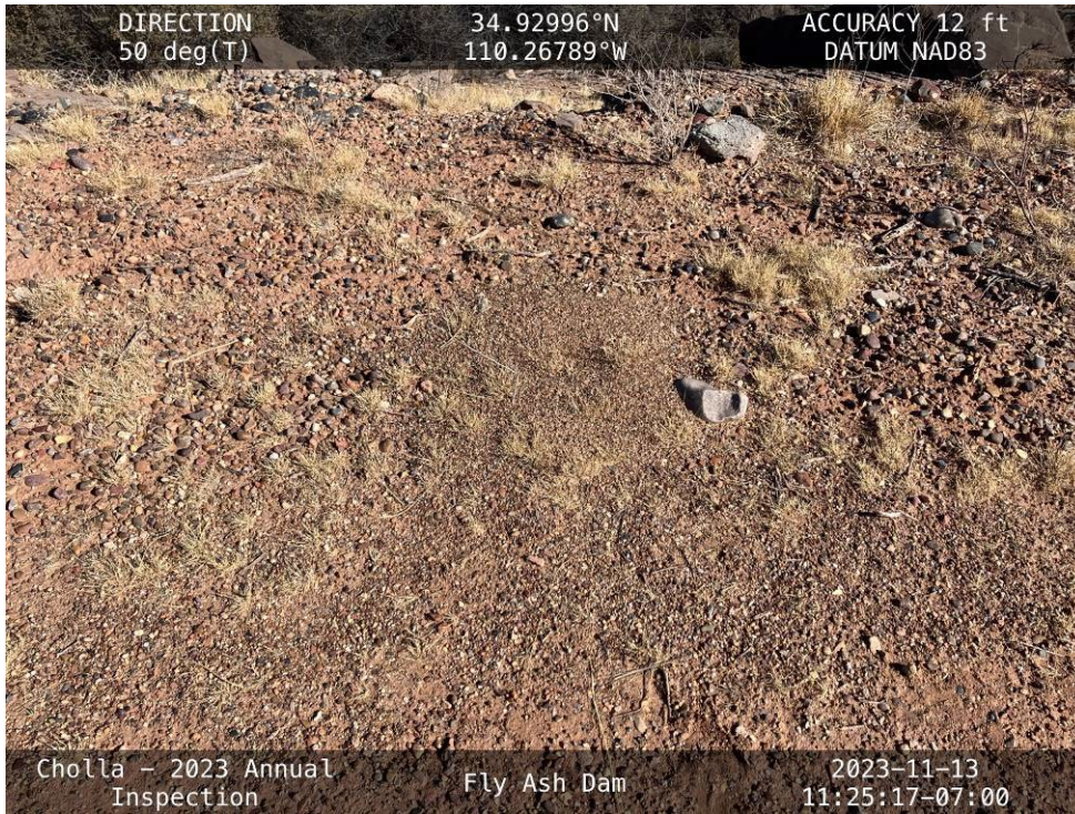
20231113 – IMG_1443 An ant hill on the West Embankment crest.
