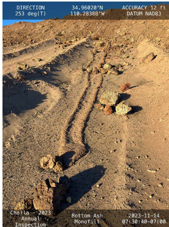
20231114 – IMG_1862 A streak of cemented ash along the downstream slope of the East Embankment.
