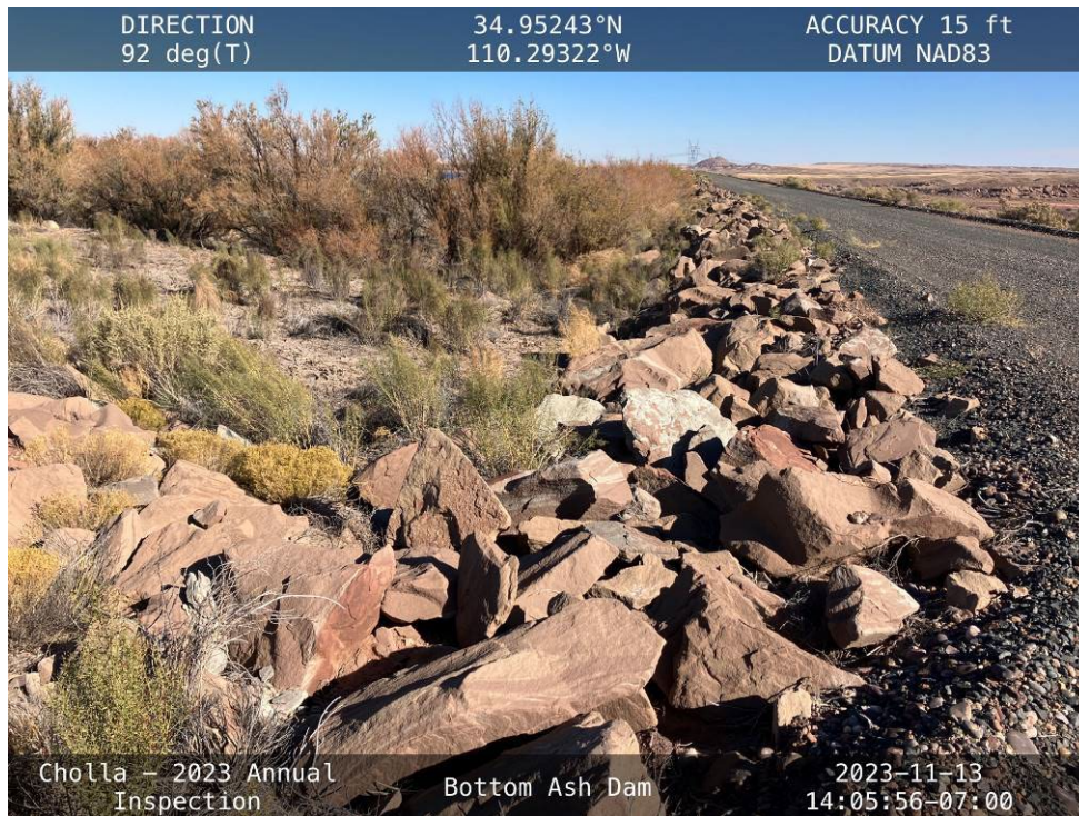
20231113 – IMG_1609 Trees and other woody vegetation to be removed from the South Embankment upstream slope.
