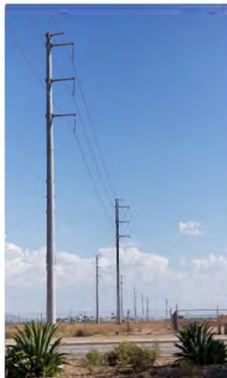
230kV Single Circuit
