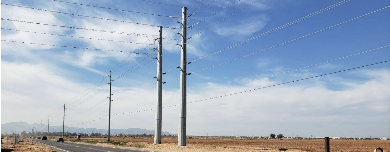
69kV Transmission Line
