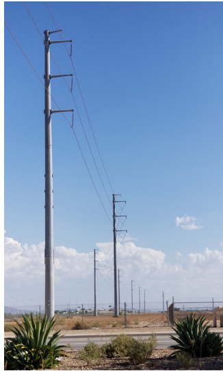
230kV Single Circuit
