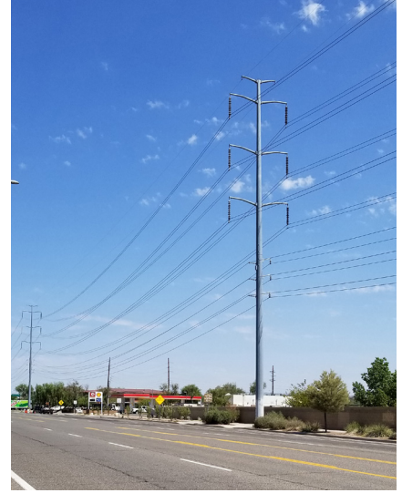
230kV Double Circuit with 69kV Double Circuit Underbuild
