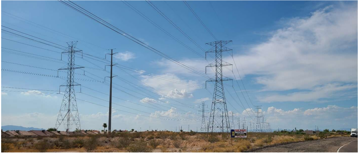
230/345kV Transmission Line Corridor
