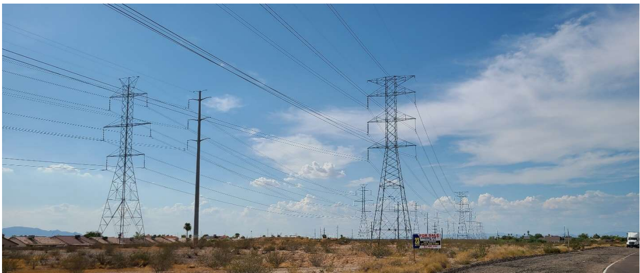
230/345kV Transmission Line Corridor
