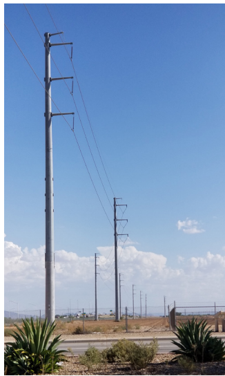
230kV Single Circuit
