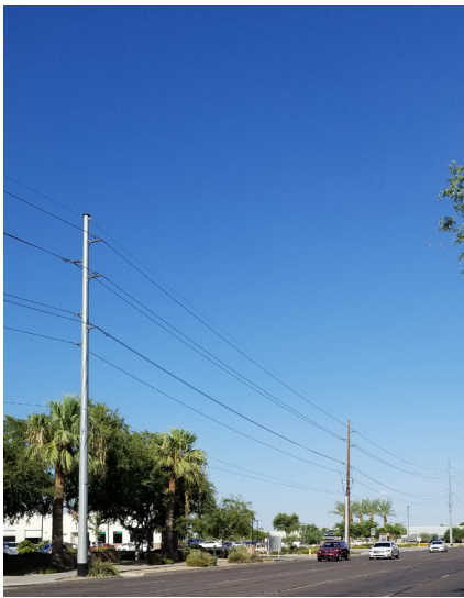
69kV Single Circuit (example of 230kV rebuild opportunity)
