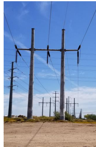
230kV single-circuit H-frame (crossing existing power lines)
