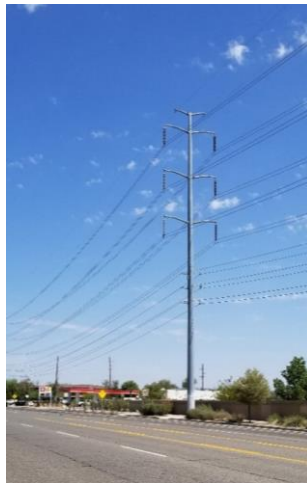
230kV double-circuit monopole with double-circuit 69kV under build
