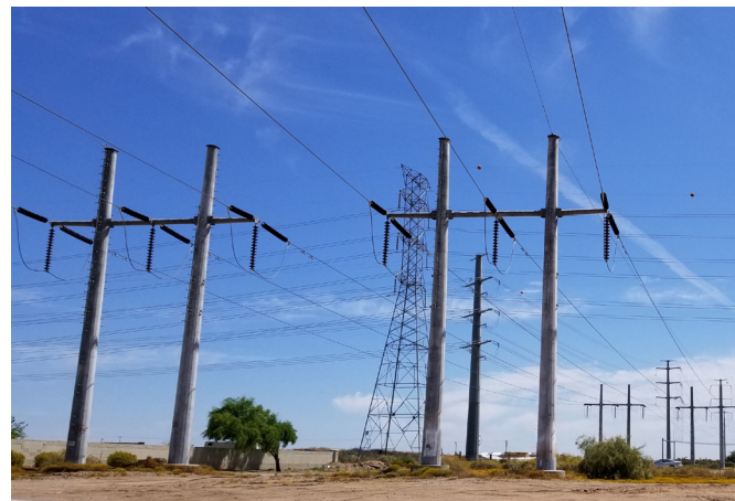
Typical double-circuit 230kV H-Frame structures
