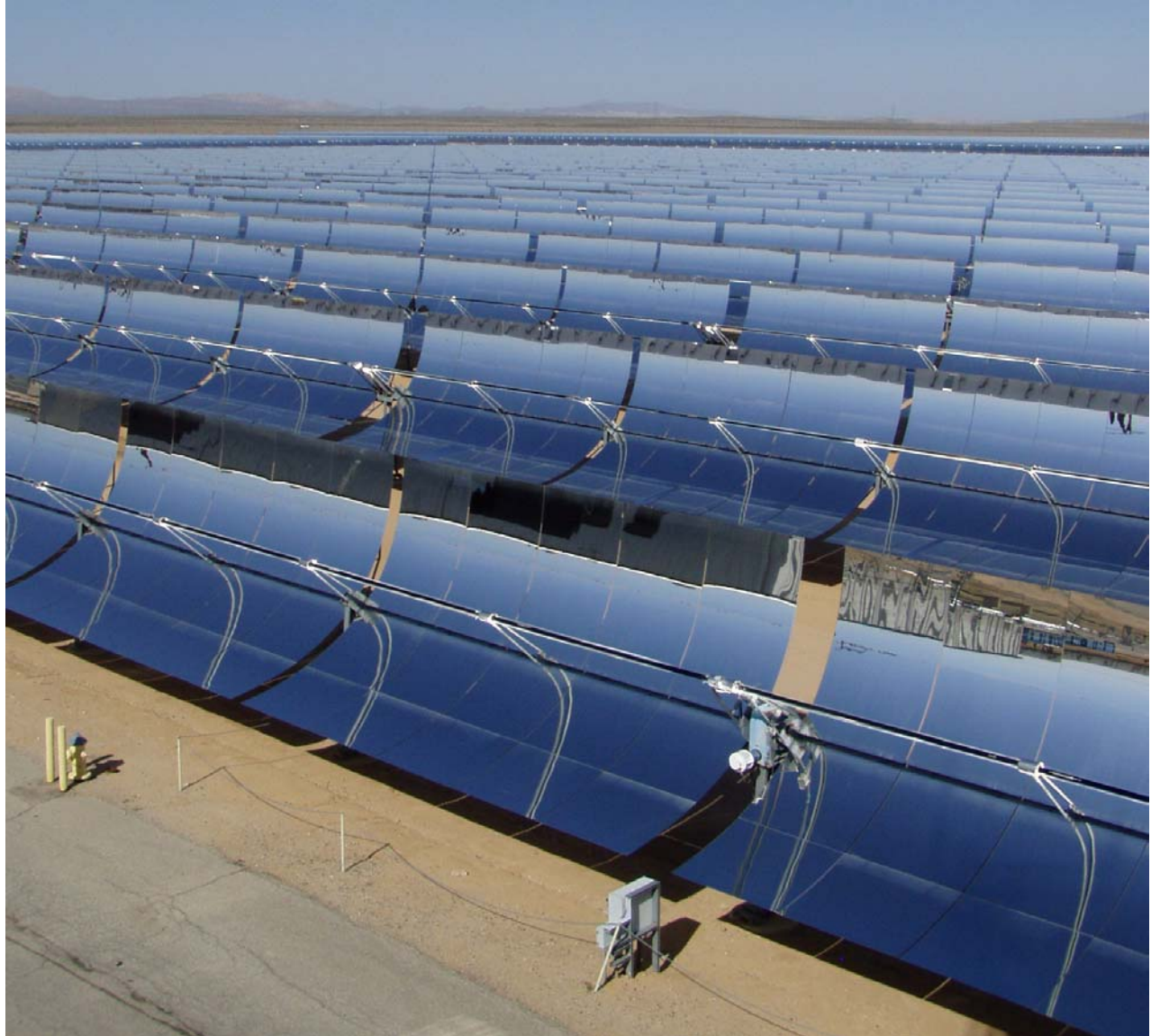
Northern view of the new solar trough plant near APS' Saguaro Power Plant.
