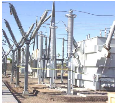
3-NXVCTs Installed at Deer Valley Substation
