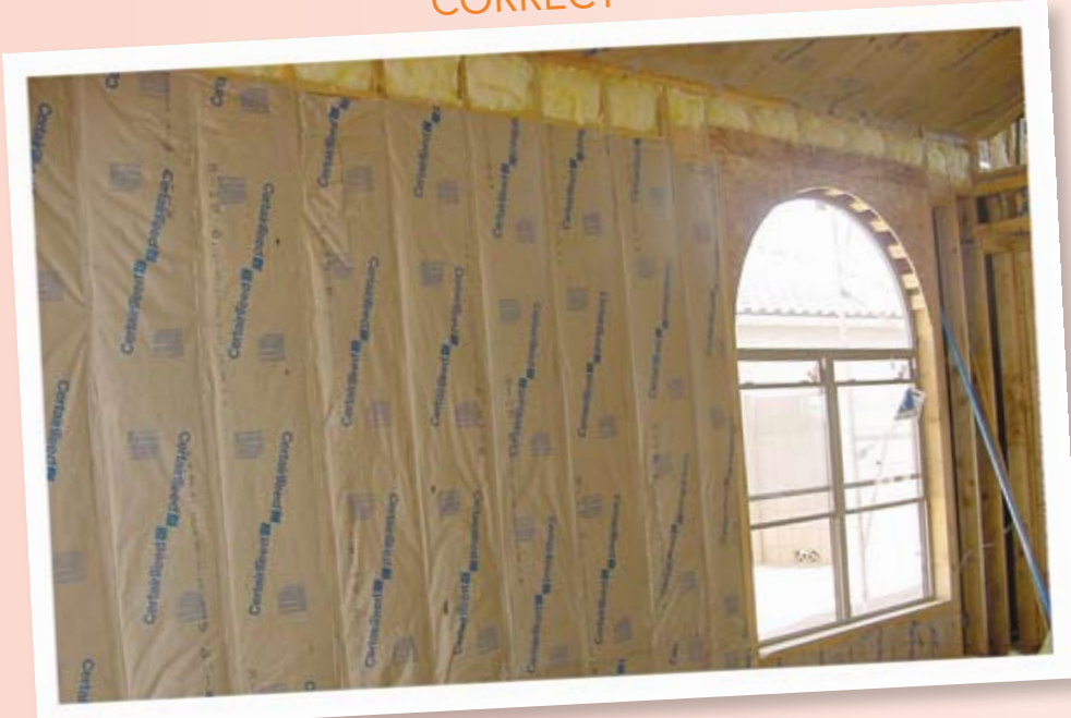
This batt insulation in an ENERGY STAR home does not have gaps, voids or compressions, and comes in to full contact with the air barrier
