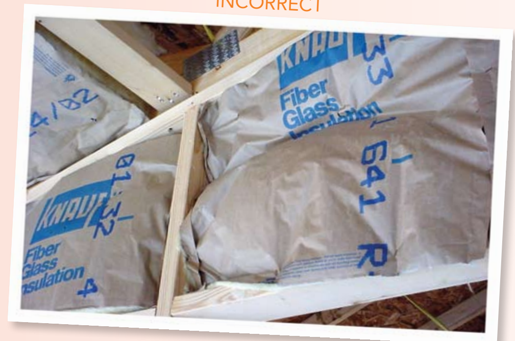
This batt insulation in a standard construction home shows gaps and compressions, which allows air to enter or escape the home
