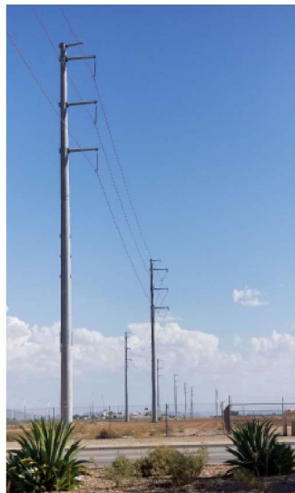
230kV Single Circuit
