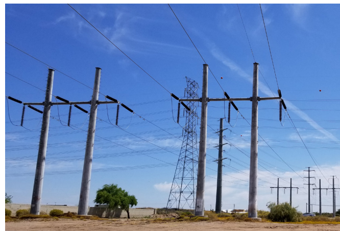
Typical double-circuit 230kV H-Frame structures
