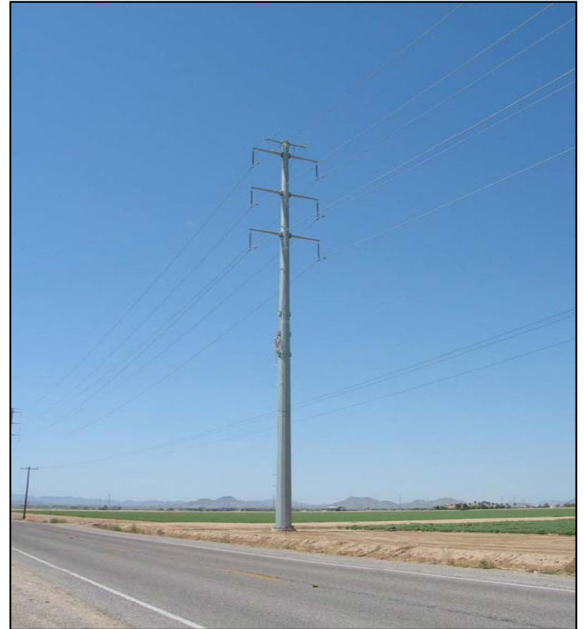
Typical Double-Circuit 230kV Transmission Structure with no 69kV Underbuild
