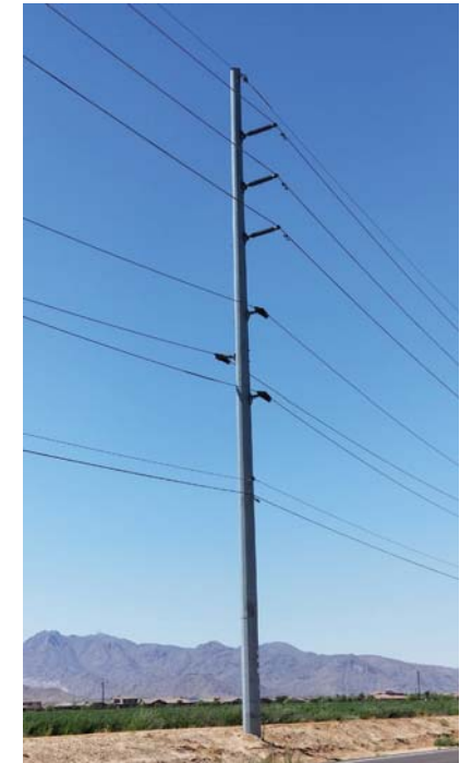
Single-circuit 69kV pole with 12kV underbuild
